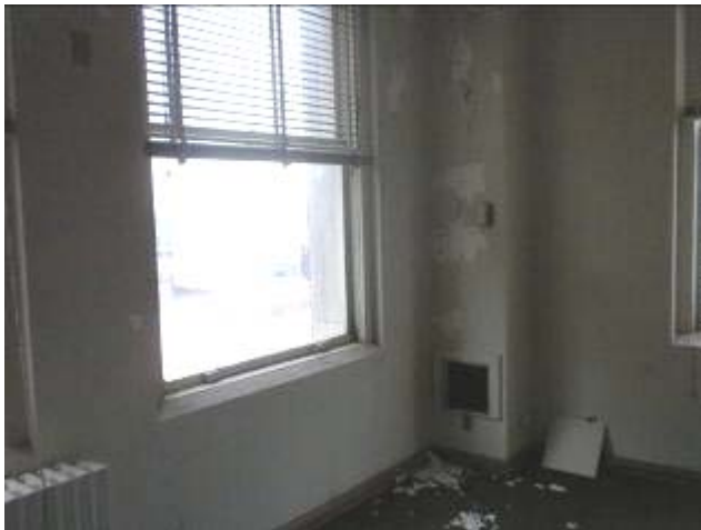
Wall Damage & Cracked Window
