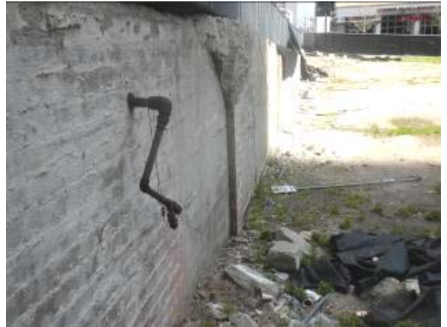
Deteriorating Retaining Wall/Foundation
