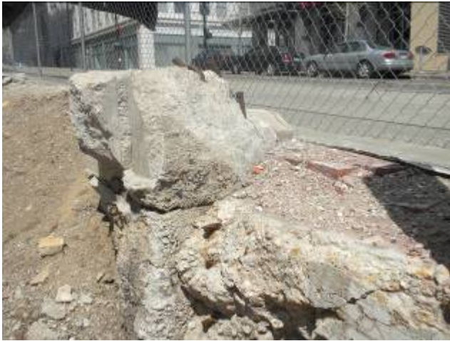
Deteriorating Retaining Wall
