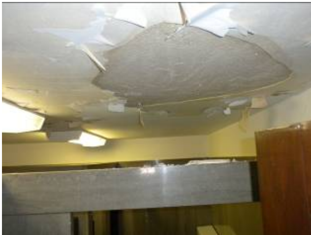
Damaged Office Ceiling Structure
