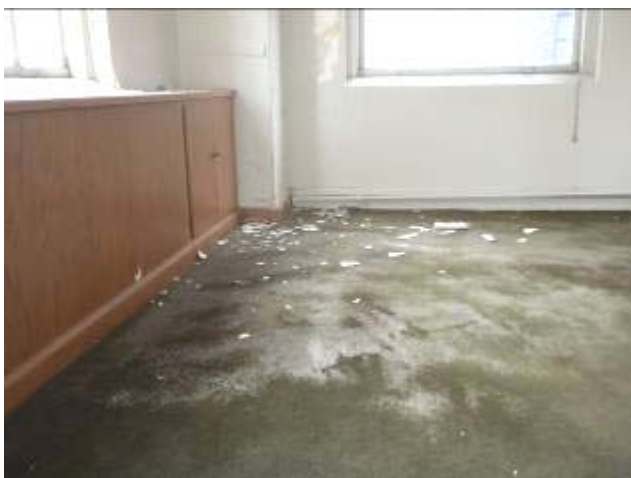
Office Wall & Floor Damage
