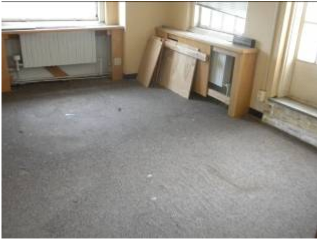
Damaged Office Finish
