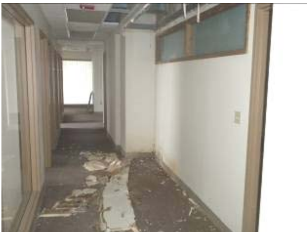
Office Ceiling Damage
