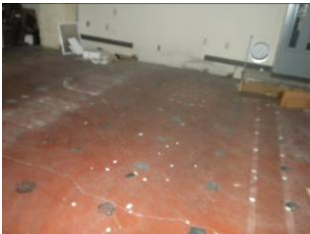
Damaged Office Finish
