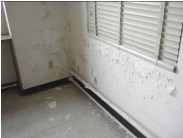
Damaged Office Wall
