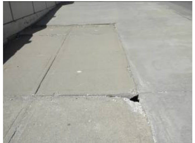
Another View Collapsing Sidewalk Along Baltimore
