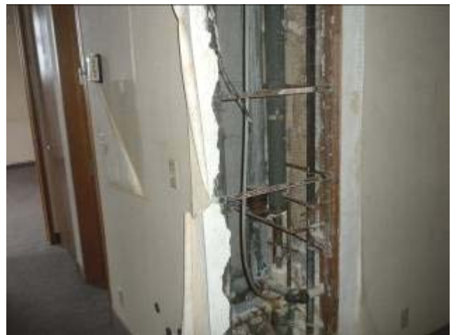
Damaged Office Wall
