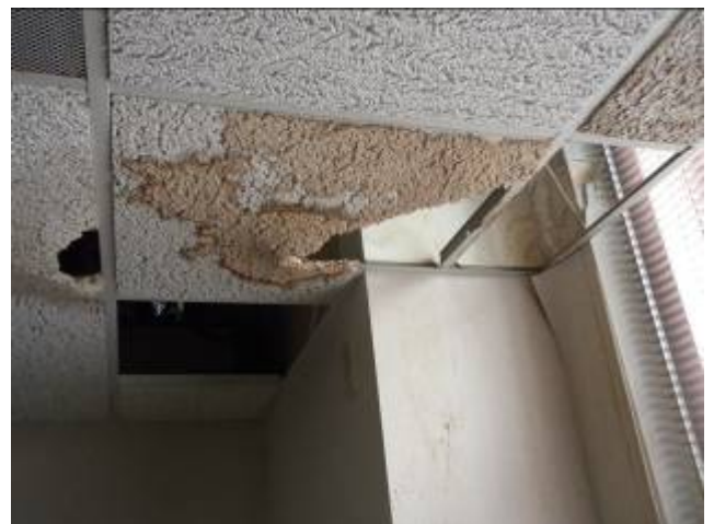
Damaged Office Ceiling
