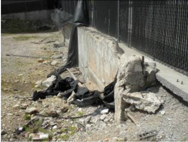
Deteriorating Retaining Wall/Foundation
