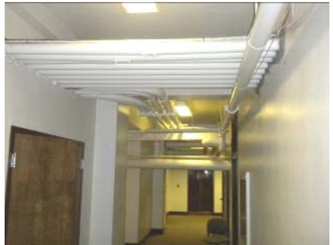
Very Low Pipes In Upper Floor Office Space
