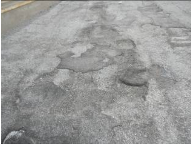
Deteriorating Asphalt In The South Alley
