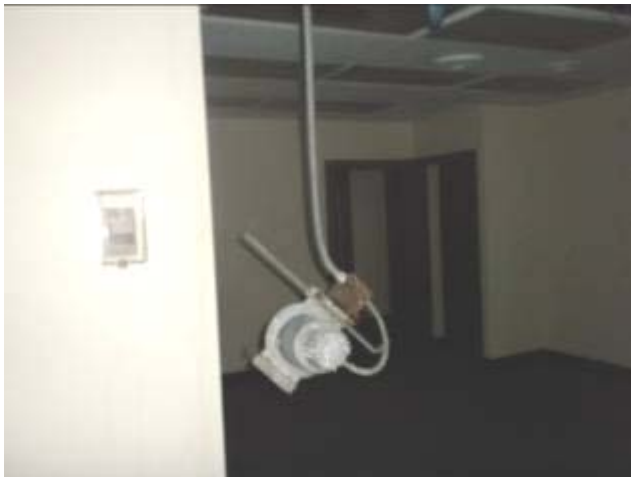
Collapsed Incandescent Light Fixture
