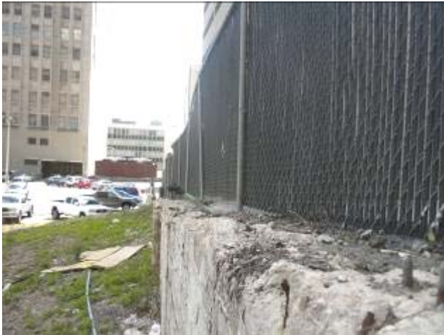
Deteriorating Retaining Wall/Foundation
