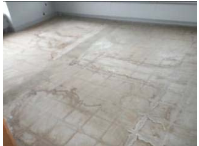
Damaged Office Flooring
