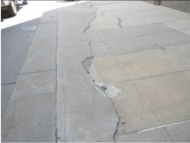
Sidewalk Damage Along Baltimore Avenue
