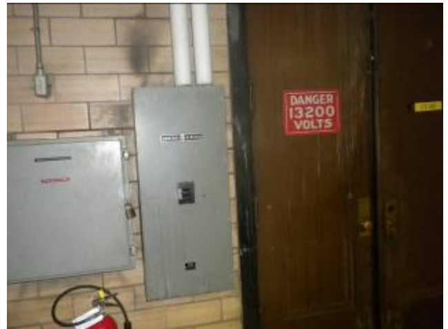
Neighborhood Substation In Sub-Basement
