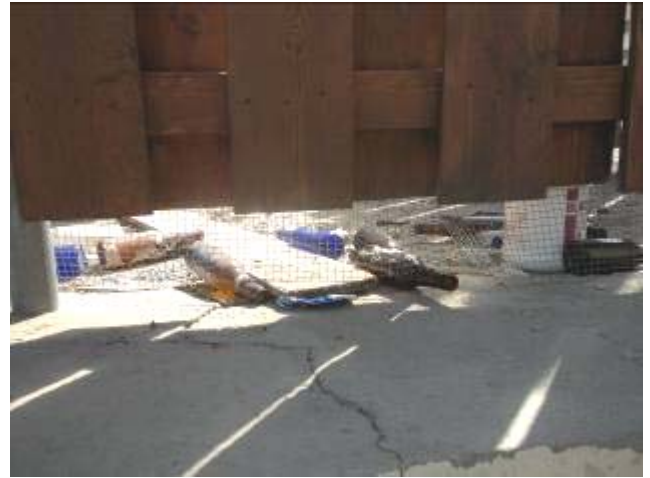
←← Vagrancy At Ground Level Cooling Towers
