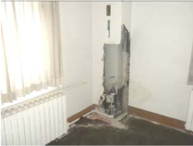
Office Wall Damage
