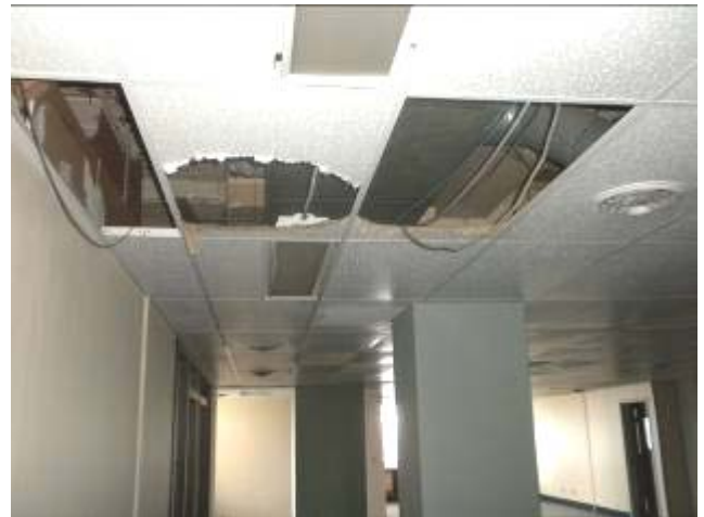
Damaged Office Ceiling
