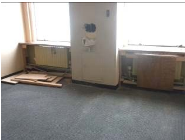
Damaged Office Finish
