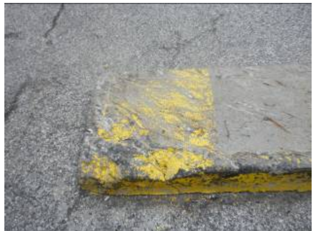
Deteriorating Concrete Island
