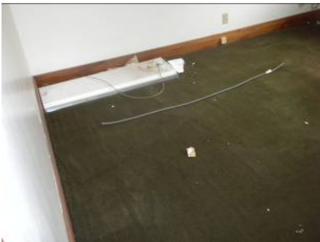
Collapsed Fluorescent Light Fixture In Office
