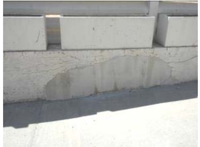
Deteriorating Wall Fronting Baltimore Avenue
