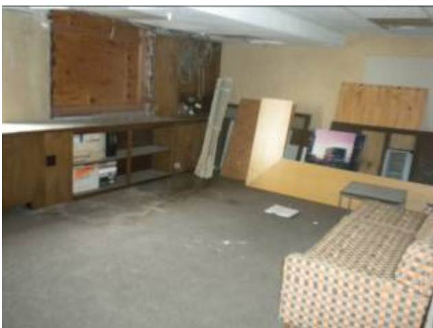
Dated & Deteriorating Office Finish
