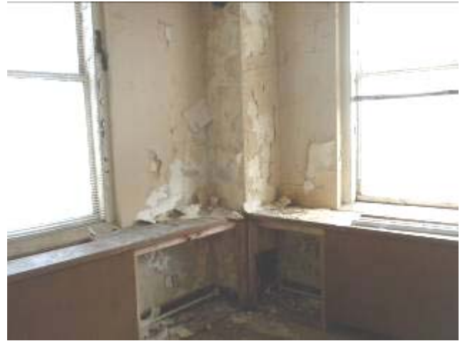
Office Wall Damage
