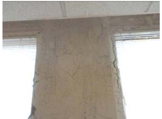
Office Wall Damage
