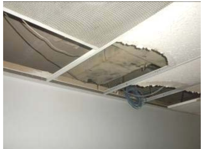
Office Ceiling Damage
