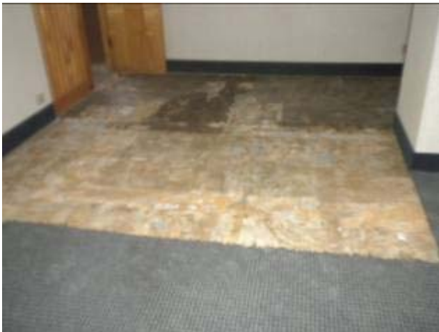
Damaged Office Flooring
