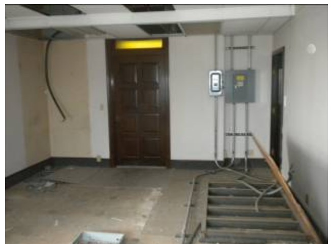
Poor/Deteriorating Office Finish
