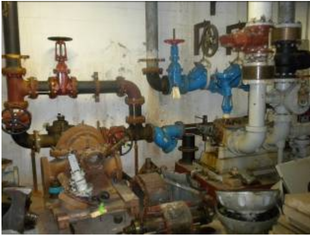
Non-Functioning Fire Standpipe System
