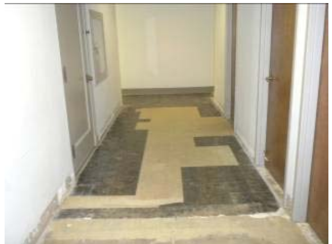
Damaged Flooring In Office Space
