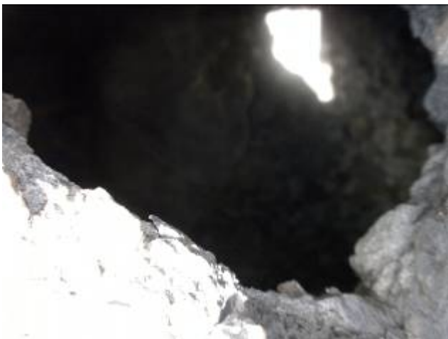
Another View Collapsing Sidewalk Along Baltimore
