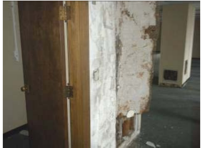
Damaged Office Wall
