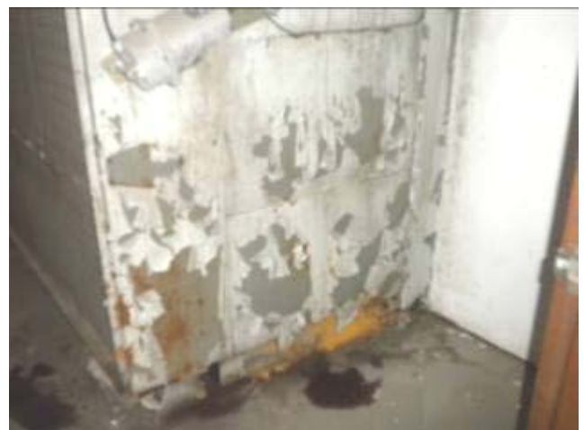
Peeling Paint (LB?) On Office Floor Air Handler
