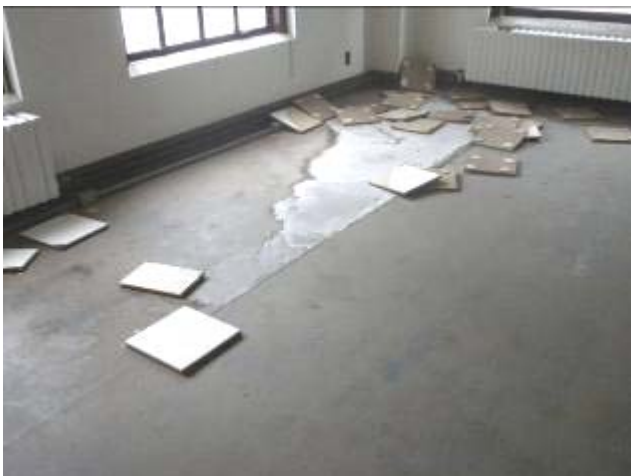
Collapsing Ceiling Tiles & Floor Damage
