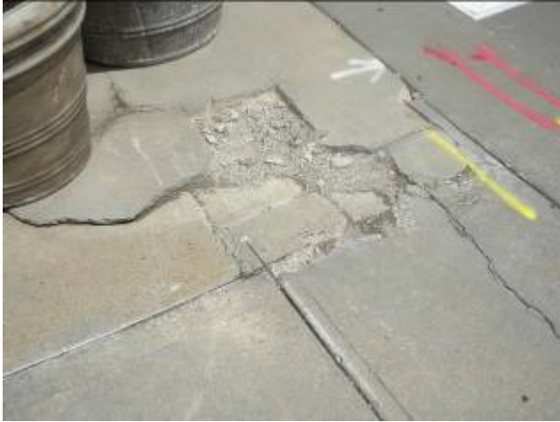
Sidewalk Damage Along W 14 th Street
