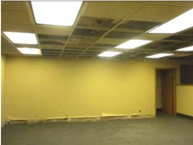
Damaged Office Finish
