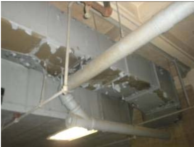
Peeling Paint (Lead-Based?)
