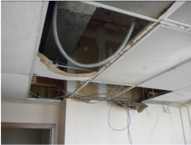
Ceiling & Wiring Damage
