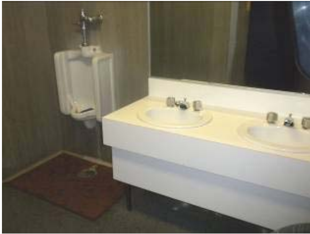
Poor Restroom Design
