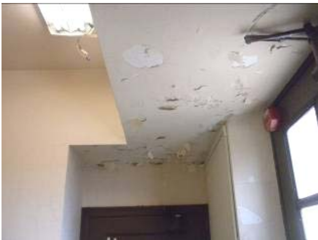
Damaged Office Ceiling
