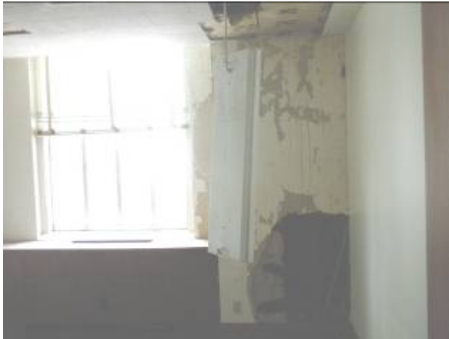
Office Wall Damage
