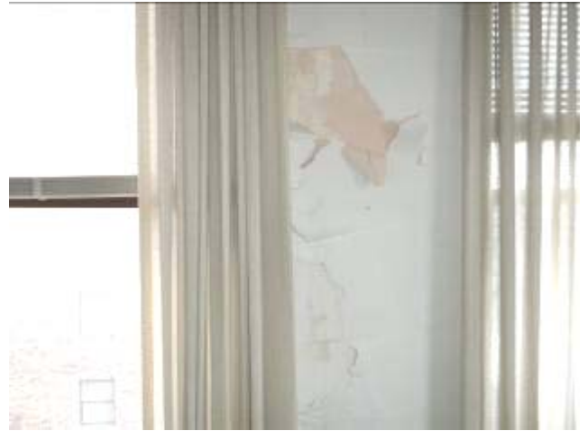
Office Wall Damage
