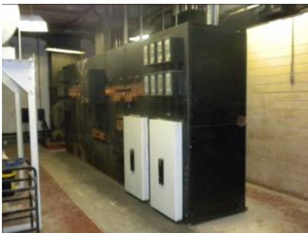
Dated Building Electrical Panels
