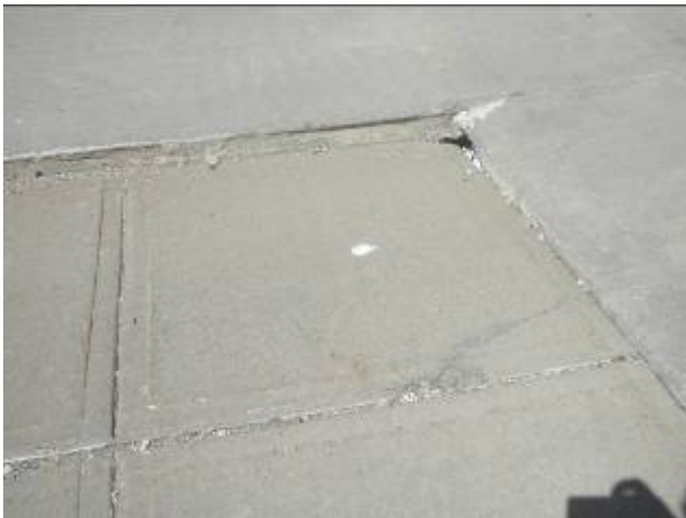
Collapsing Sidewalk Along Baltimore Avenue
