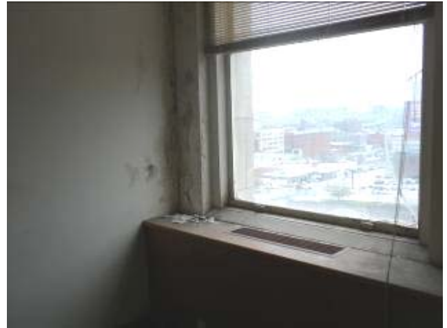
Wall Damage & Cracked Window
