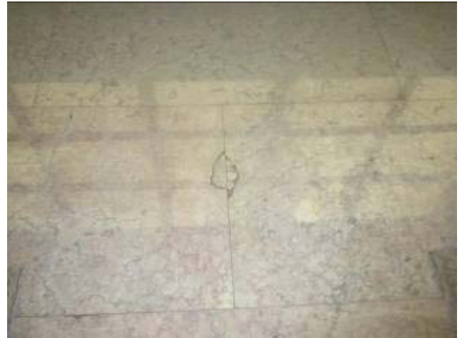
Cracked Marble Wall Panel
