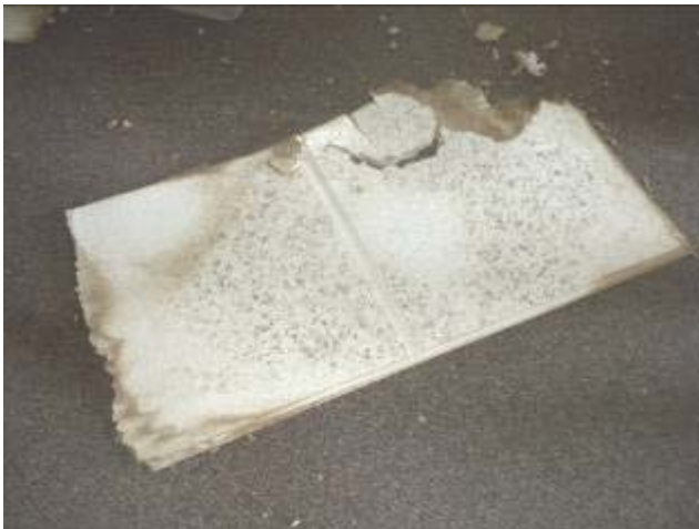
Ceiling Damage & Black Mold
