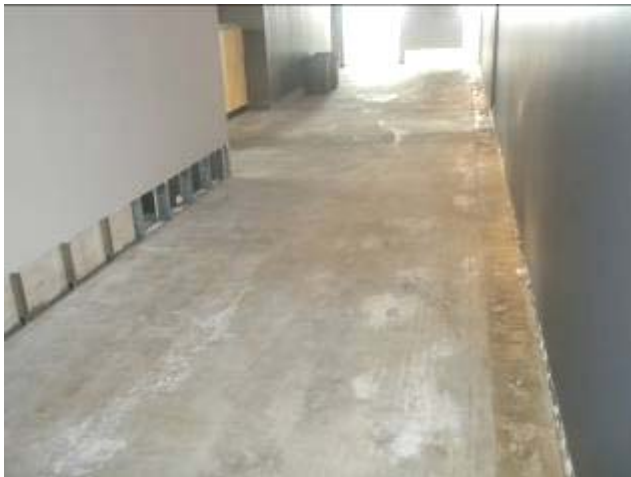
Poor Office Finish
