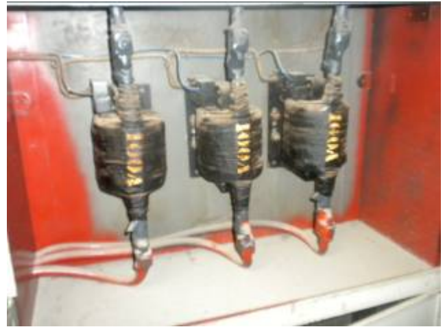
Dated Electrical Distribution
