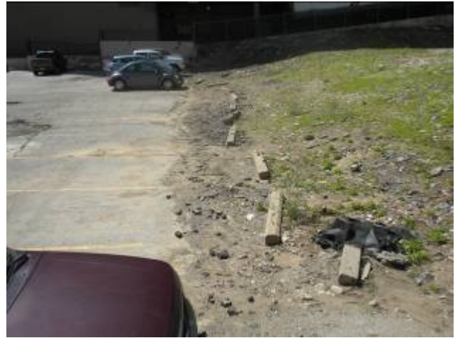
Misplaced Parking Blocks
