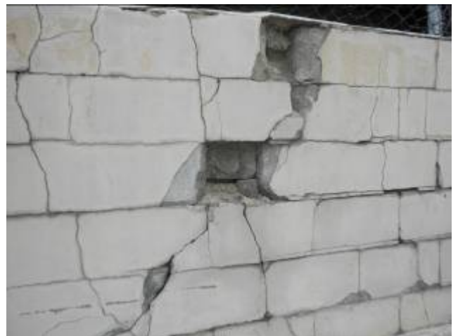
Deteriorating Retaining Wall
