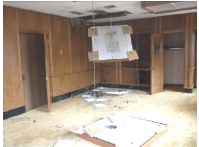
Collapsed 4'x4' Light Fixtures
