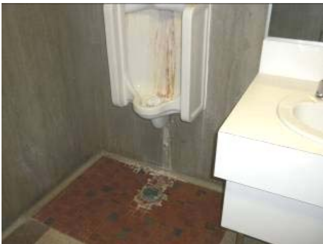
Deteriorating Plumbing Fixtures
