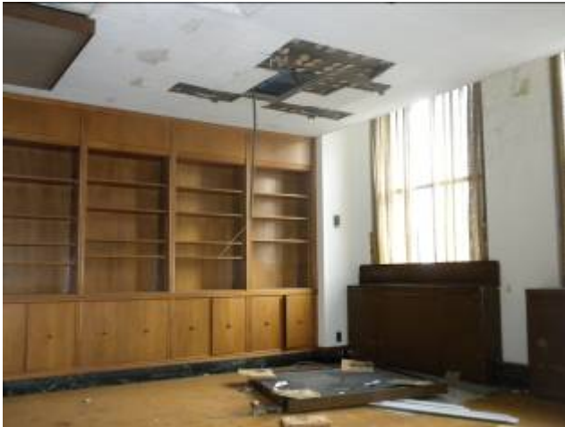
Collapsed 4'x4' Light Fixture
