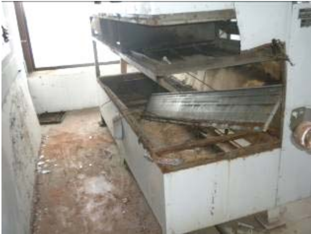
Damaged Air Handling Unit On Upper Floor Office
