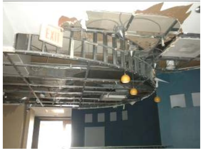
Damaged Office Ceiling Structure
