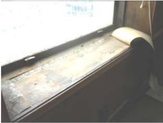
Deteriorated Steam Radiator Cabinet
