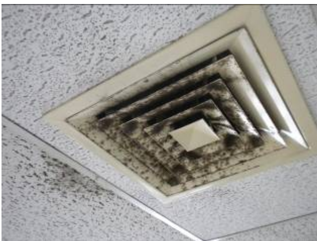
Mold On Office Air Vent
