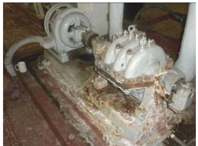
Rusted Mechanical Equipment
