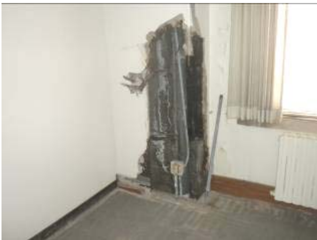
Office Wall Damage
