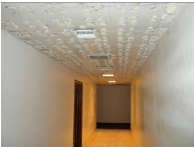
Damaged Hallway Ceiling
