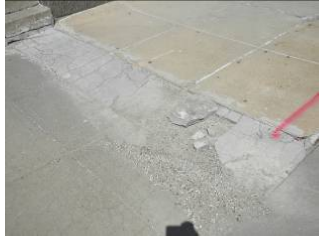
Sidewalk Damage Along W 14 th Street
