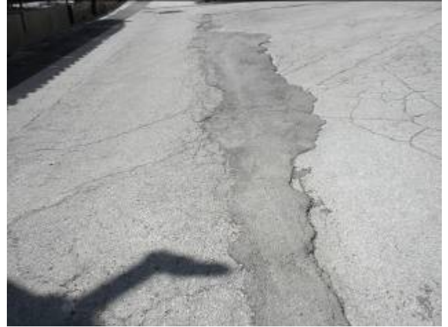
Deteriorating Asphalt In The West Alley
