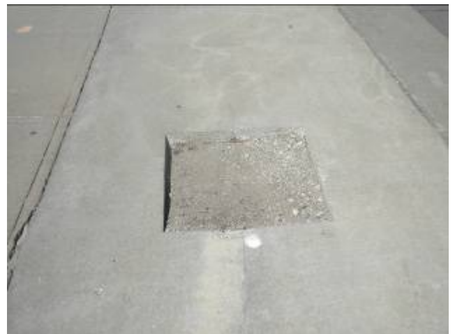
Sidewalk Damage Along Baltimore Avenue
