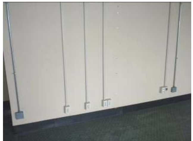
Dysfunctional Electrical Distribution
