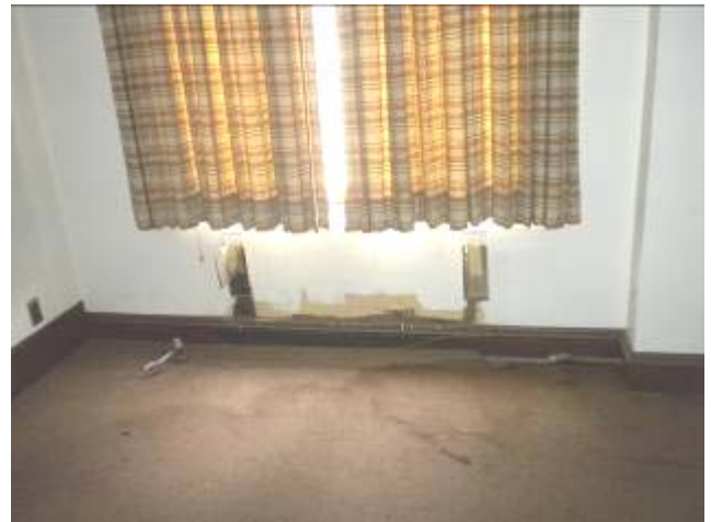
Dated Curtains & Wall & Floor Damage
