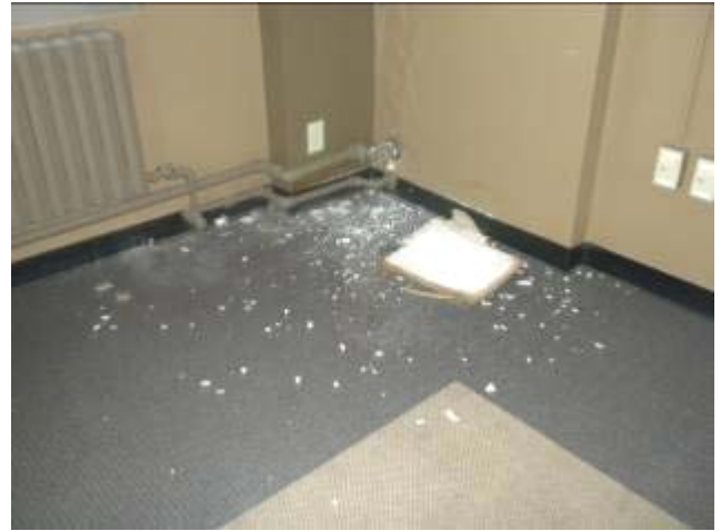
Office Ceiling/Wall/Floor Damage
