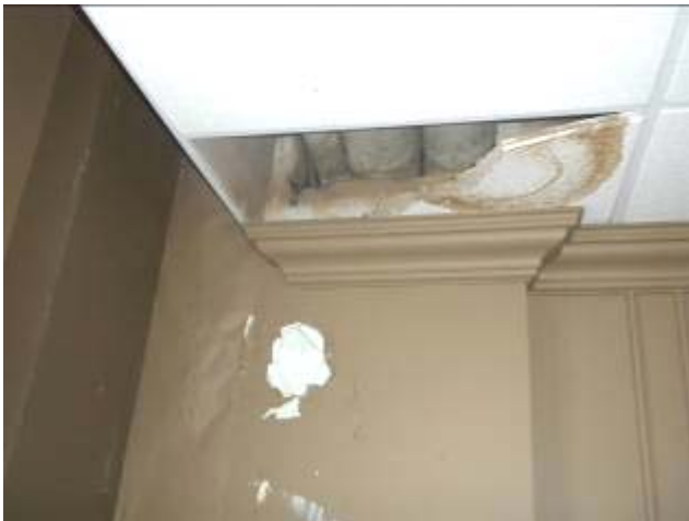
Office Ceiling & Wall Damage
