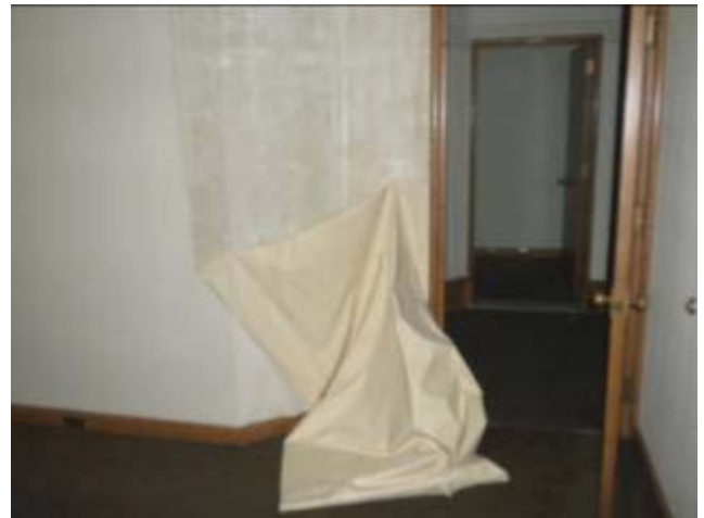
Delaminated Vinyl Wallcovering
