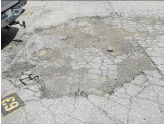
Deteriorating Asphalt Paving
