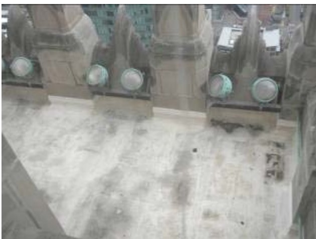
Dated Roof Covering
