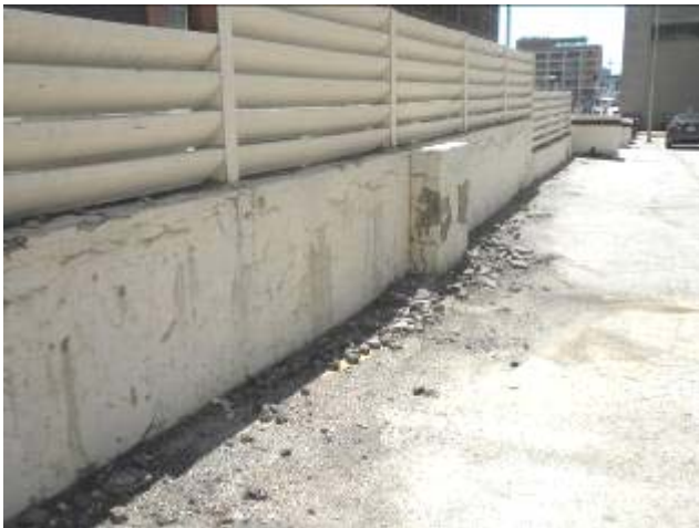
Deteriorating Retaining Wall
