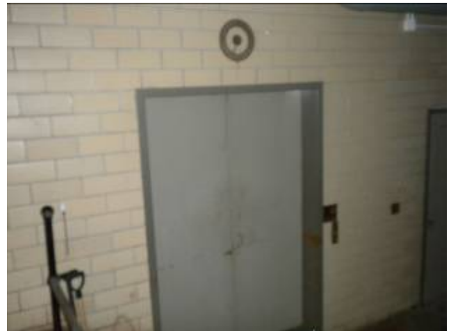
Non-Maintained Freight Elevator
