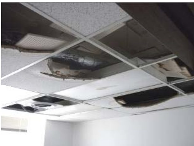
Damaged Office Ceiling
