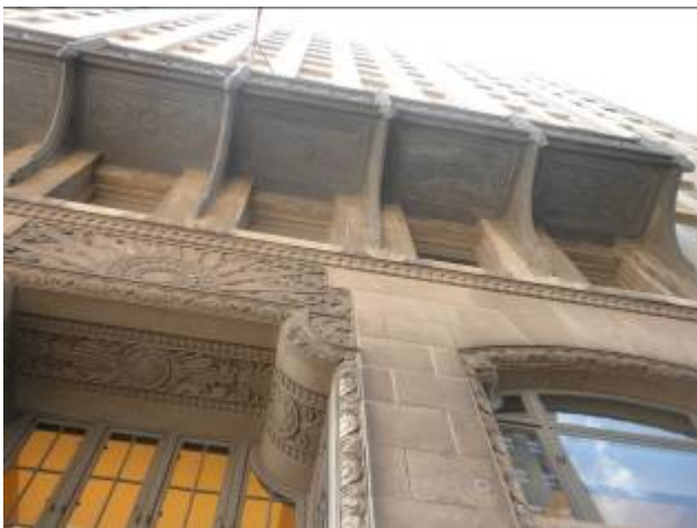
Discolored Deteriorating Exterior
