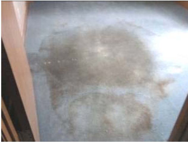
Damaged Office Carpeting
