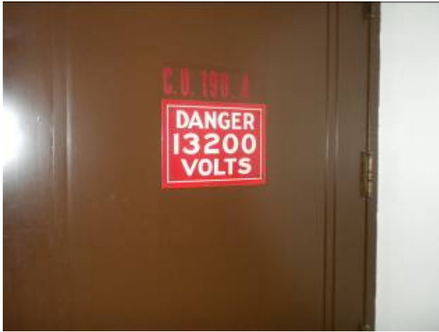
Upper Floor Electrical Closet → →
