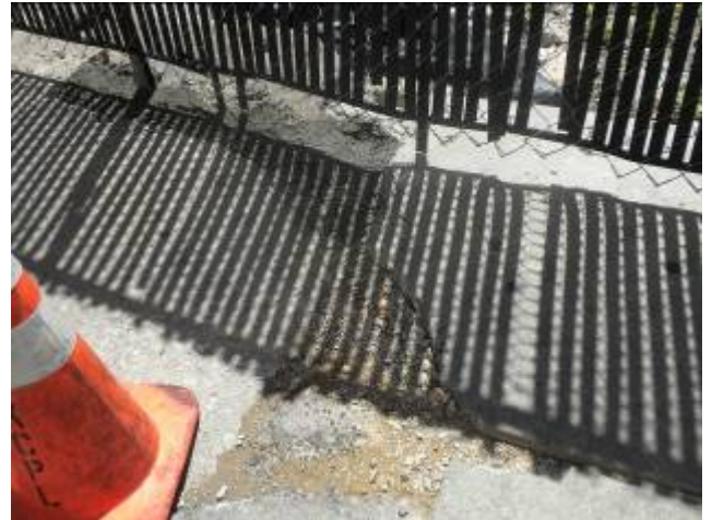
Sidewalk Damage Along W 13 th Street
