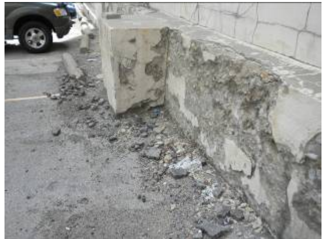
Deteriorating Retaining Wall
