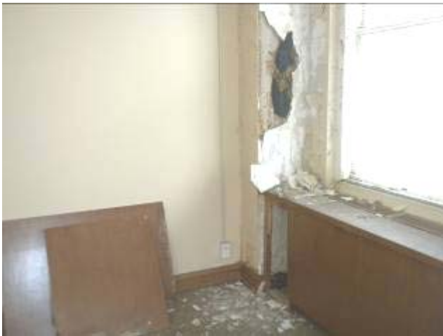
Office Wall Damage
