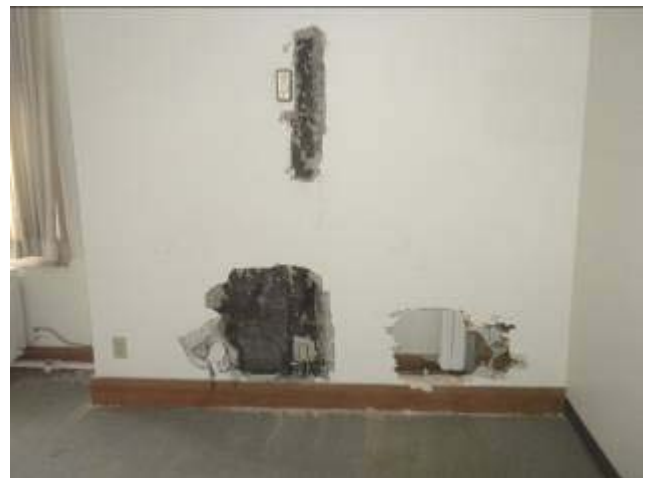
Office Wall Damage
