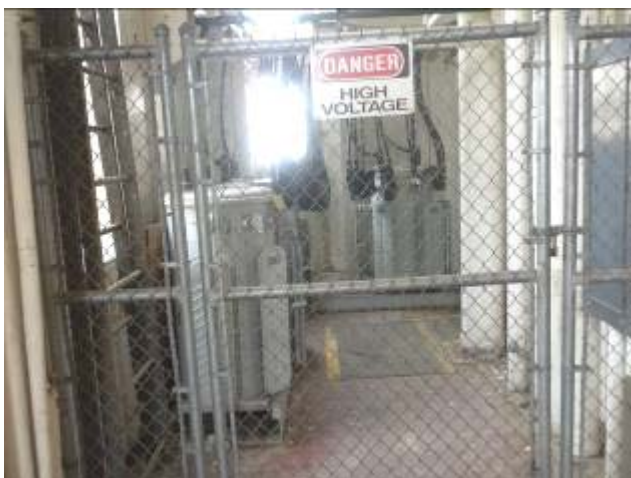
Dated Electrical Distribution On Upper Floor
