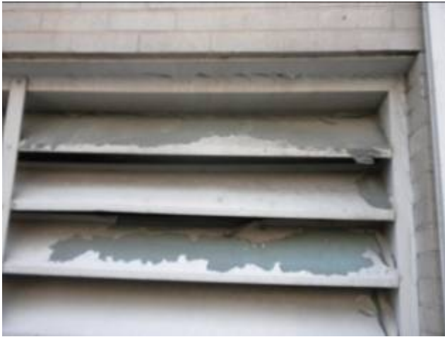
Peeling Paint (Lead-Based?)
