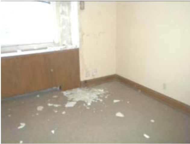
Office Wall Damage
