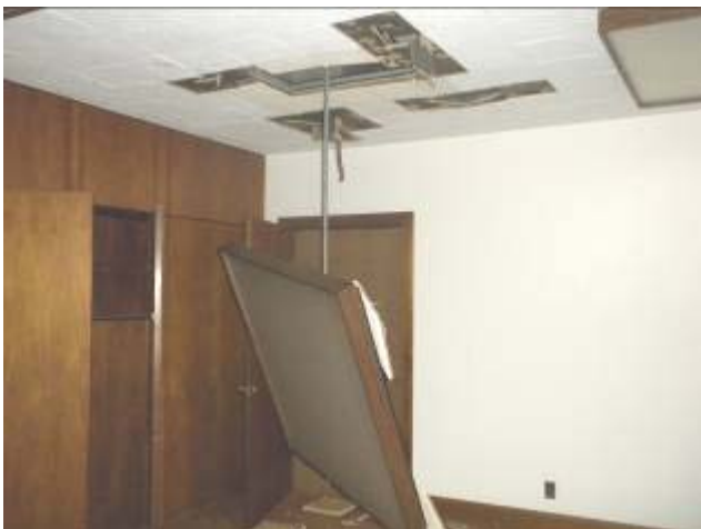
Collapsed 4'x4' Light Fixture
