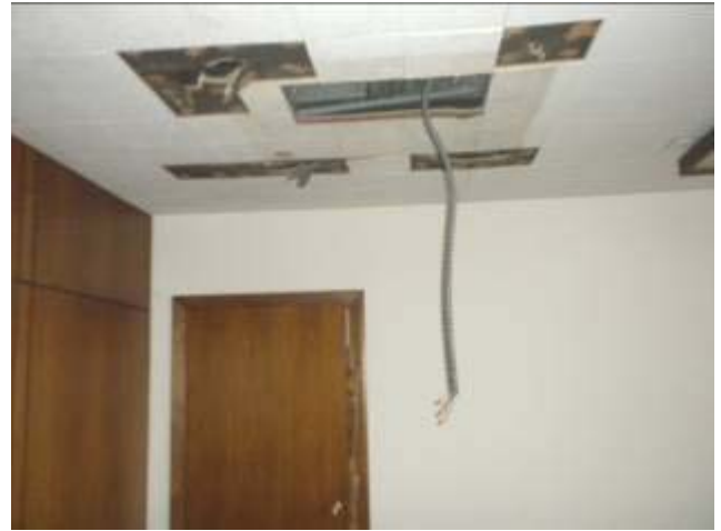
Damaged Office Ceiling & Electrical
