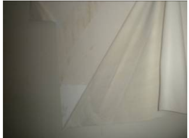
Delaminating Vinyl Wallcovering
