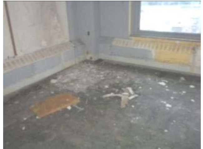
Damaged Office Finish
