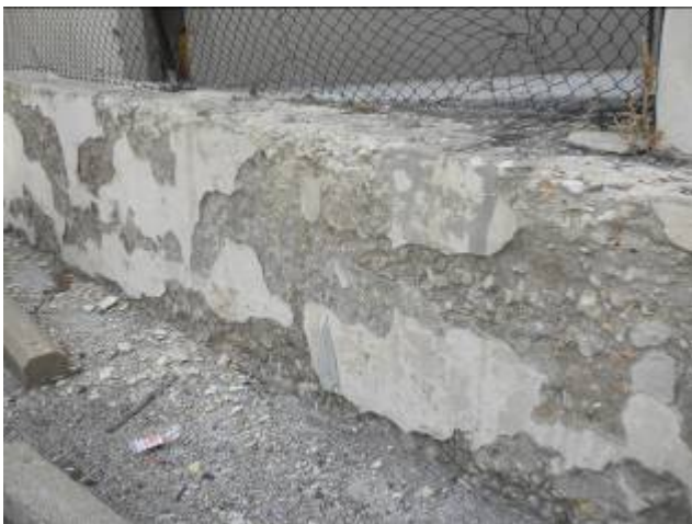
Deteriorating Retaining Wall
