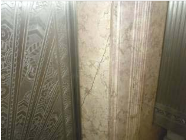
Cracked Marble Wall Panel
