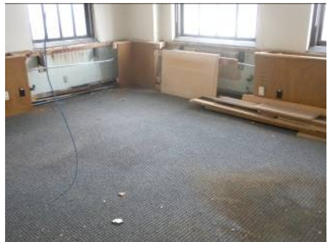
Deteriorated Office Space
