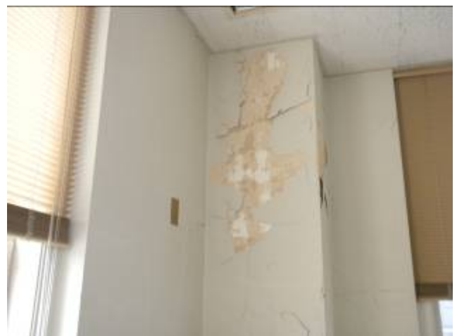
Office Wall Damage
