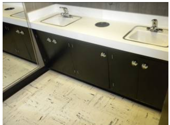
Dated Restroom Finish – Non-ADA Compliant
