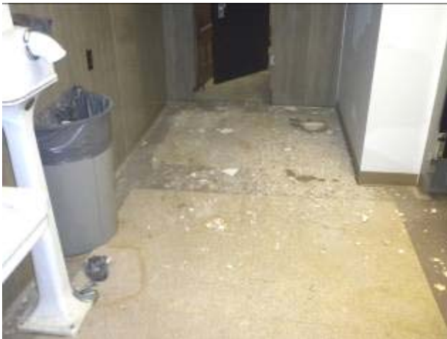
Damage Within Restroom
