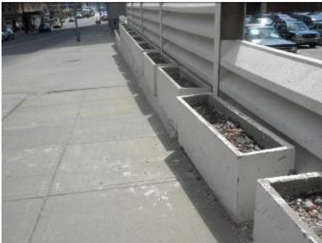
Deteriorating Planters Fronting Baltimore Avenue
