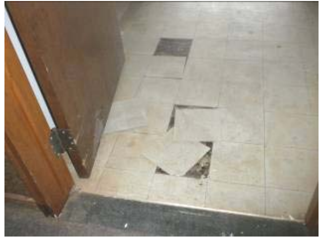
Damaged Office Flooring
