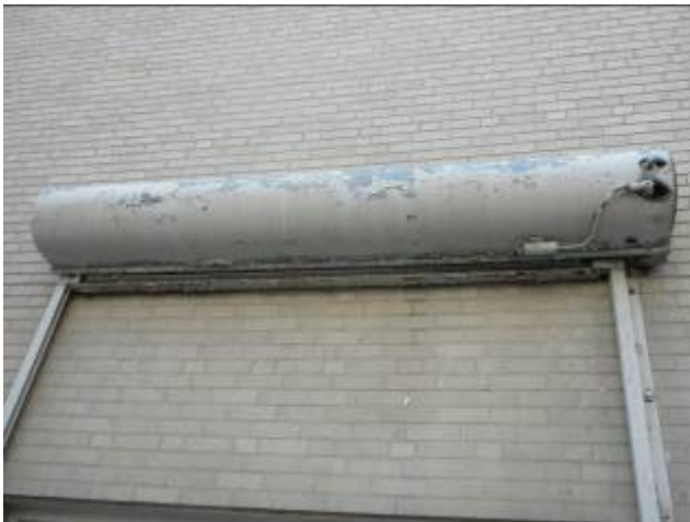
Peeling Paint (Lead-Based?)
