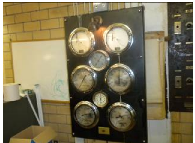
Dated Steam Heat Controls
