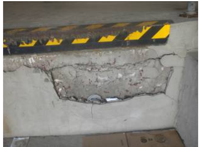
Damaged Dock Area
