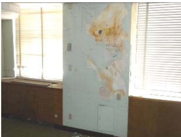
Damaged Office Finish
