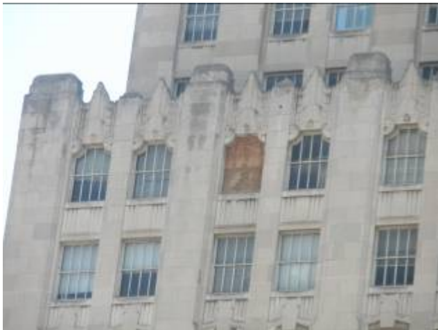
Unightly Discoloration & Broken Window
