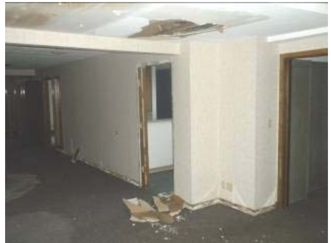
Damaged Office Finish
