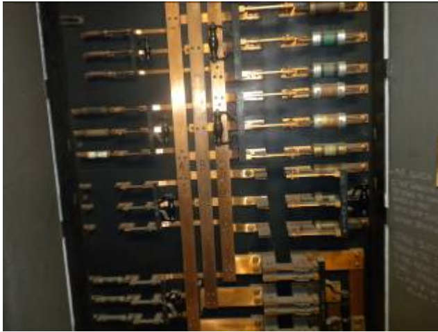
Dated Electrical Distribution
