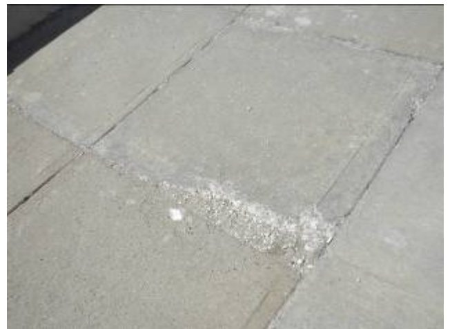
Sidewalk Damage Along Baltimore Avenue
