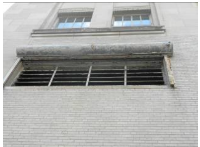
Peeling Paint (Lead-Based?)
