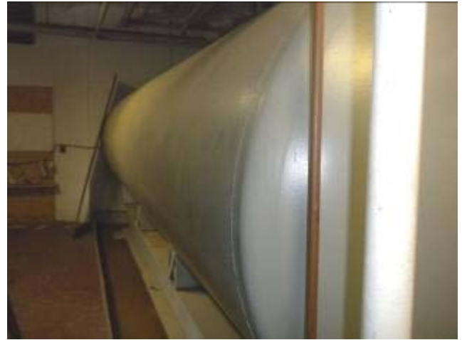
Cooling Water Holding Tank On Upper Floor
