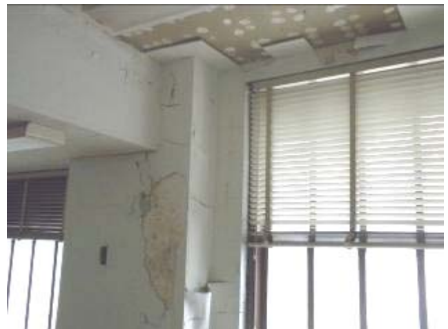
Office Ceiling & Wall Damage
