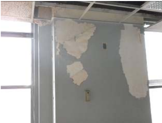
Damaged Office Ceiling & Wall
