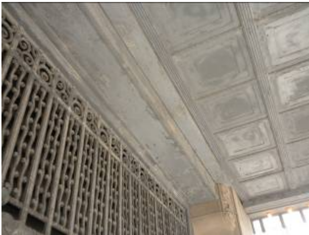
Deteriorating Art Deco Features
