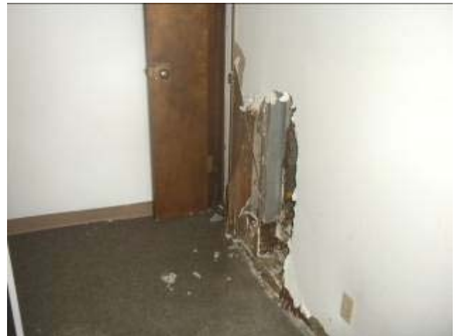
Damaged Office Wall
