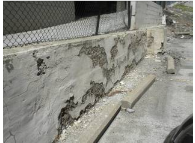
Deteriorating Retaining Wall
