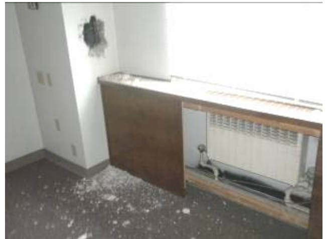
Wall Damage & Dated HVAC
