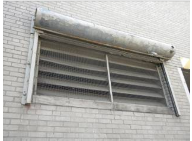
Peeling Paint (Lead-Based?)
