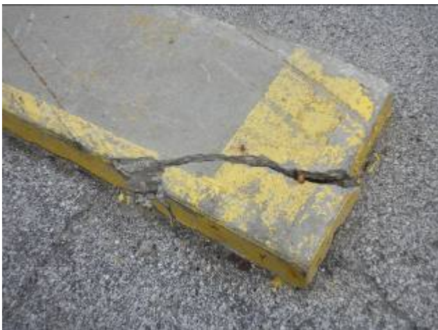
Deteriorating Concrete Island
