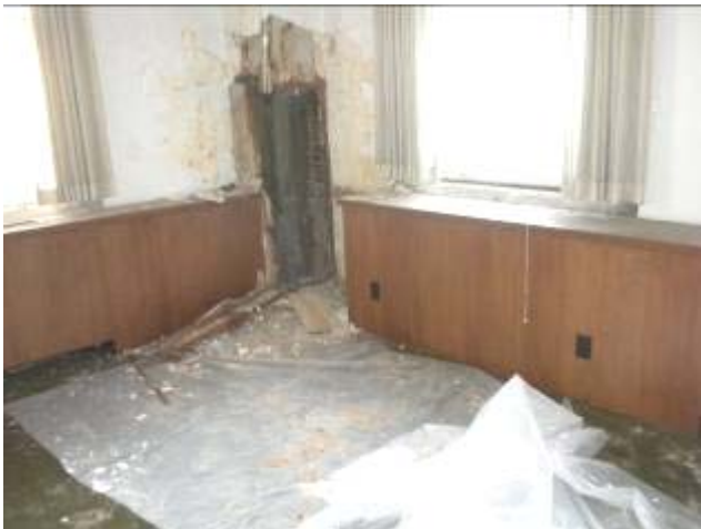
Office Wall Damage
