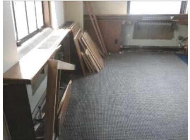
Damaged Office Space
