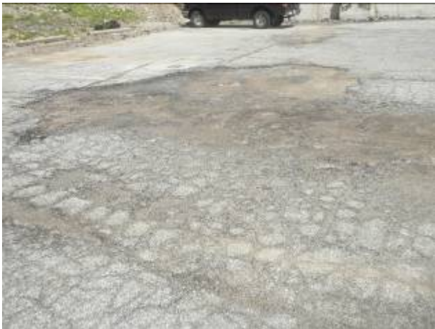
Deteriorating Asphalt Paving
