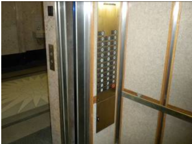
Obsolete, Non-Pressurized Elevators
