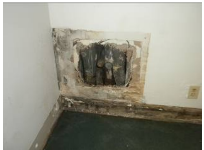
Damaged Office Finish
