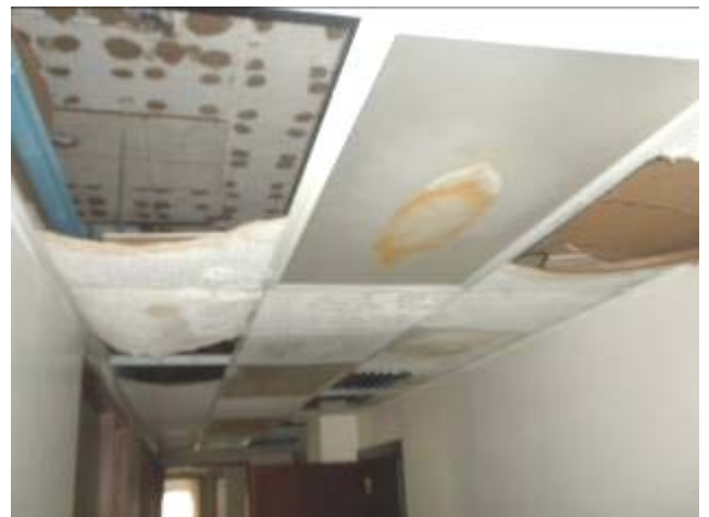
Office Ceiling Damage
