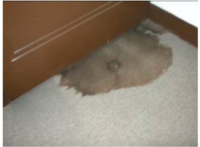
← ←Leakage Beneath Upper Floor Elec. Closet
