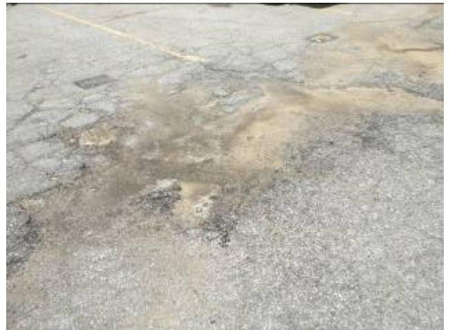
Deteriorating Asphalt Paving
