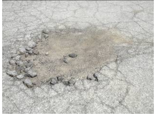
Deteriorating Asphalt Paving
