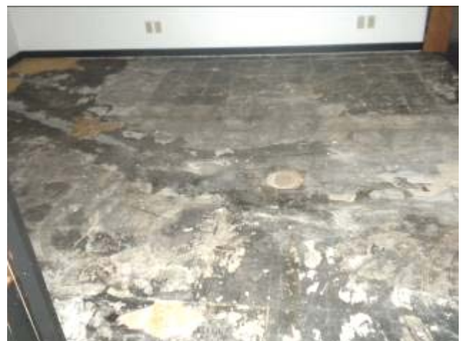
Poor Floor Finish
