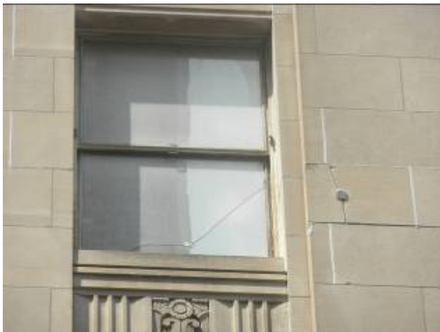
Broken Window & Cracked Limestone Block
