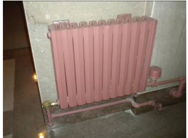
Obsolete Radiator Steam Heat
