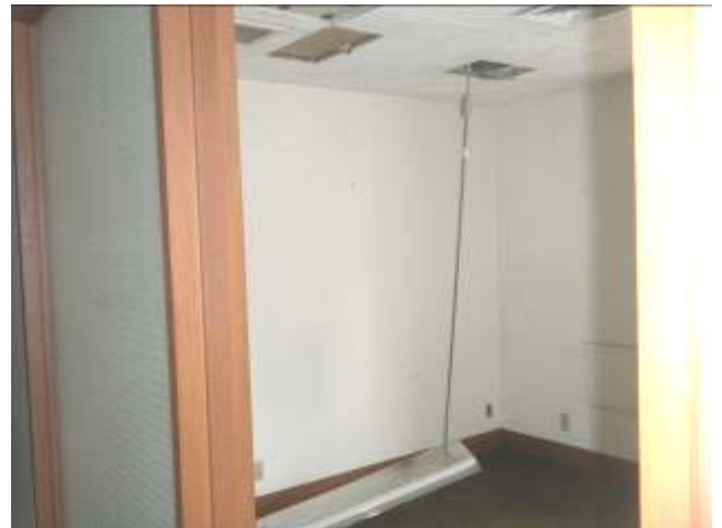
Collapsed Fluorescent Light Fixture In Office
