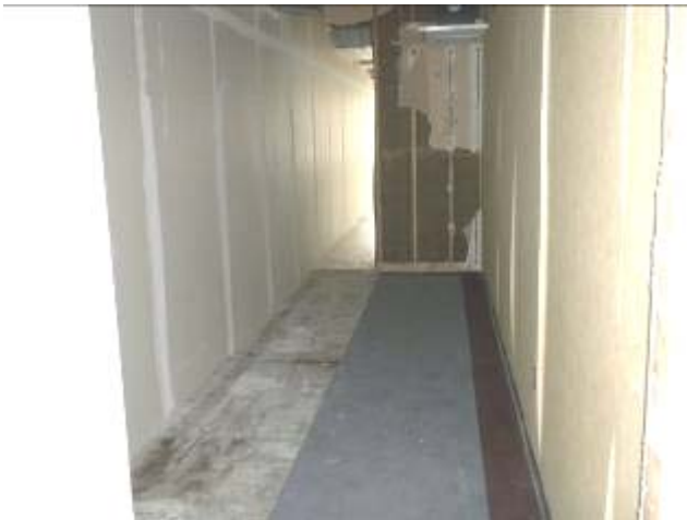
Damaged Office Walls & Floors
