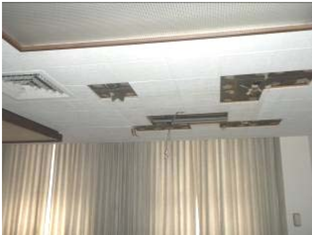
Damaged Office Ceiling & Dated Curtains
