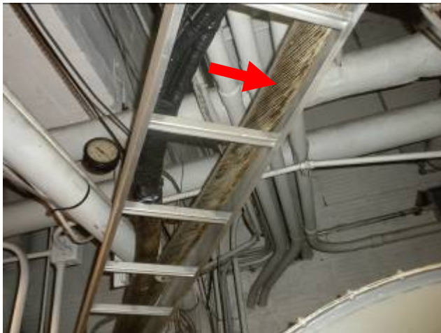
Unprotected 13,200-Volt Cable
