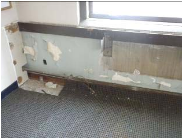
Wall & Carpet Damage
