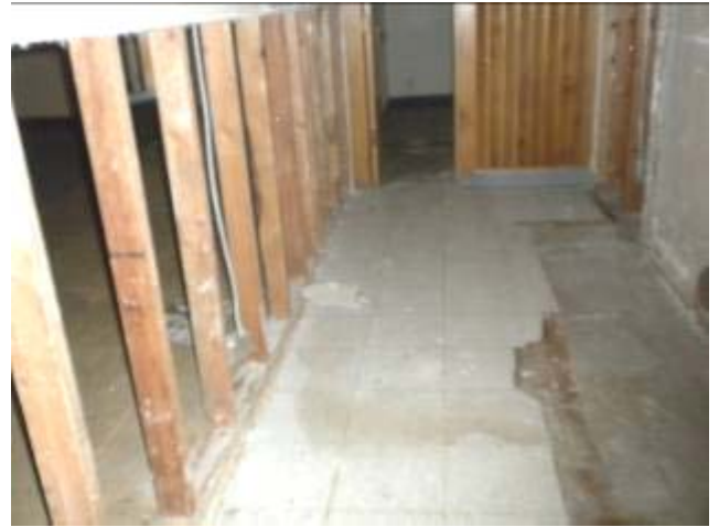
Office Wall & Floor Damage
