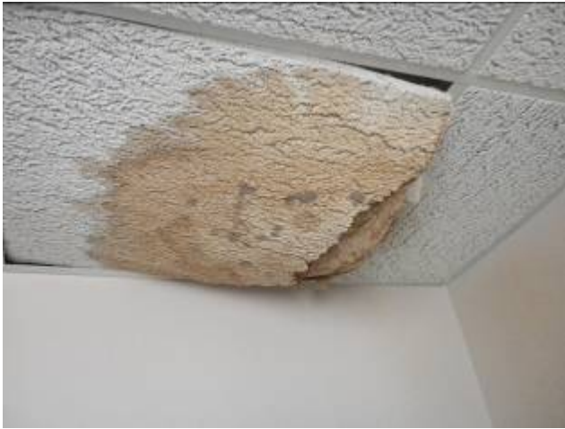
Office Ceiling Damage & Mold
