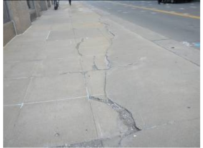
Sidewalk Damage Along Baltimore Avenue
