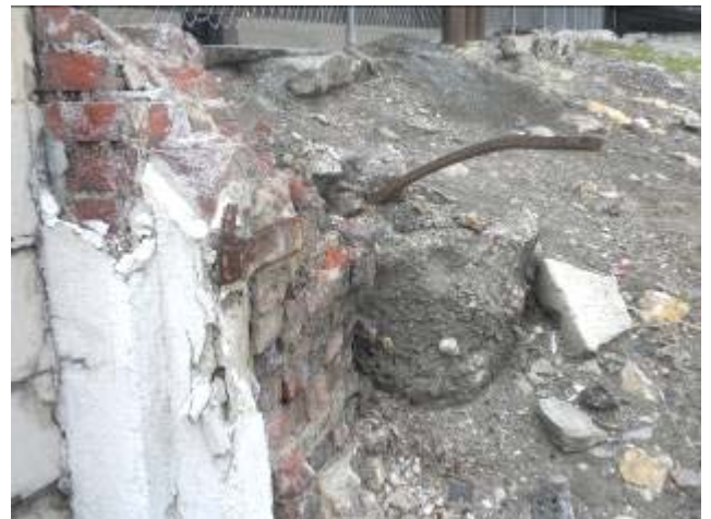
Deteriorating Retaining Wall/Foundation
