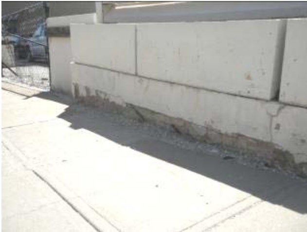
Deteriorating Wall Fronting Baltimore Avenue
