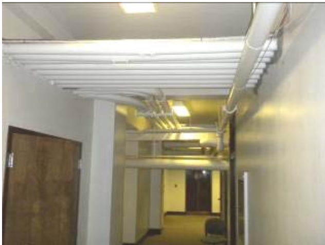
Extensive Asbestos Pipe Wrapping
