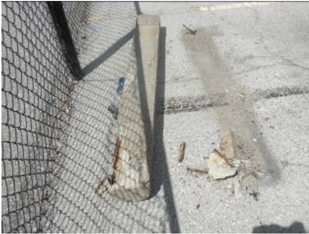
Deteriorating Parking Blocks
