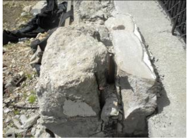
Deteriorating Retaining Wall/Foundation
