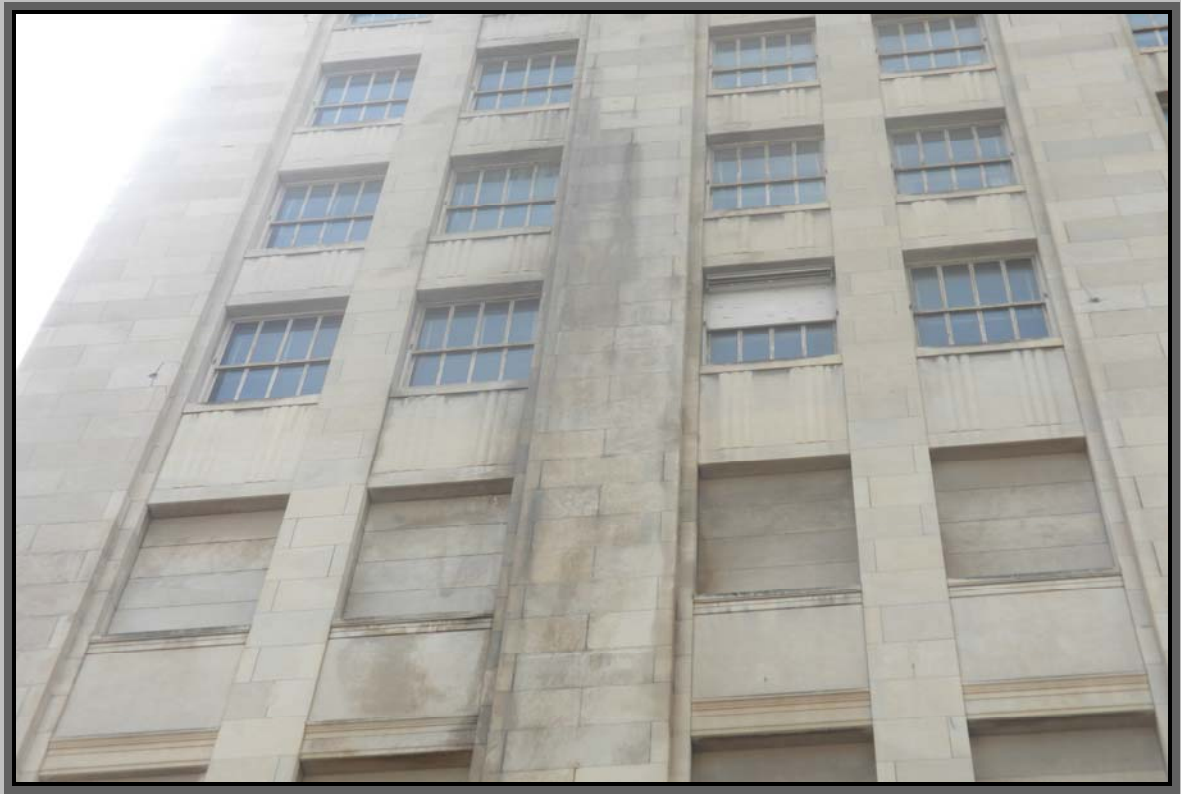
The 14 th & Baltimore PIEA Planning Area – Resolving Exterior Deterioration
