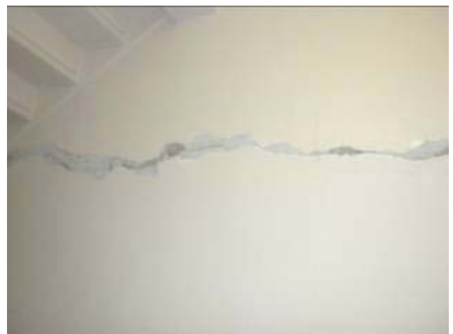
Crack In Stairwell Wall
