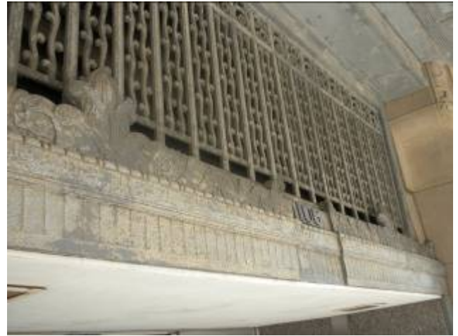
Deteriorating Art Deco Features
