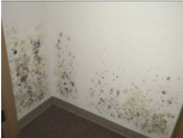
Mold In Office Walls
