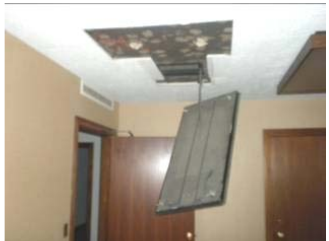
Collapsed 4'x4' Light Fixture
