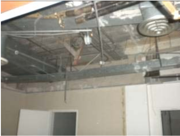
Office Ceiling Damage
