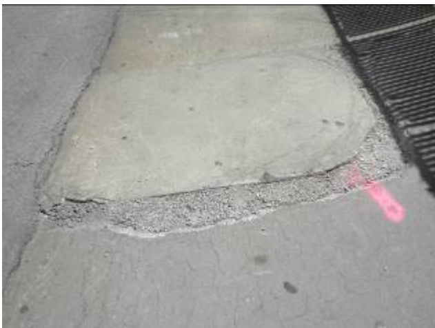
Sidewalk Damage Along W 13 th Street
