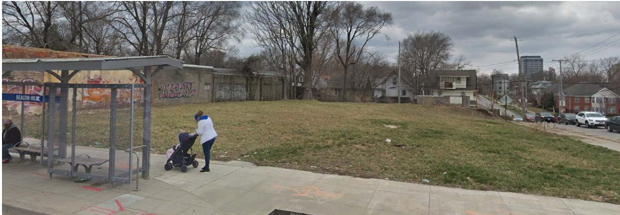
1015 E. 27 th Street/2702 Troost Avenue – trash and debris scattered across entire site; uneven grading; weeds and overgrown grass
