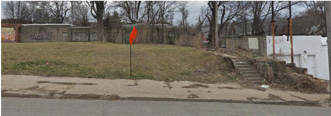
1015 E. 27 th Street/2702 Troost Avenue – broken/deteriorating sidewalk & curb; deteriorating stairs and retaining wall
