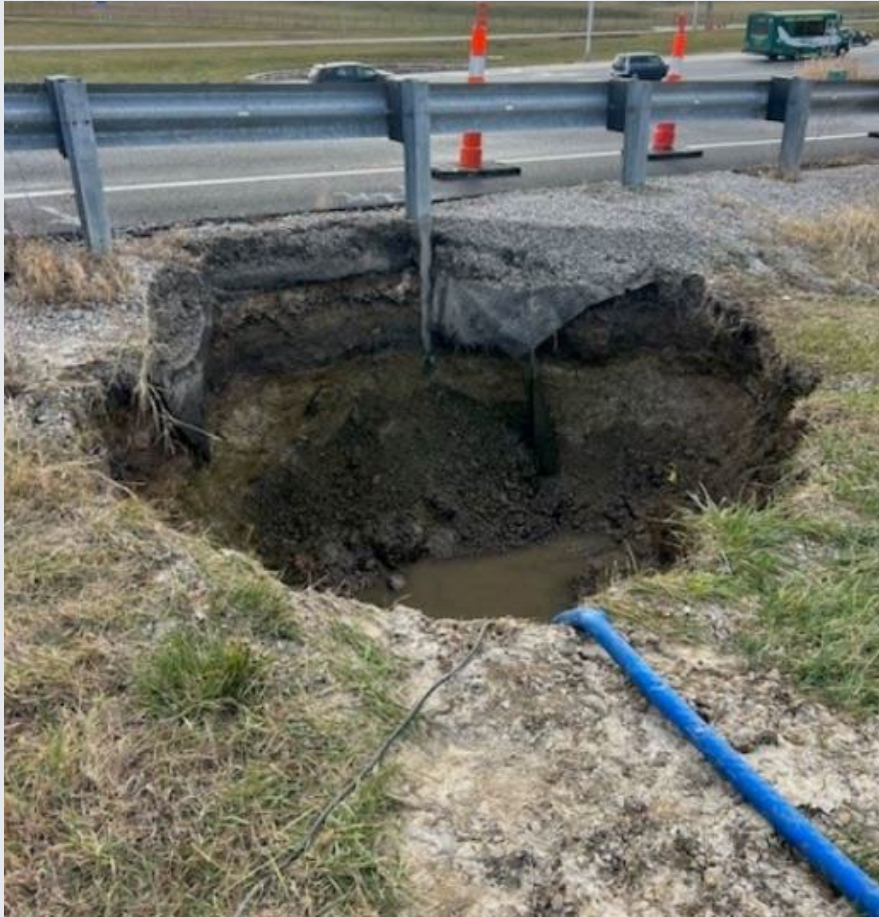
Water Main Break Aftermath
