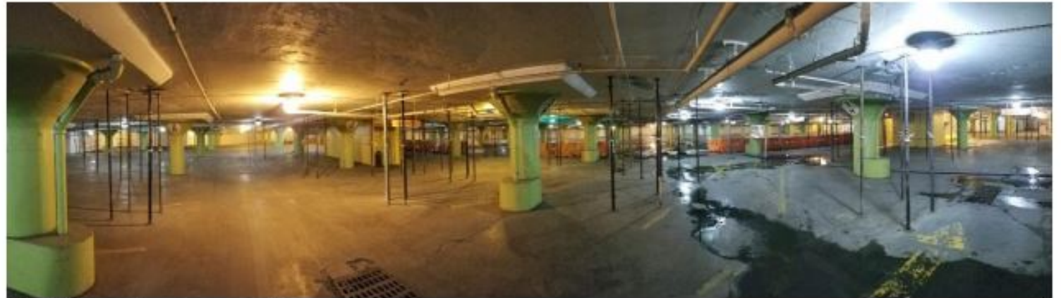
Fig. XX Lower level garage lighting
