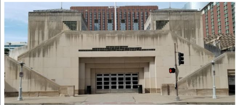
Fig. XX No discernable egress lights at south street exit
