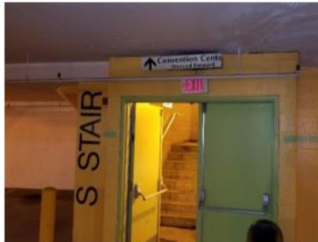
Fig. XX Exit sign at door
