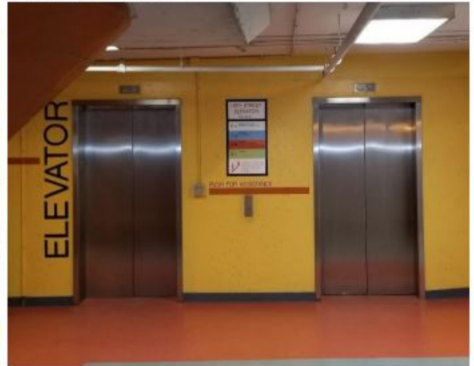
Fig. XX Call station at elevators
