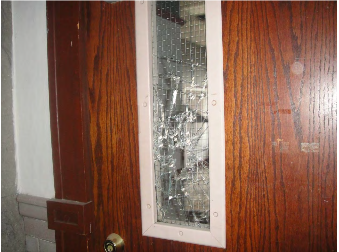
Photo 56 – Deteriorating Site Condition.
