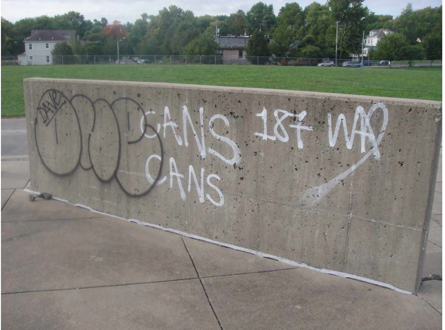
Photo 47 – Deteriorated Site Improvements.
