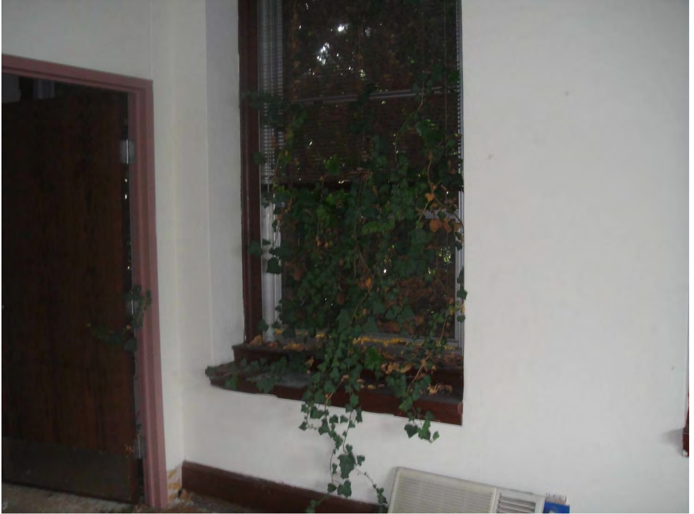
Photo 28 – Deteriorated Site Improvements.
