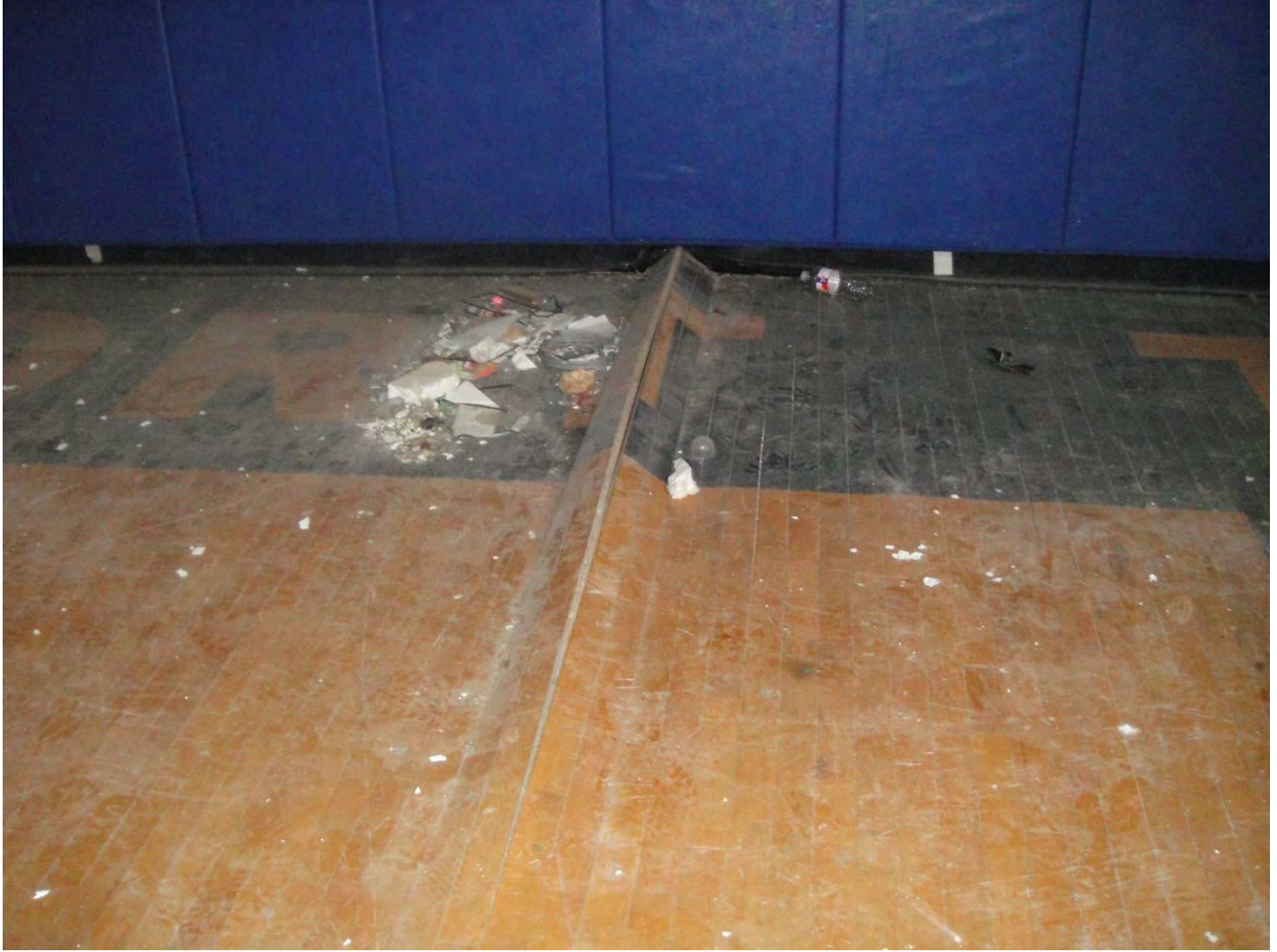
Photo 65 – Deteriorated Site Improvements.
