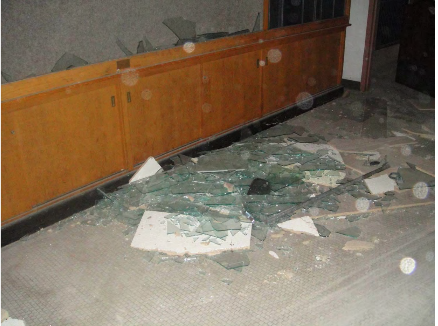
Photo 44 – Deteriorated Site Improvements.
