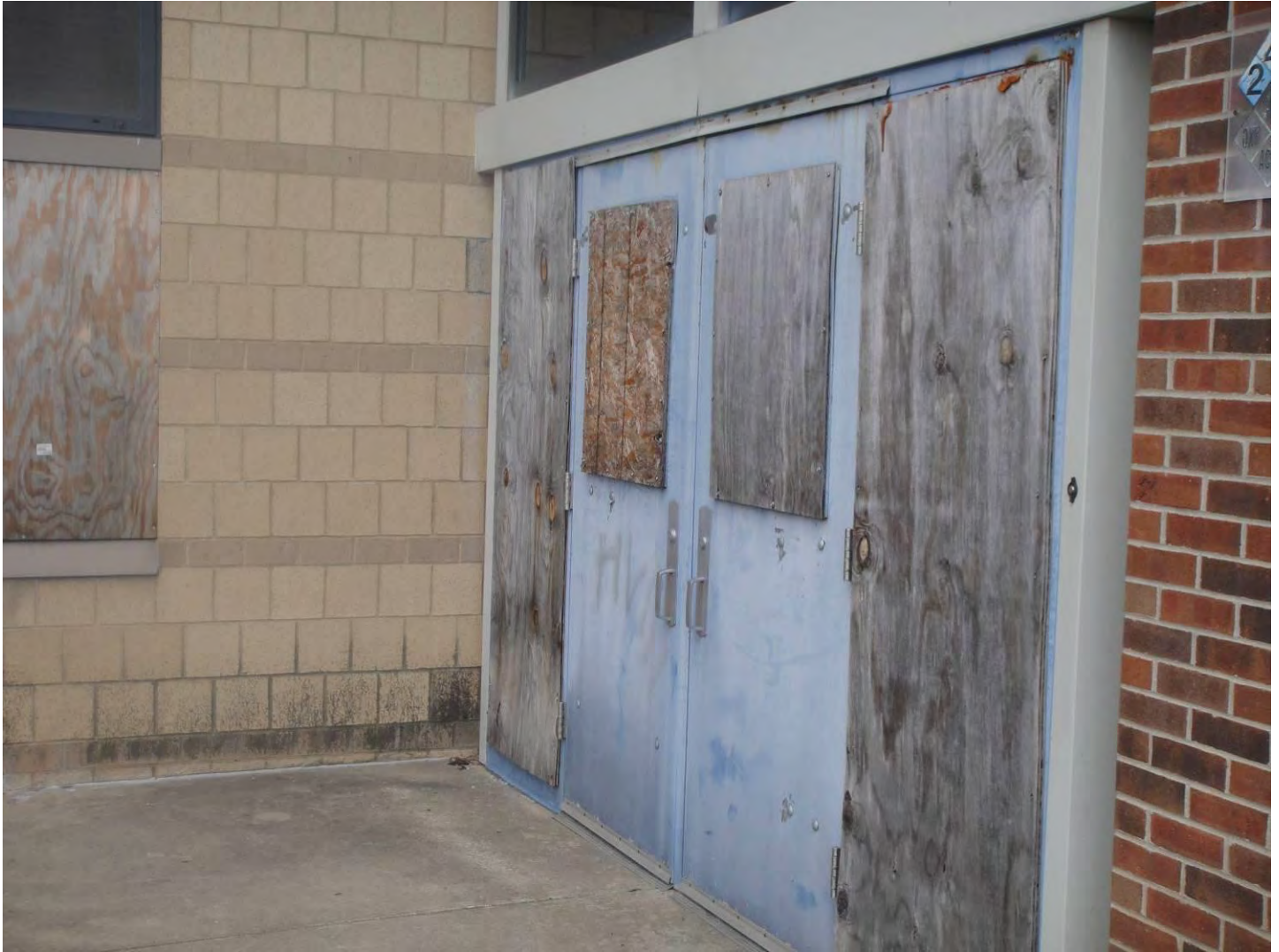
Photo 24 – Deteriorated Site Improvements.
