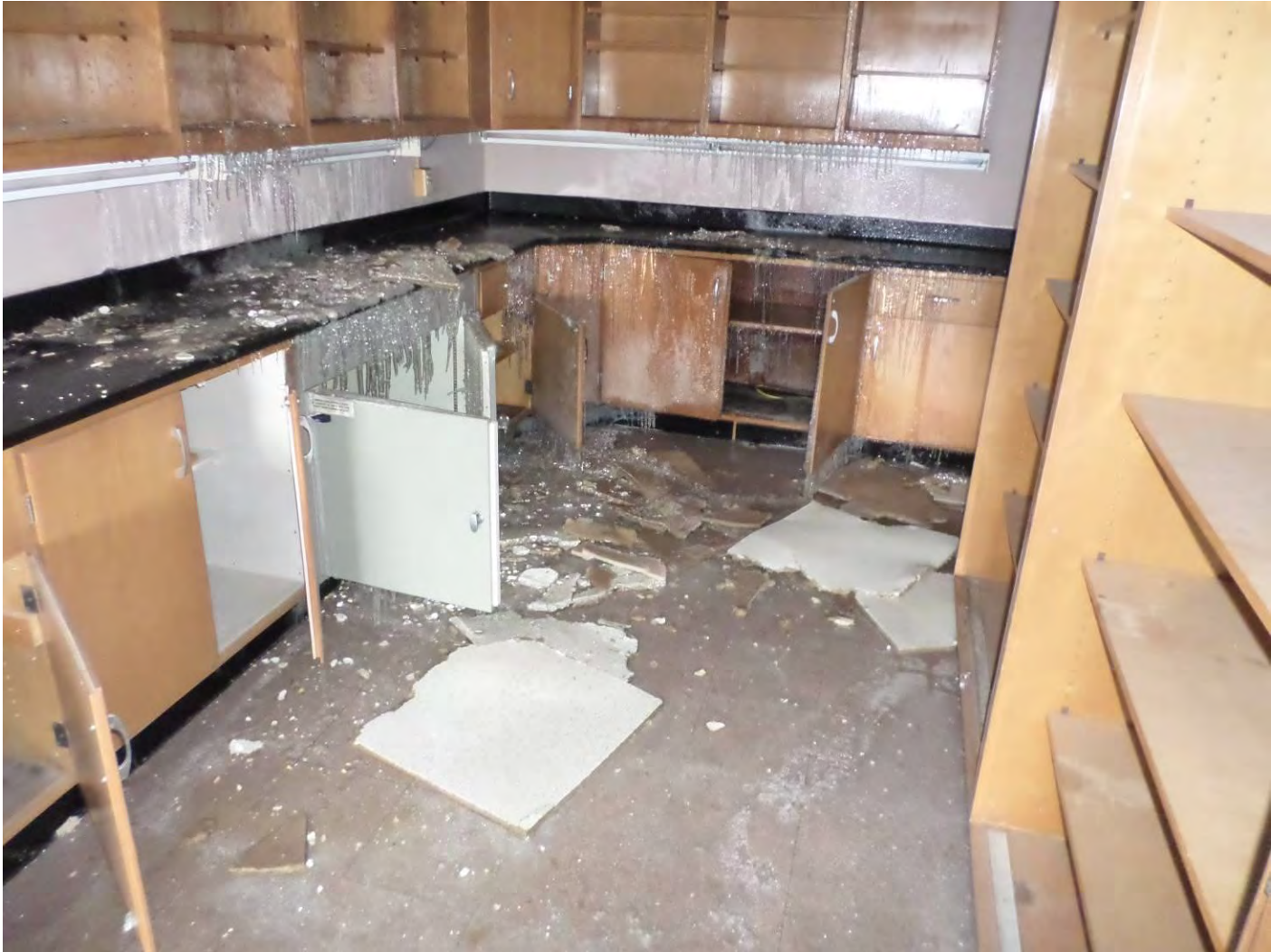
Photo 38 – Deteriorated Site Improvements. Photo courtesy property owner.
