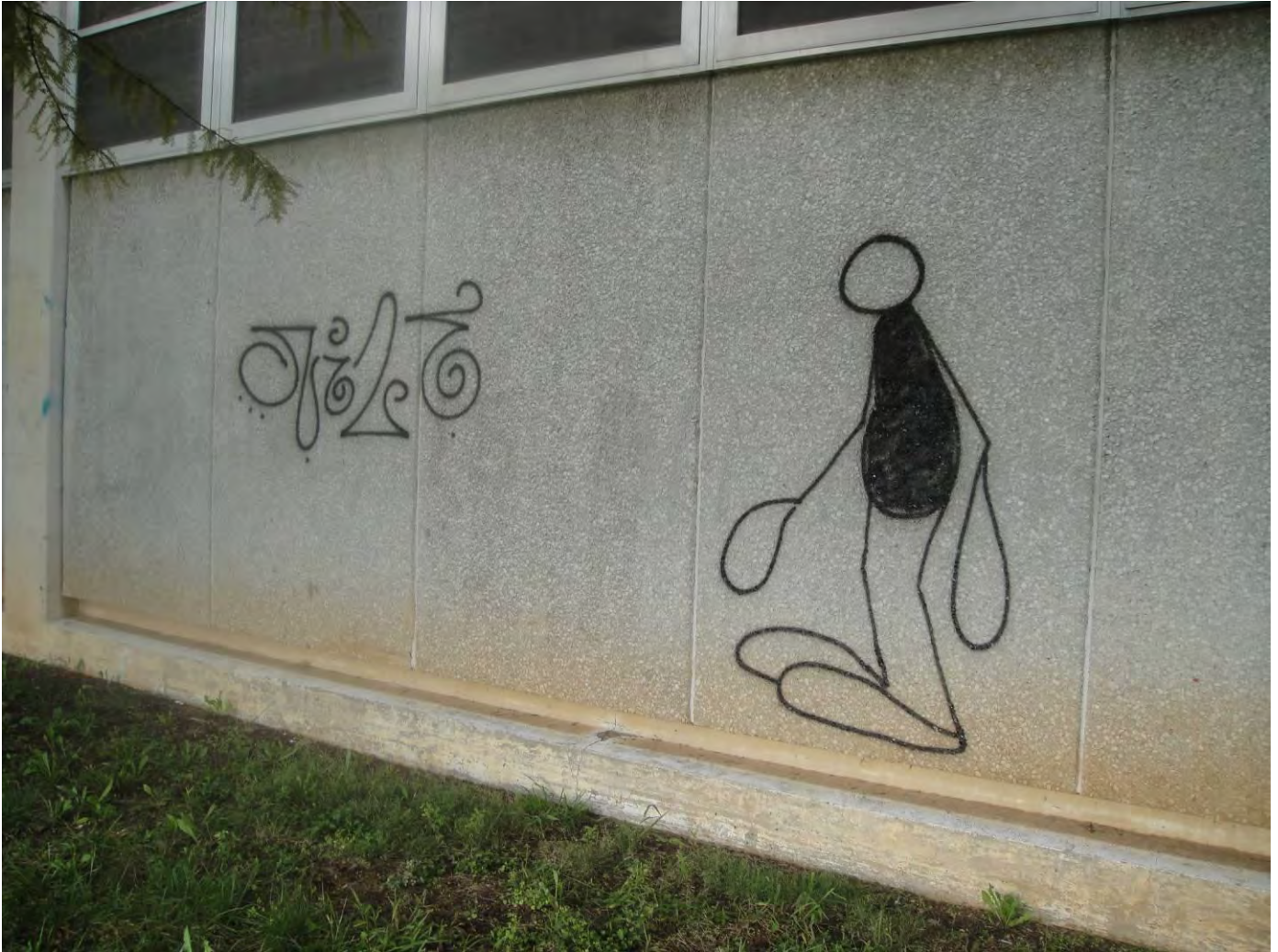
Photo 20 – Deteriorated Site Improvements.
