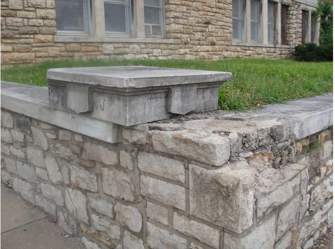
Photo 31 – Deteriorated Site Improvements. Damaged, deteriorated column capital on retaining wall.
