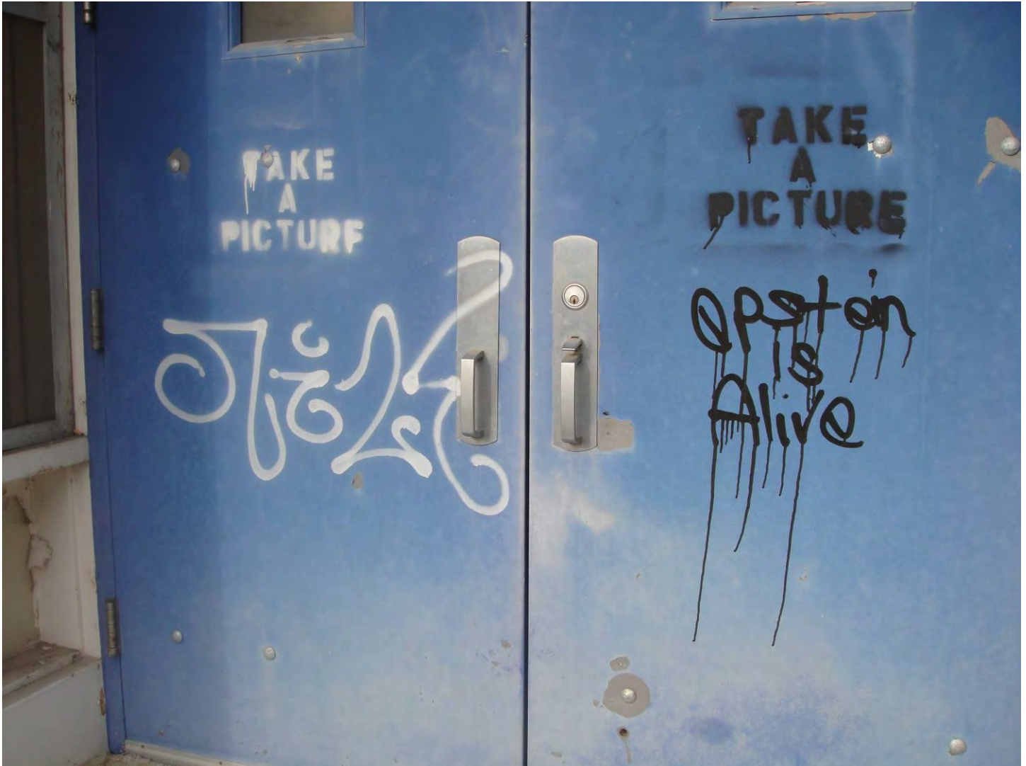
Photo 49 – Deteriorated Site Improvements.
