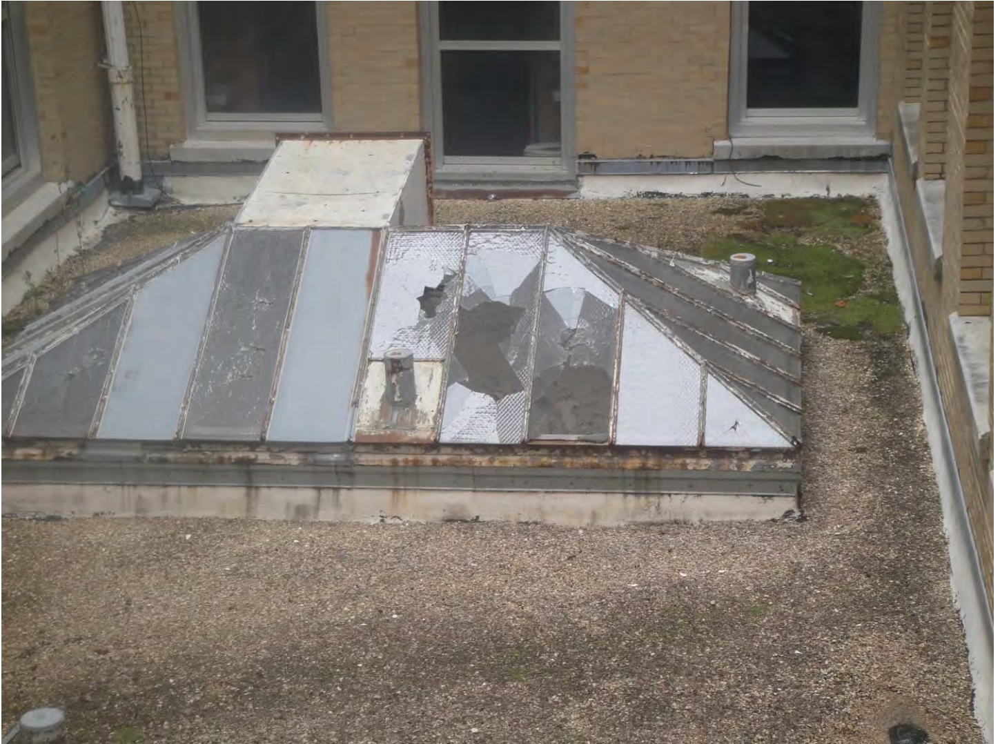
Photo 34 – Deteriorated Site Improvements.
