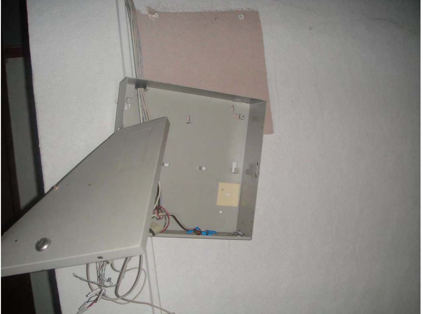
Photo 59 – Deterioration of Site Improvements.
