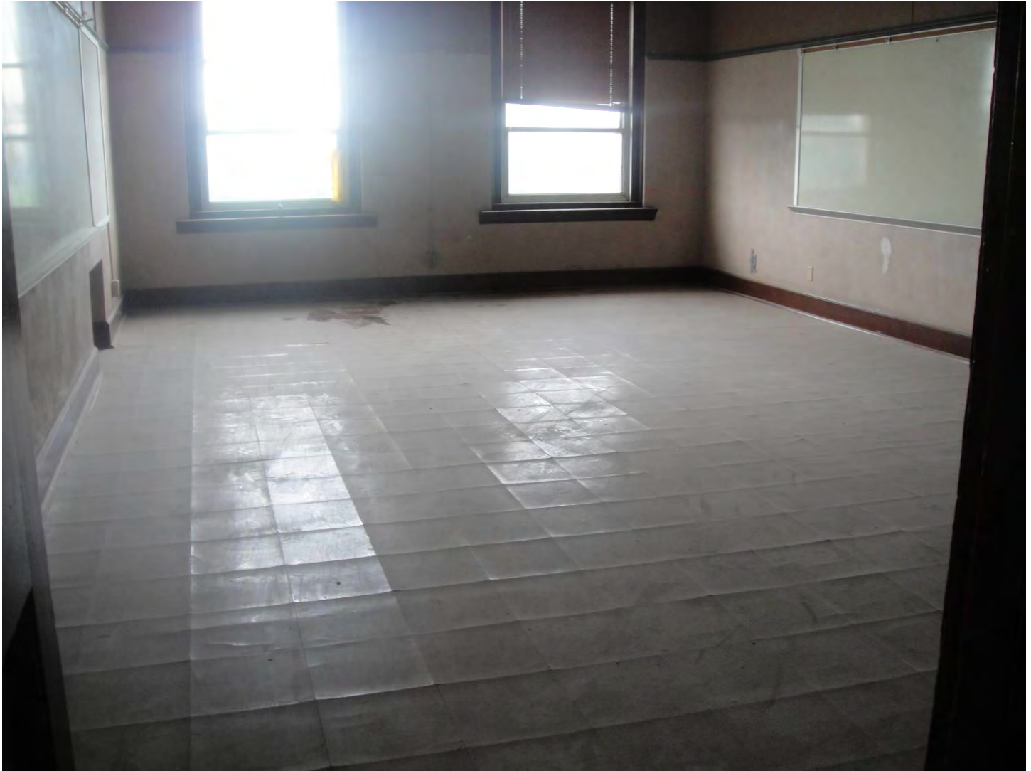
Photo 39 – Deteriorated Site Improvements.
