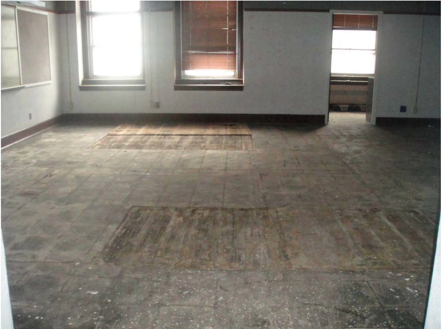
Photo 58 – Deteriorated Site Conditions.
