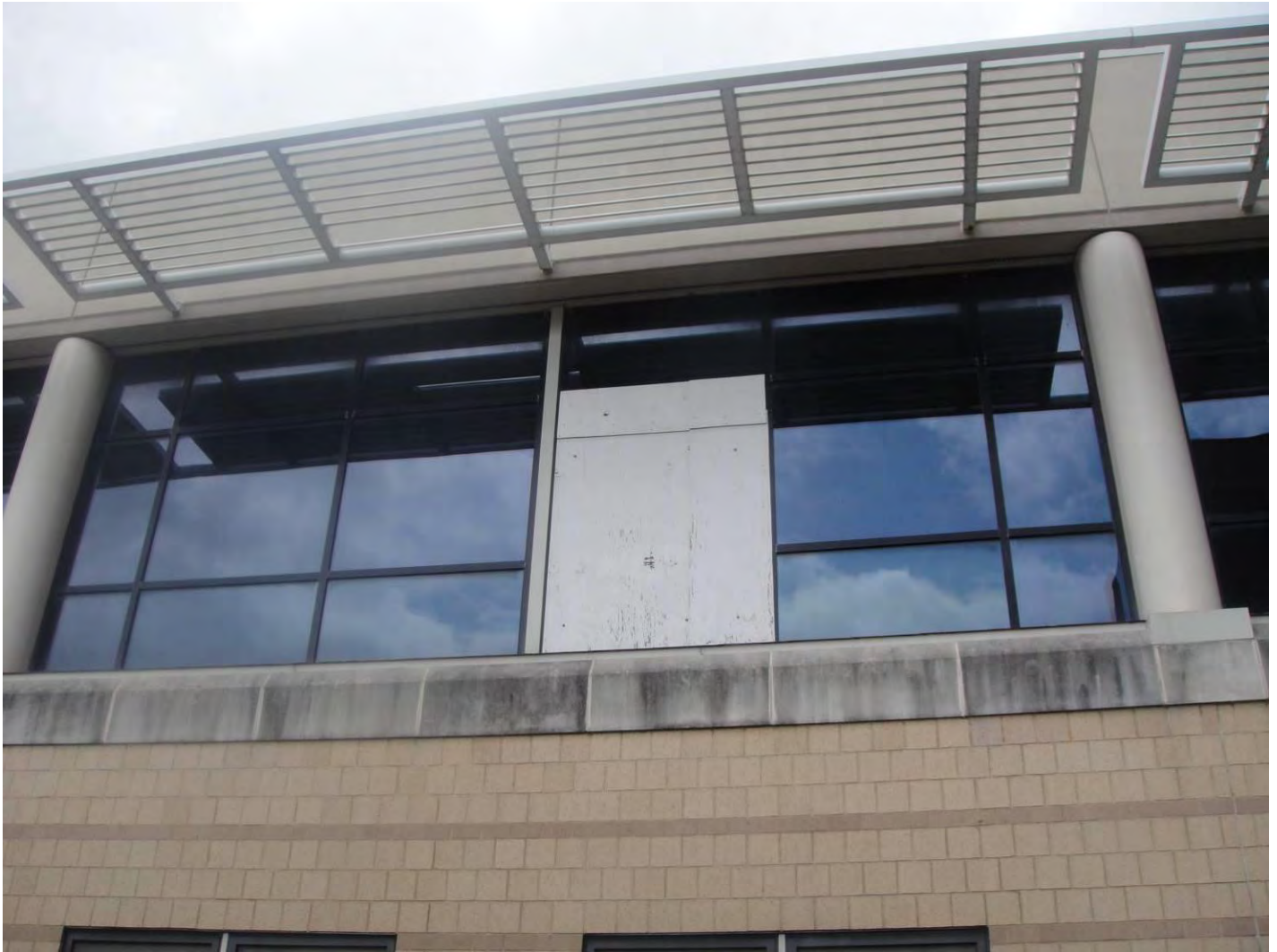
Photo 22 – Deteriorated Site Improvements.
