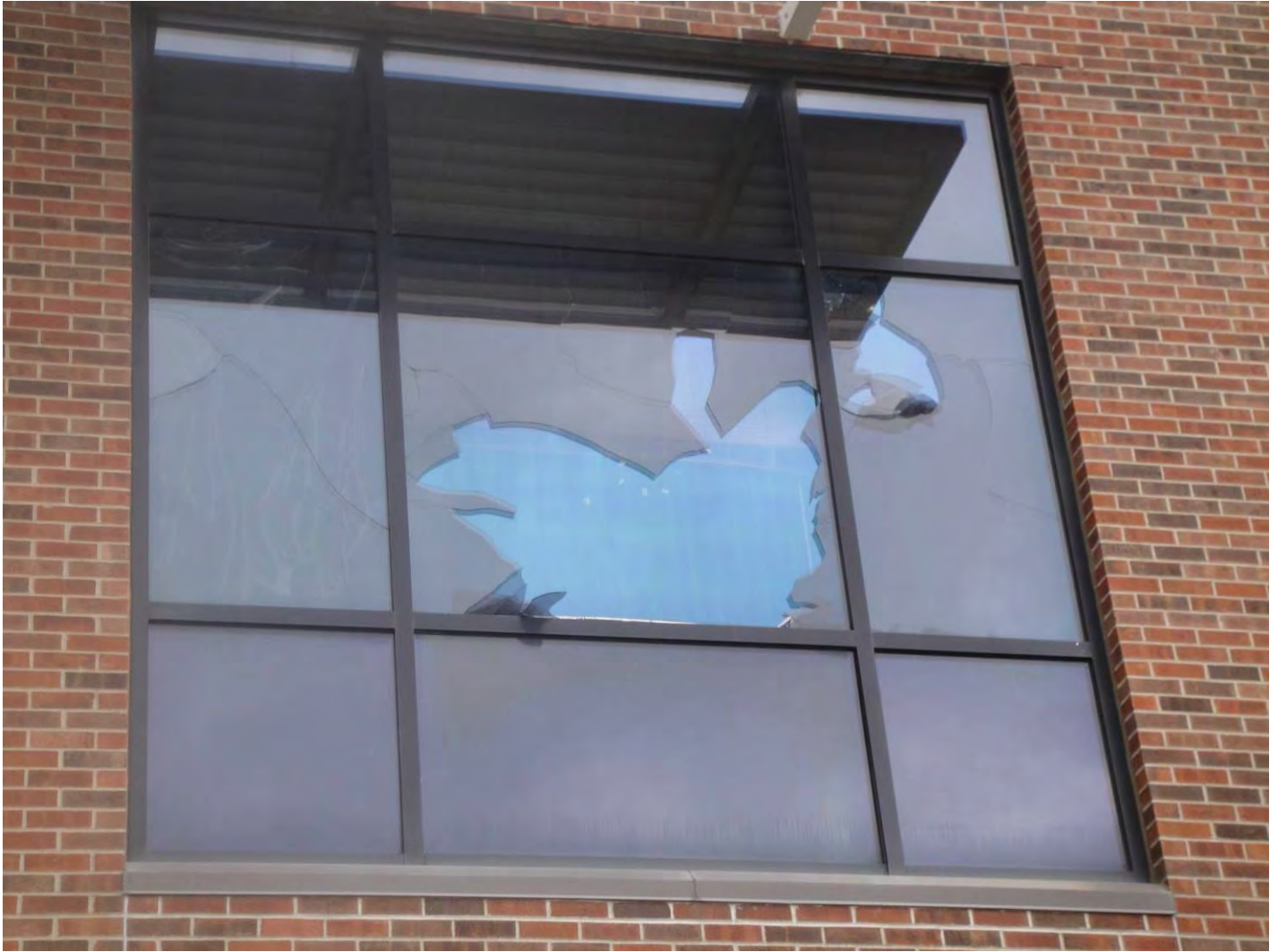
Photo 23 – Deteriorated Site Improvements.
