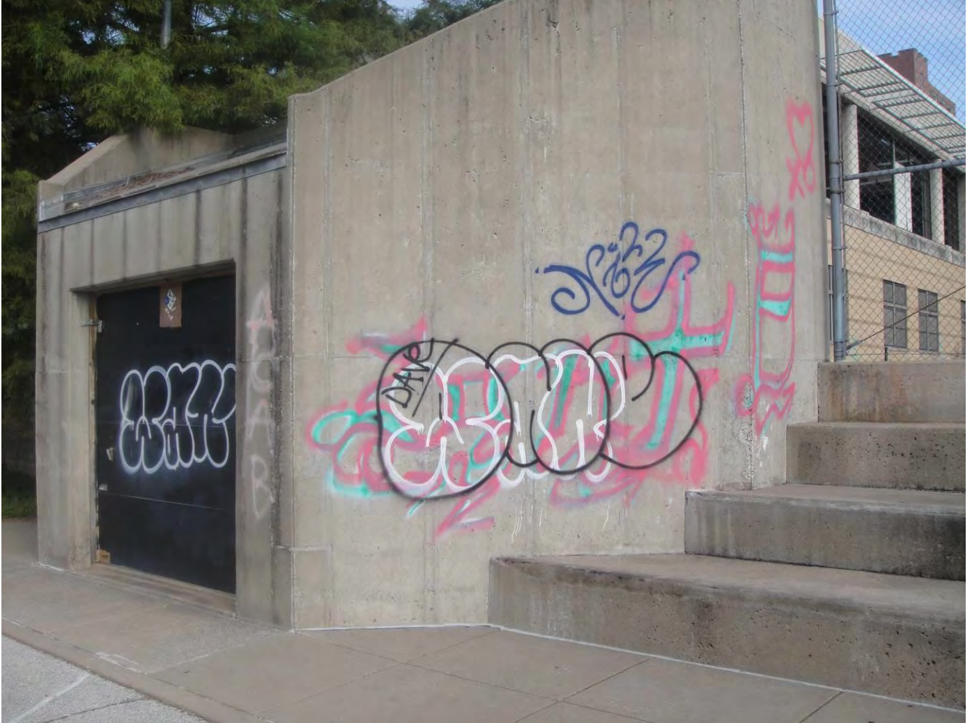
Photo 21 – Deteriorated Site Improvements.
