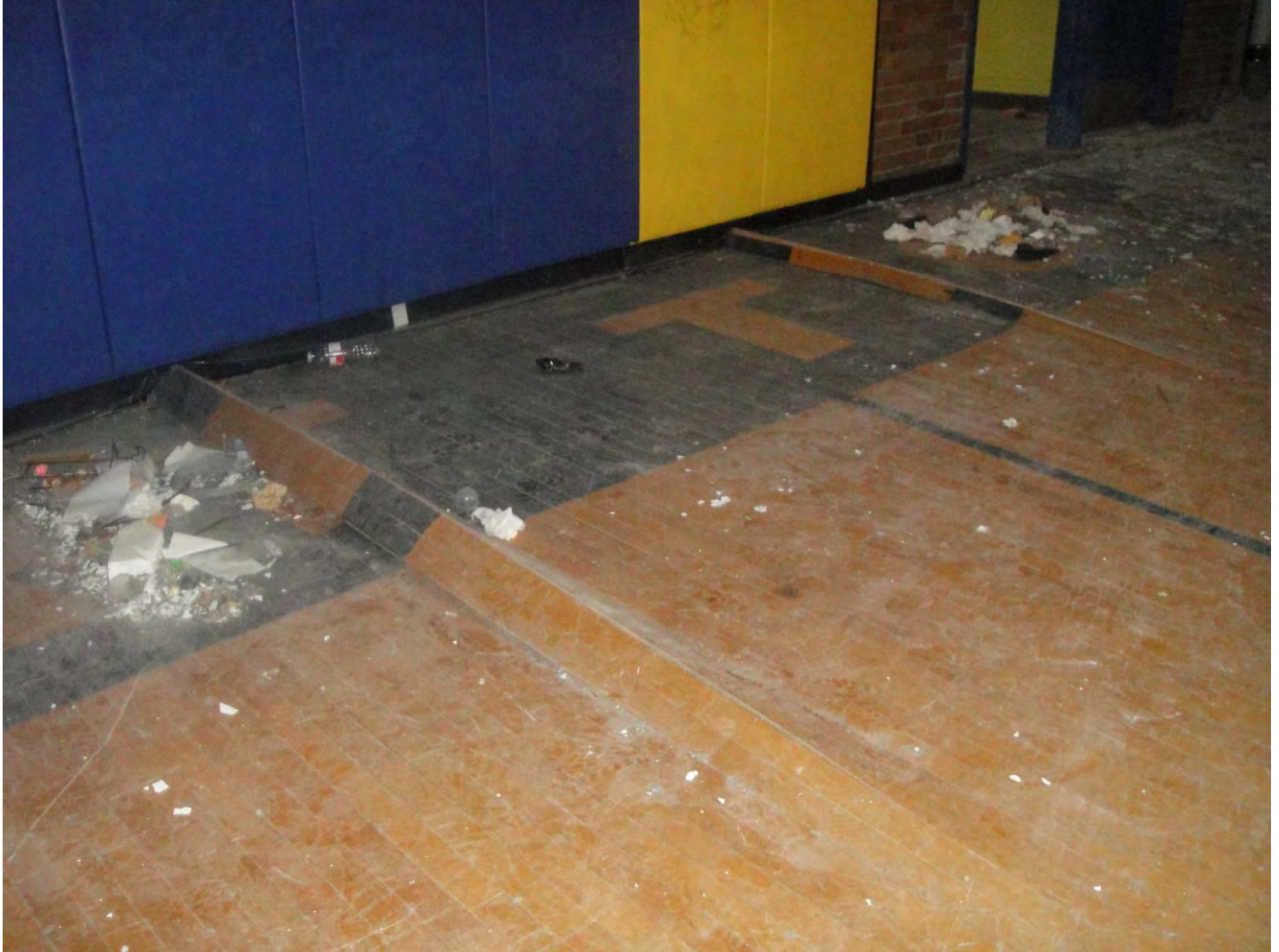
Photo 66 – Deteriorated Site Improvements.
