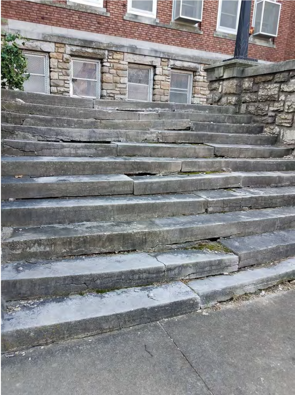
Photo 50 – Deteriorated Site Improvements.
