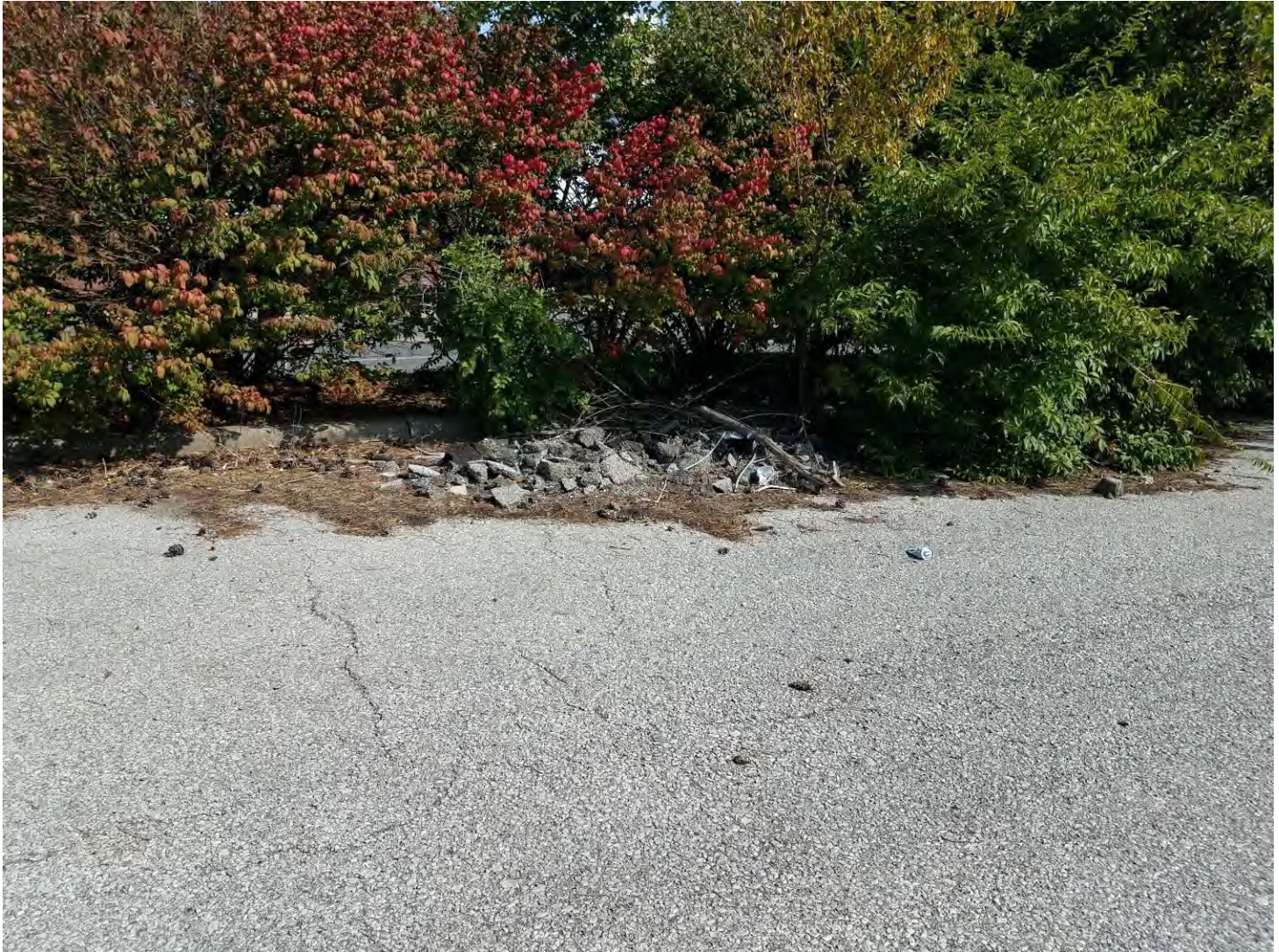
Photo 72 – Deteriorated Site Improvements.
