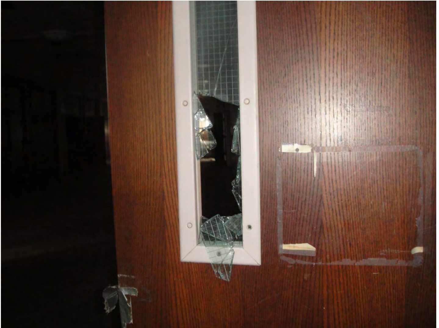
Photo 52 – Deterioration of Site Conditions.
