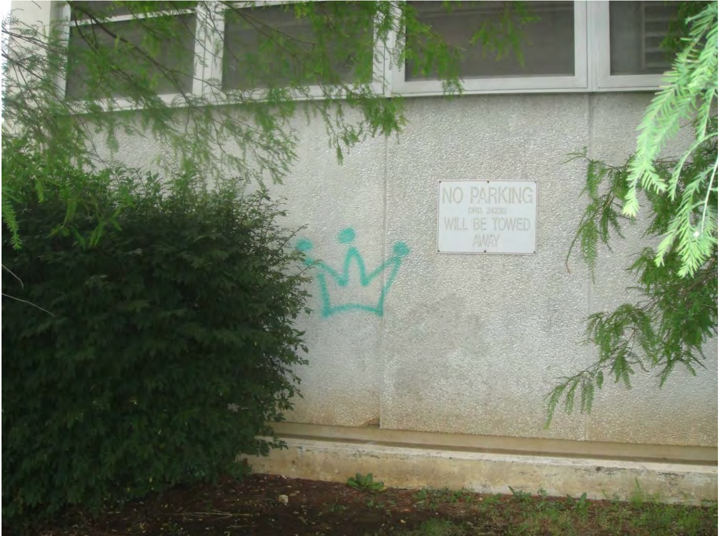
Photo 18 – Deteriorated Site Improvements.
