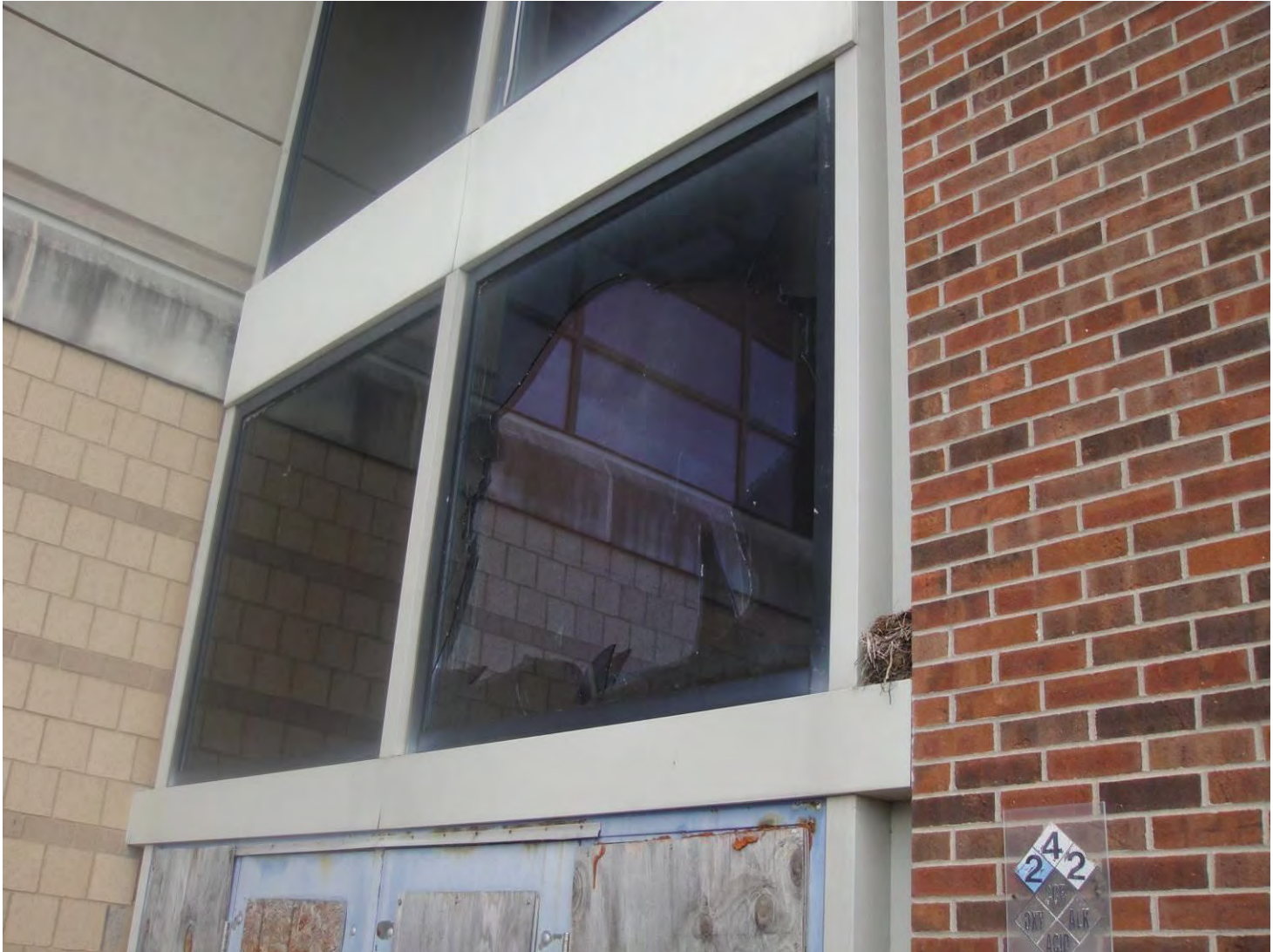
Photo 25 – Deteriorated Site Improvements.
