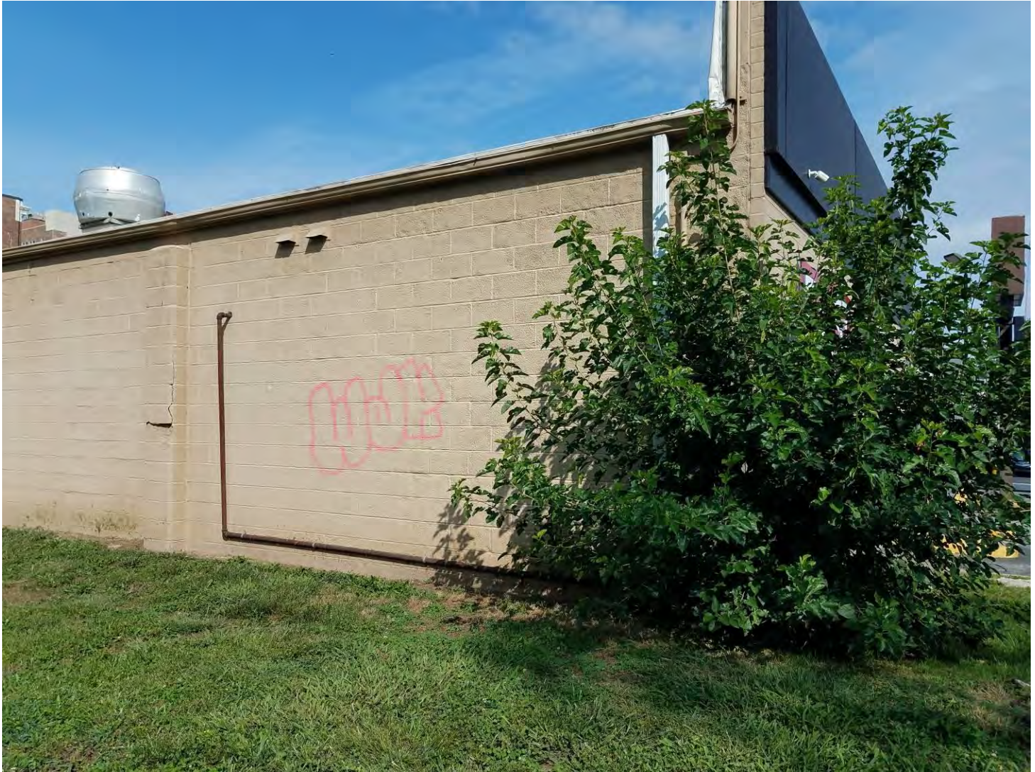
Photo 71 – Deteriorated Site Improvements.
