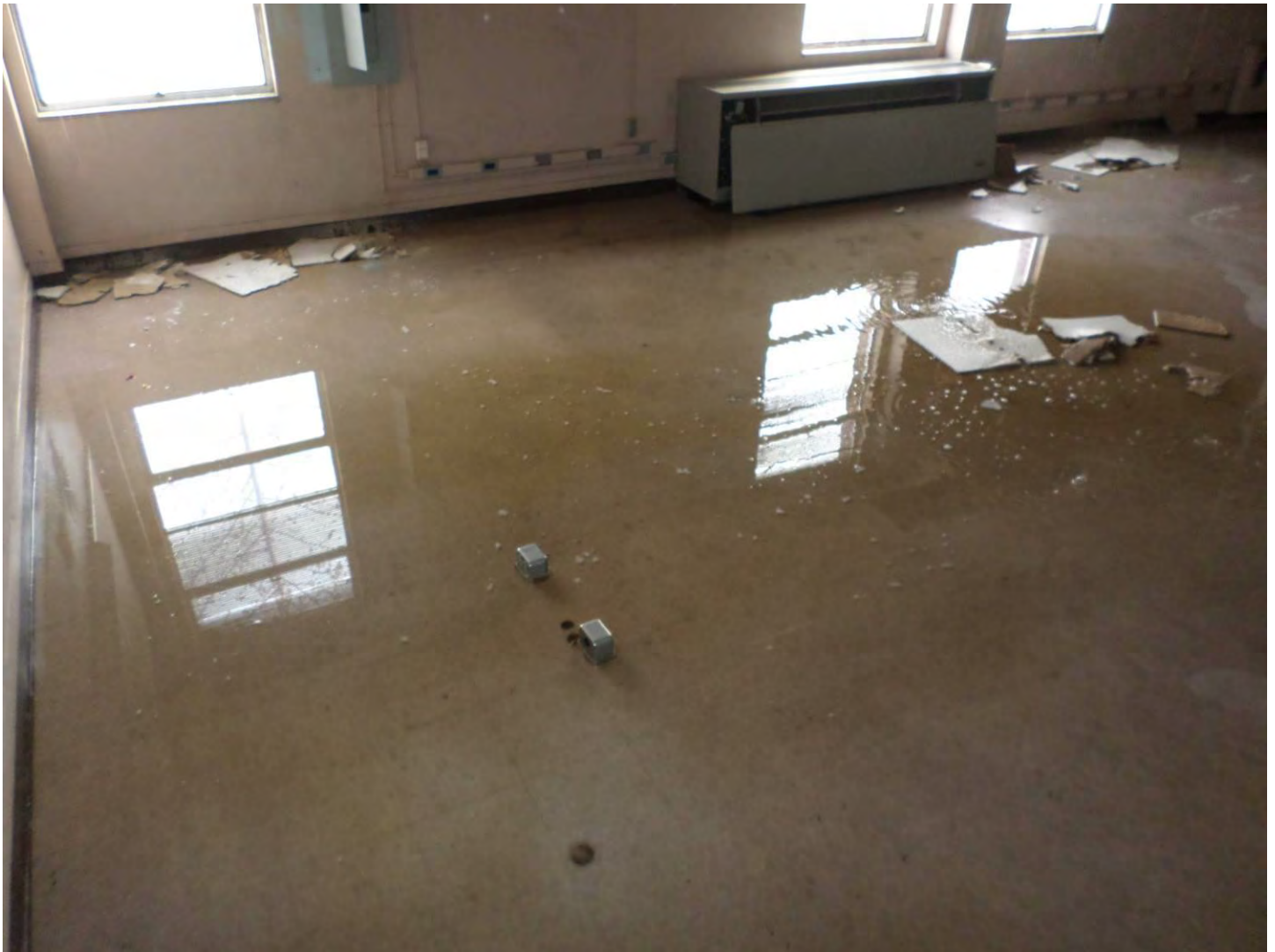
Photo 37 – Deteriorated Site Improvements. Photo courtesy property owner.
