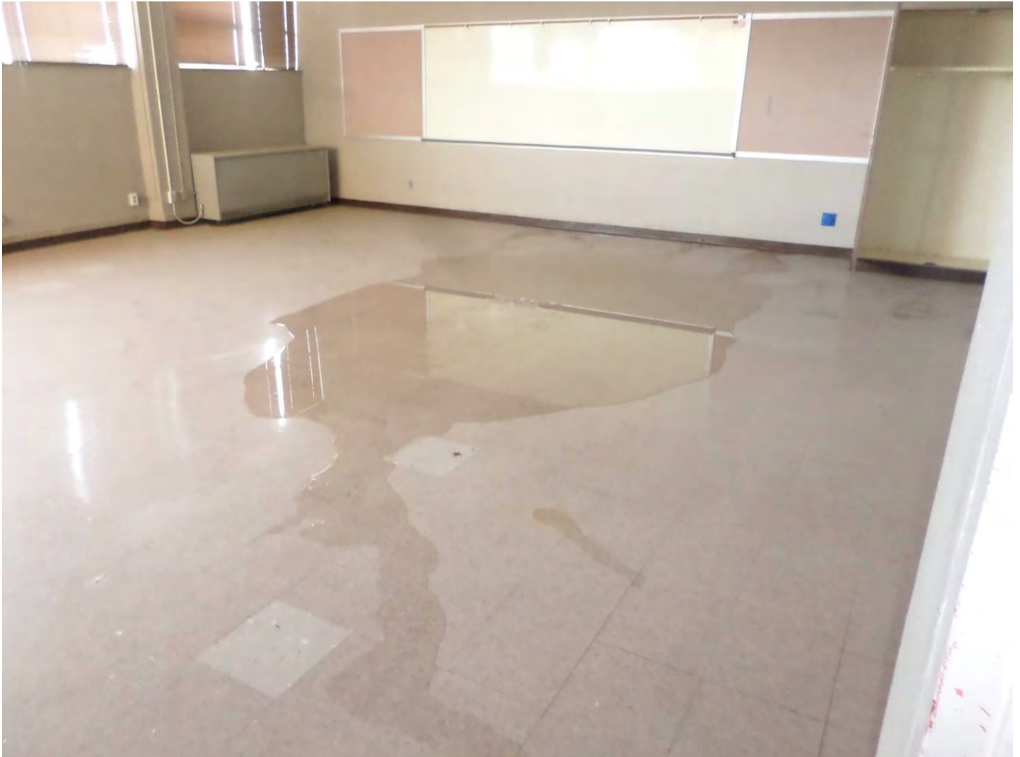
Photo 35 – Deteriorated Site Improvements. Photo courtesy property owner.
