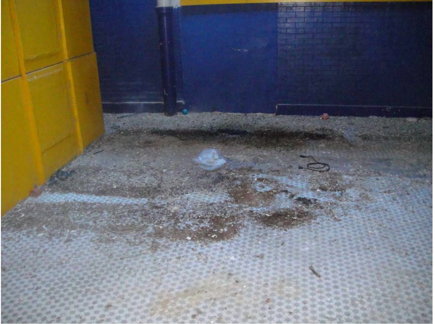
Photo 9 – Insanitary or unsafe conditions.
