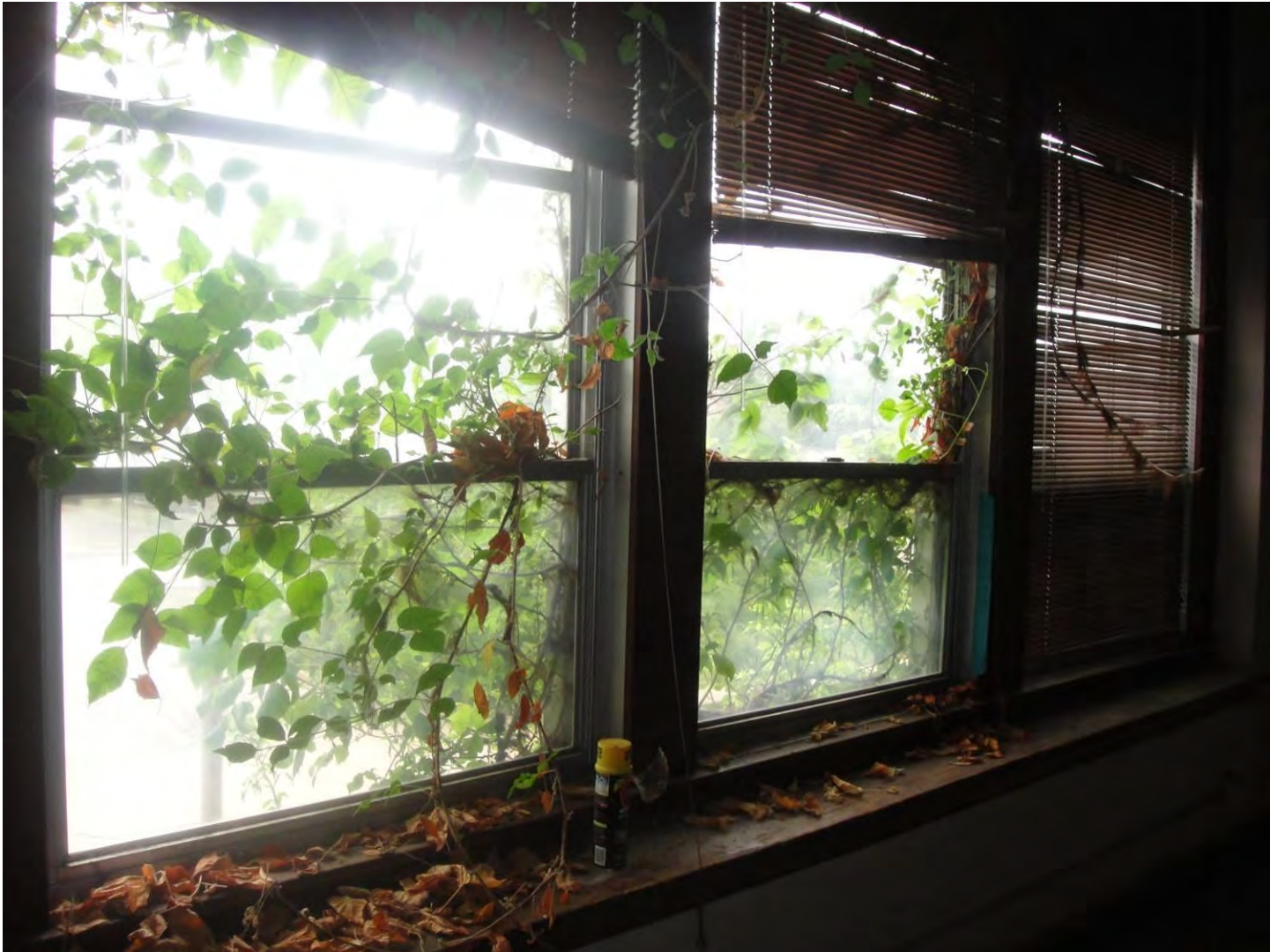
Photo 29 – Deteriorated Site Improvements.
