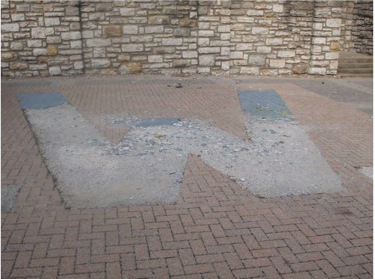
Photo 68 – Deteriorated Site Improvements.
