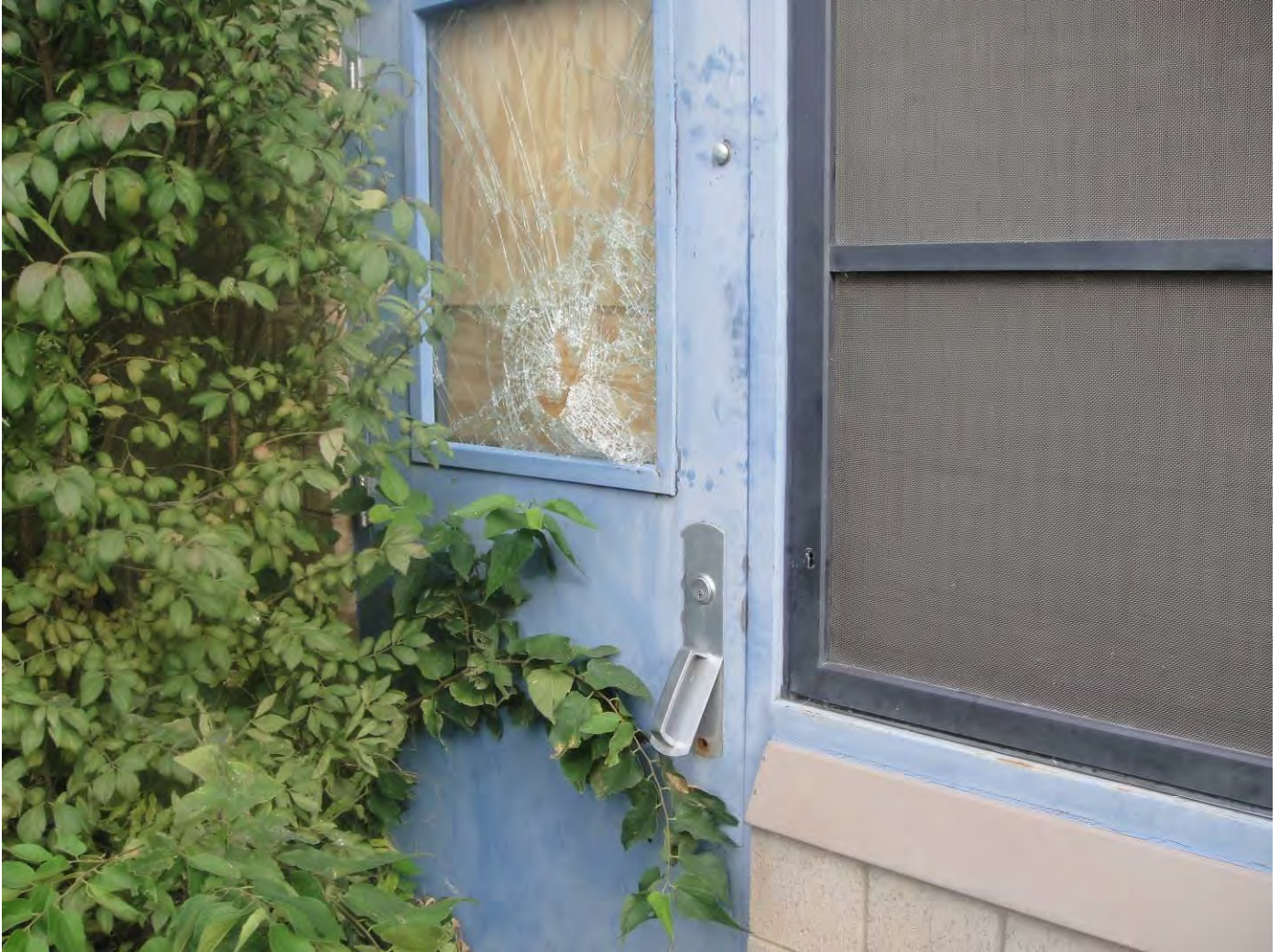
Photo 27 – Deteriorated Site Improvements.
