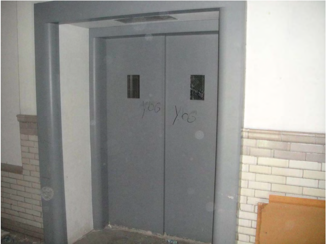
Photo 57 – Deteriorating Site Condition.
