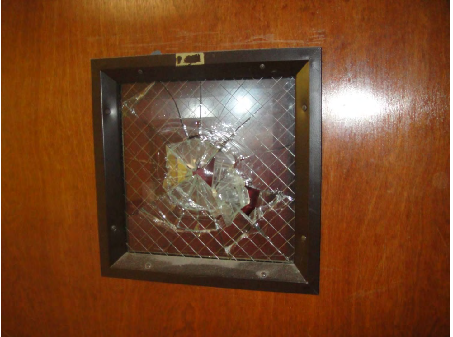
Photo 54 – Deteriorating Site Condition.
