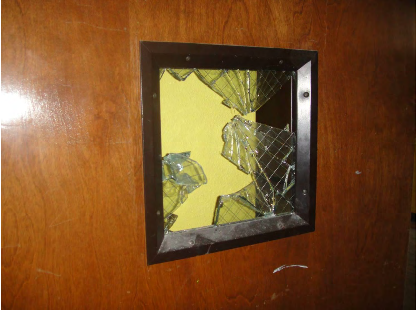
Photo 55 – Deteriorating Site Condition.
