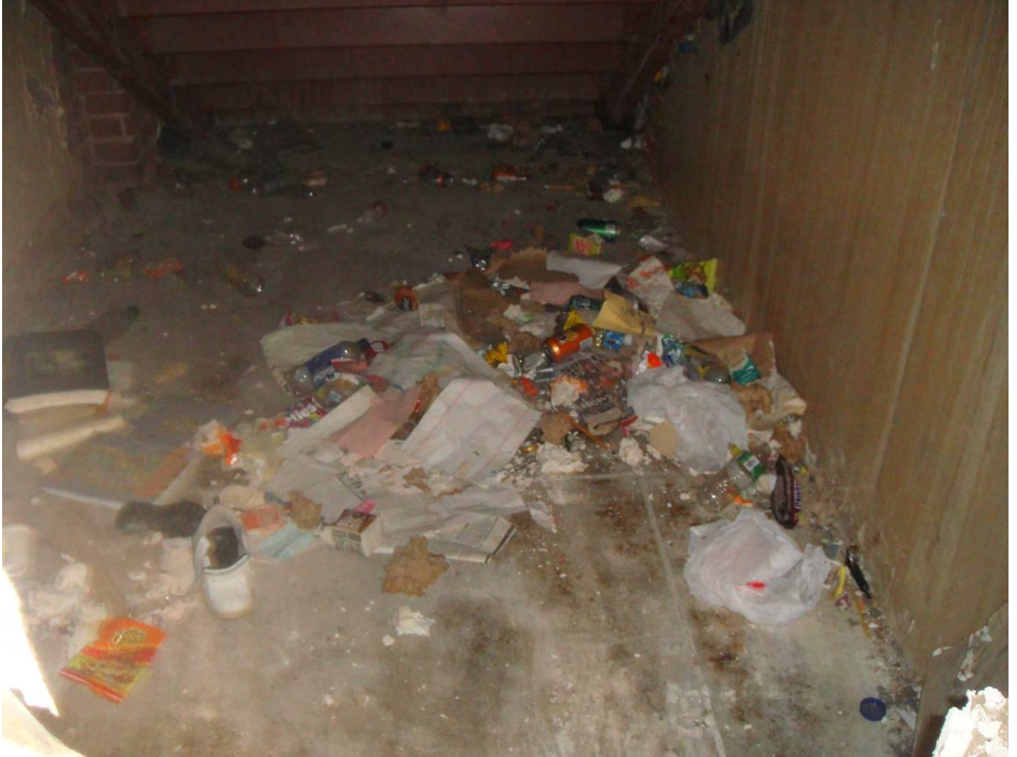
Photo 62 – Deteriorated Site Improvements.
