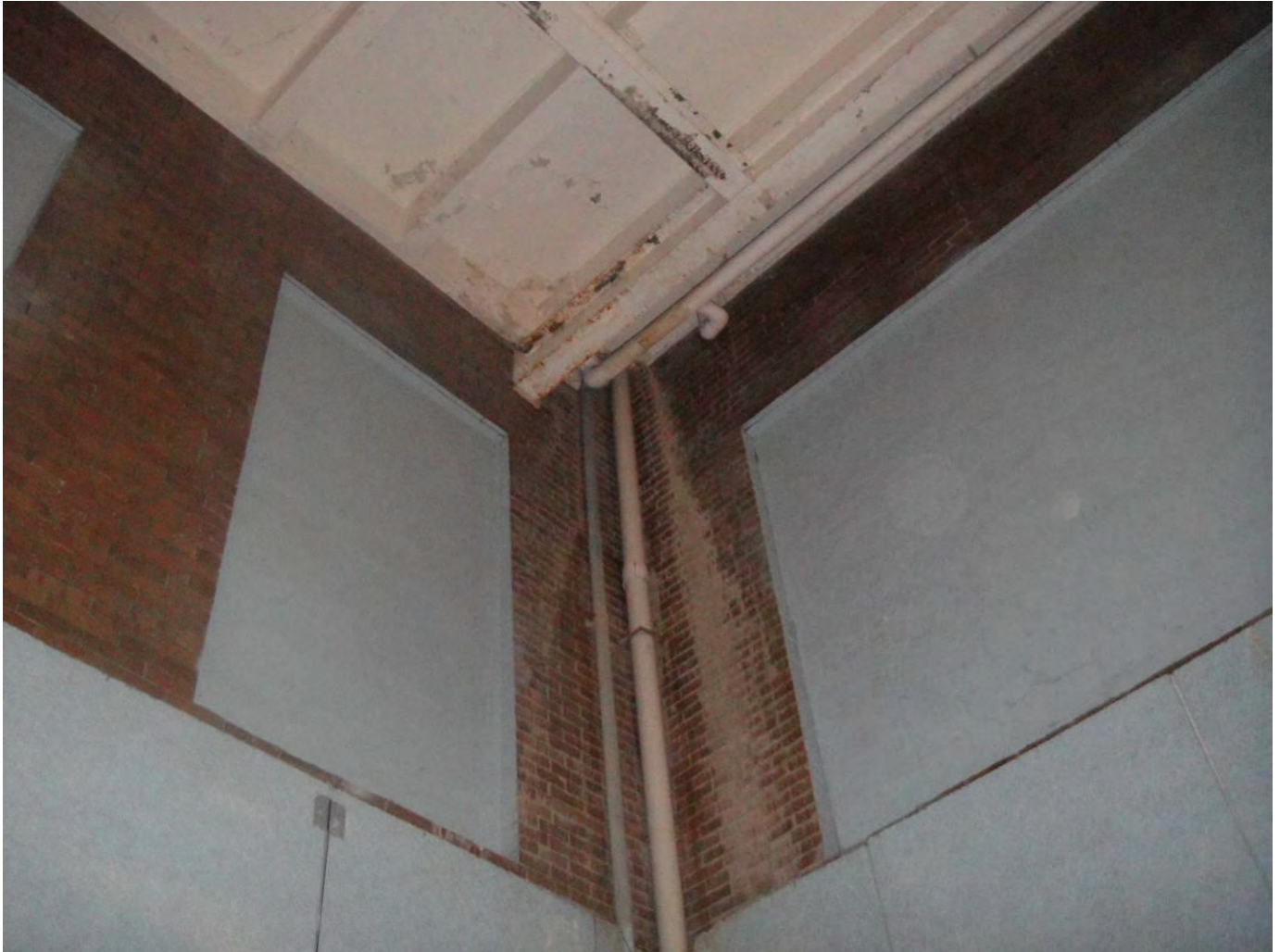
Photo 63 – Deteriorated Site Improvements.
