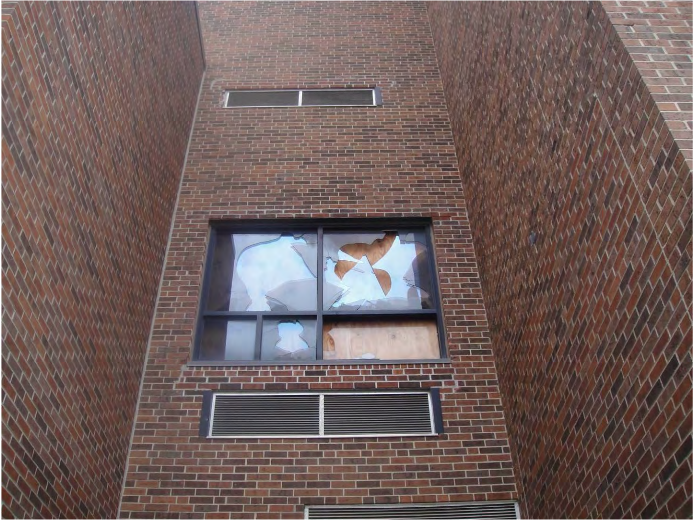
Photo 26 – Deteriorated Site Improvements.
