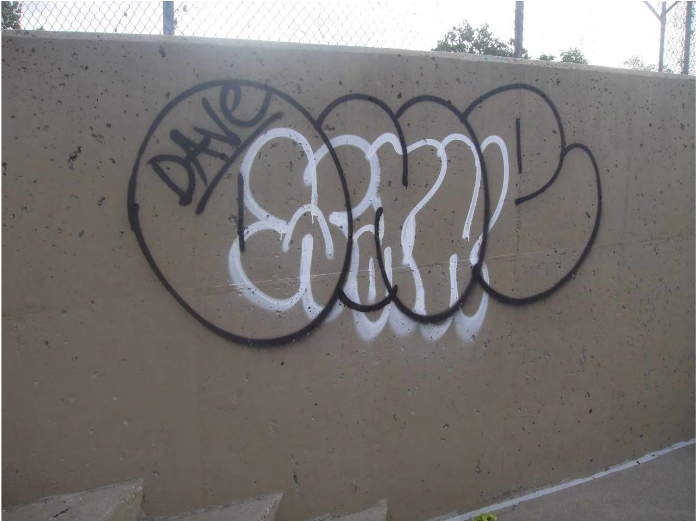
Photo 48 – Deteriorated Site Improvements.
