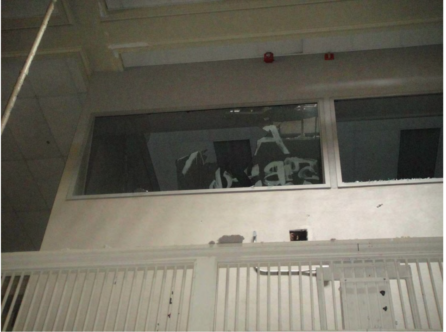
Photo 43 – Deteriorated Site Improvements.
