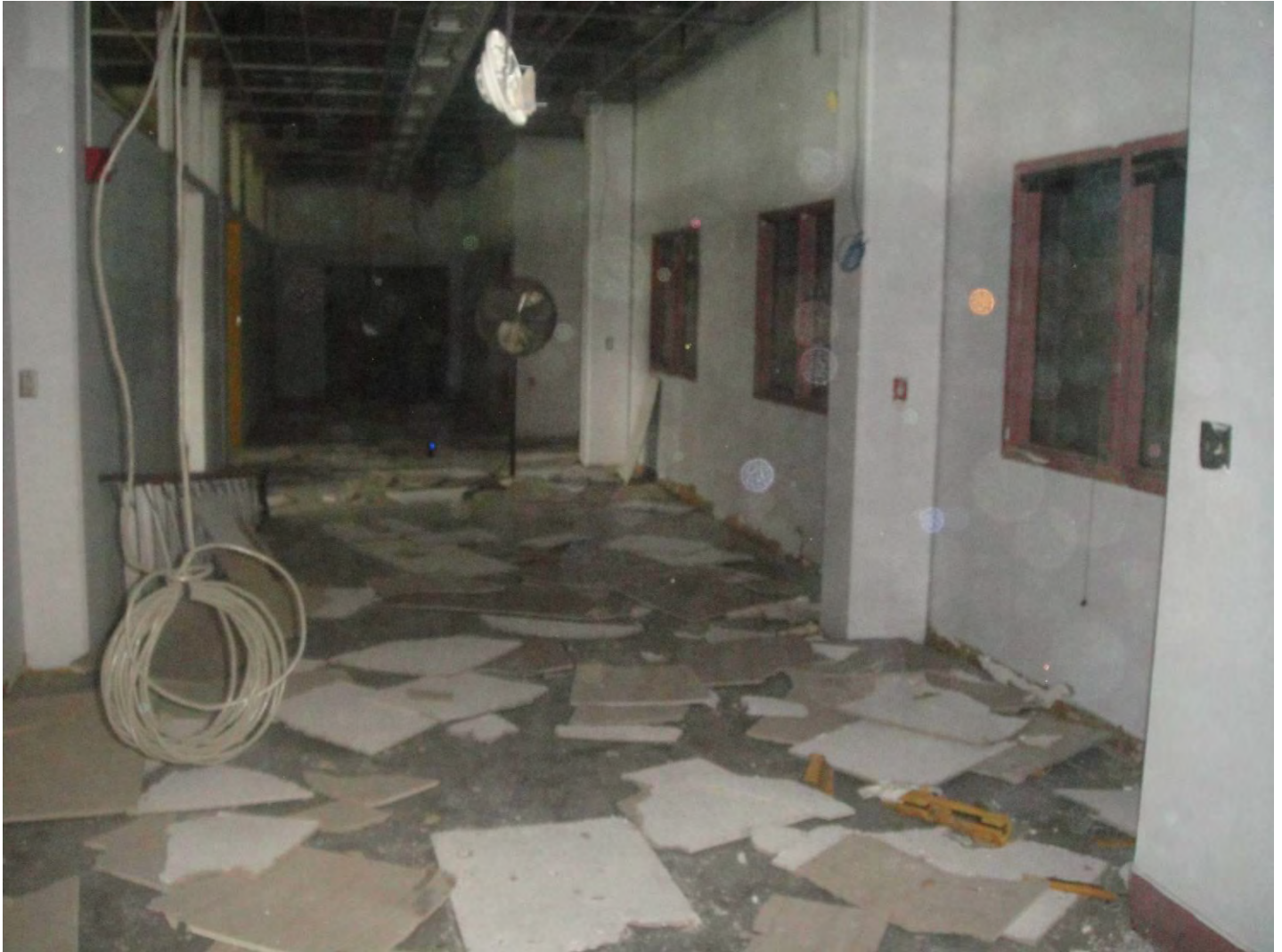
Photo 32 – Deteriorated Site Improvements.
