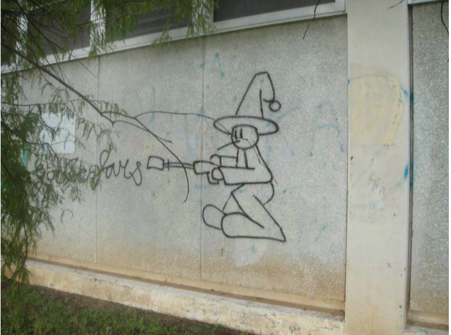
Photo 46 – Deteriorated Site Improvements.
