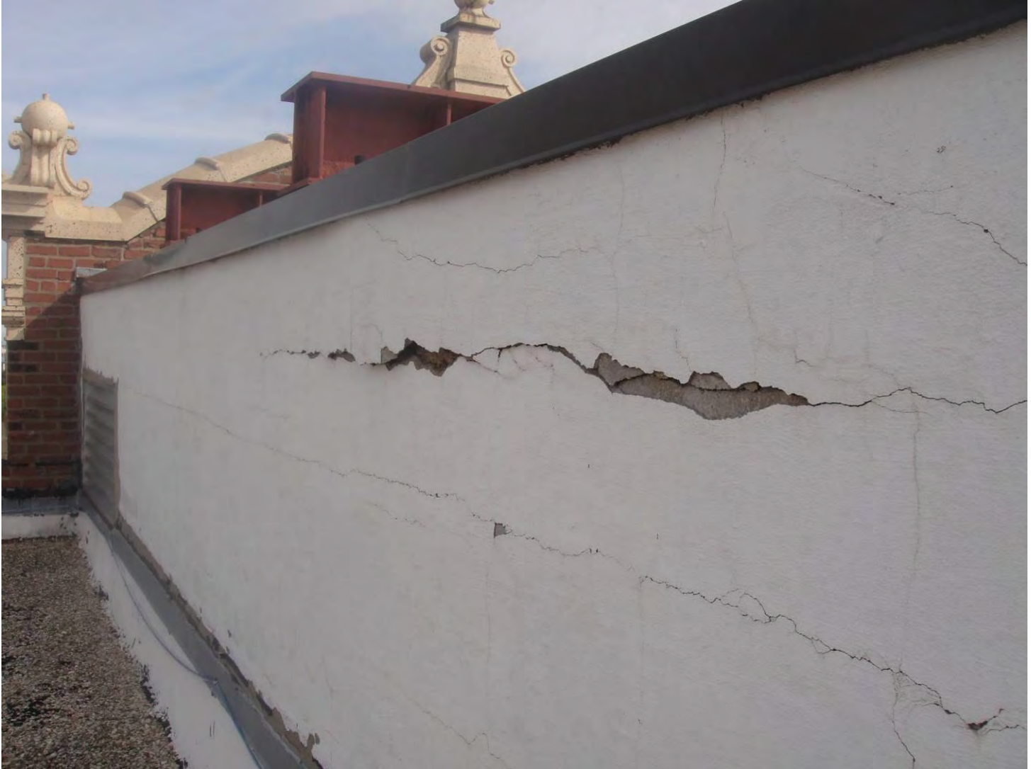
Photo 67 – Deteriorated Site Improvements.
