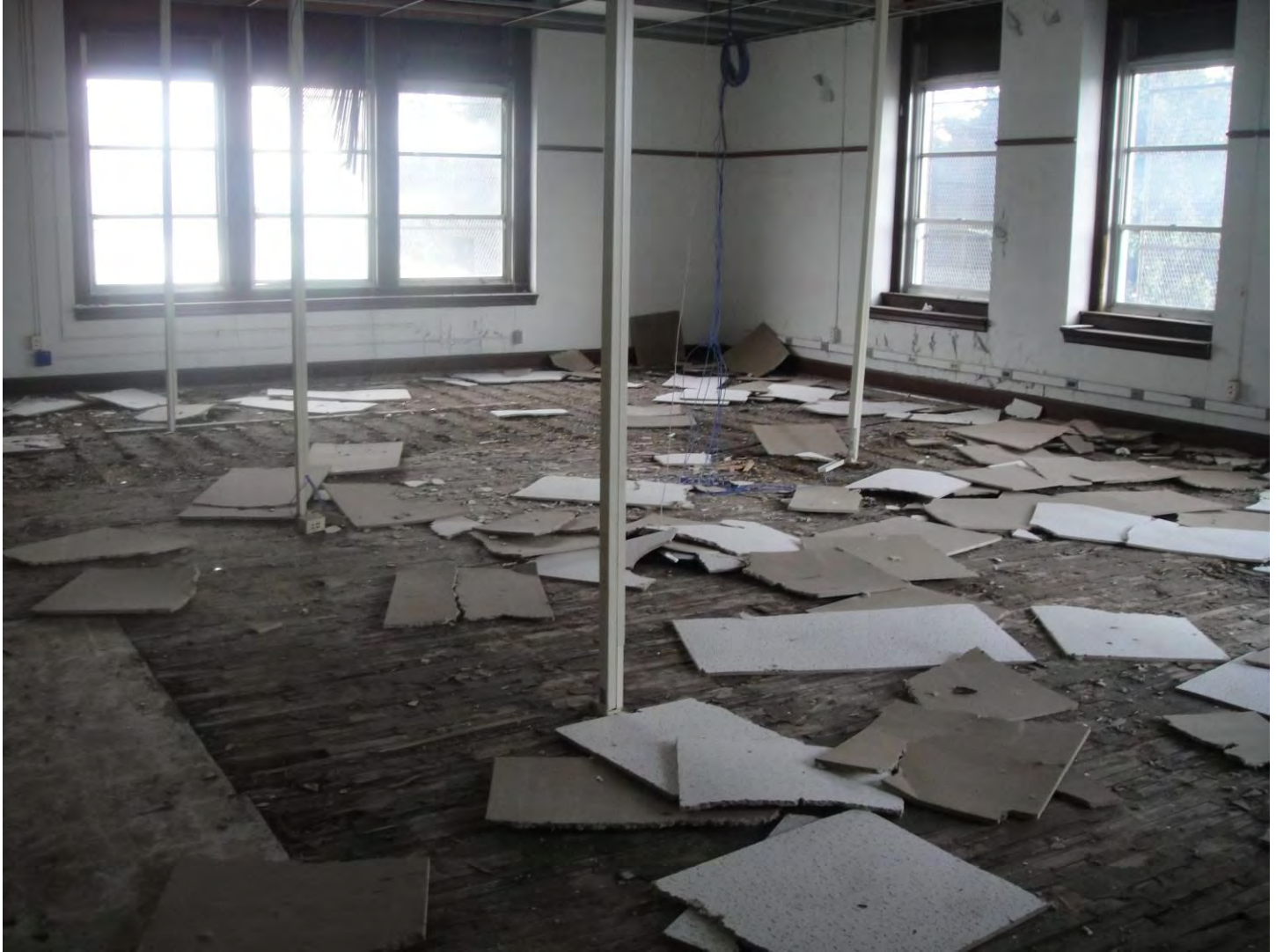
Photo 51 – Deteriorated Site Improvements.
