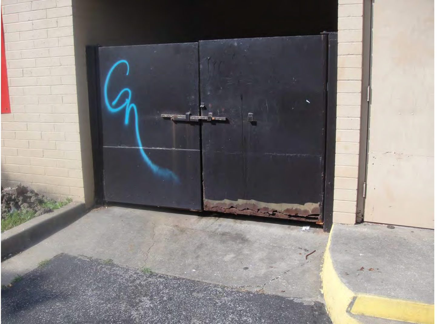
Photo 69 – Deteriorated Site Improvements.
