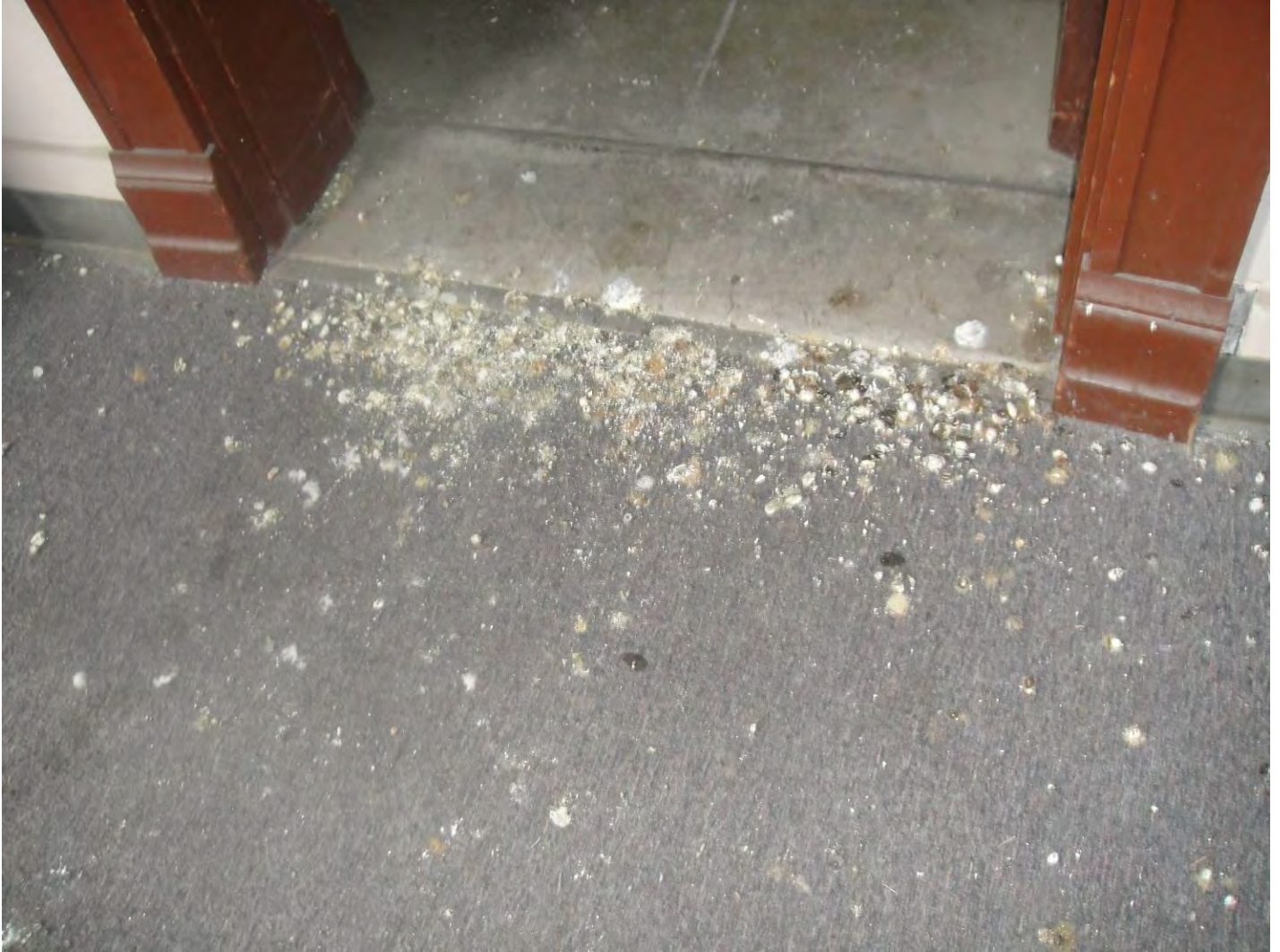
Photo 8 – Insanitary or unsafe conditions.
