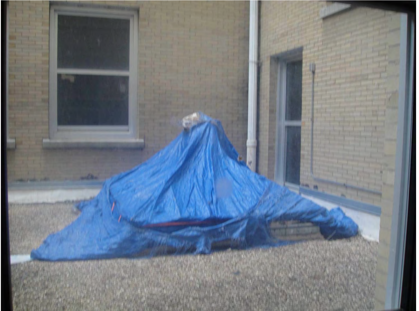
Photo 33 – Deteriorated Site Improvements.
