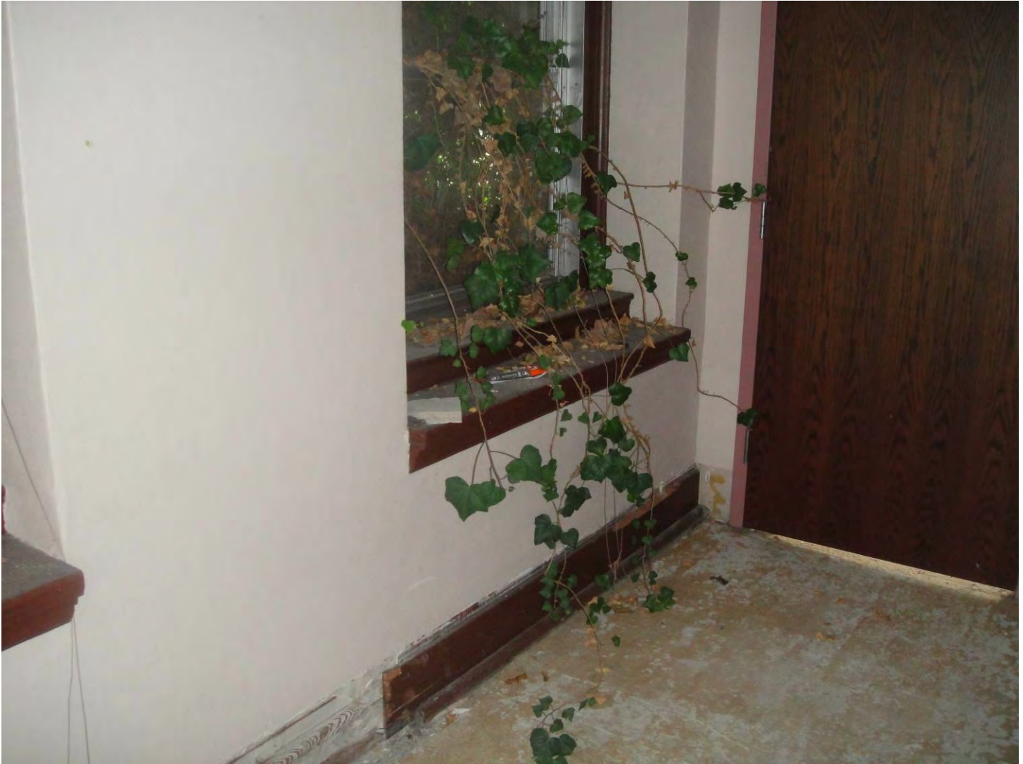
Photo 30 – Deteriorated Site Improvements.
