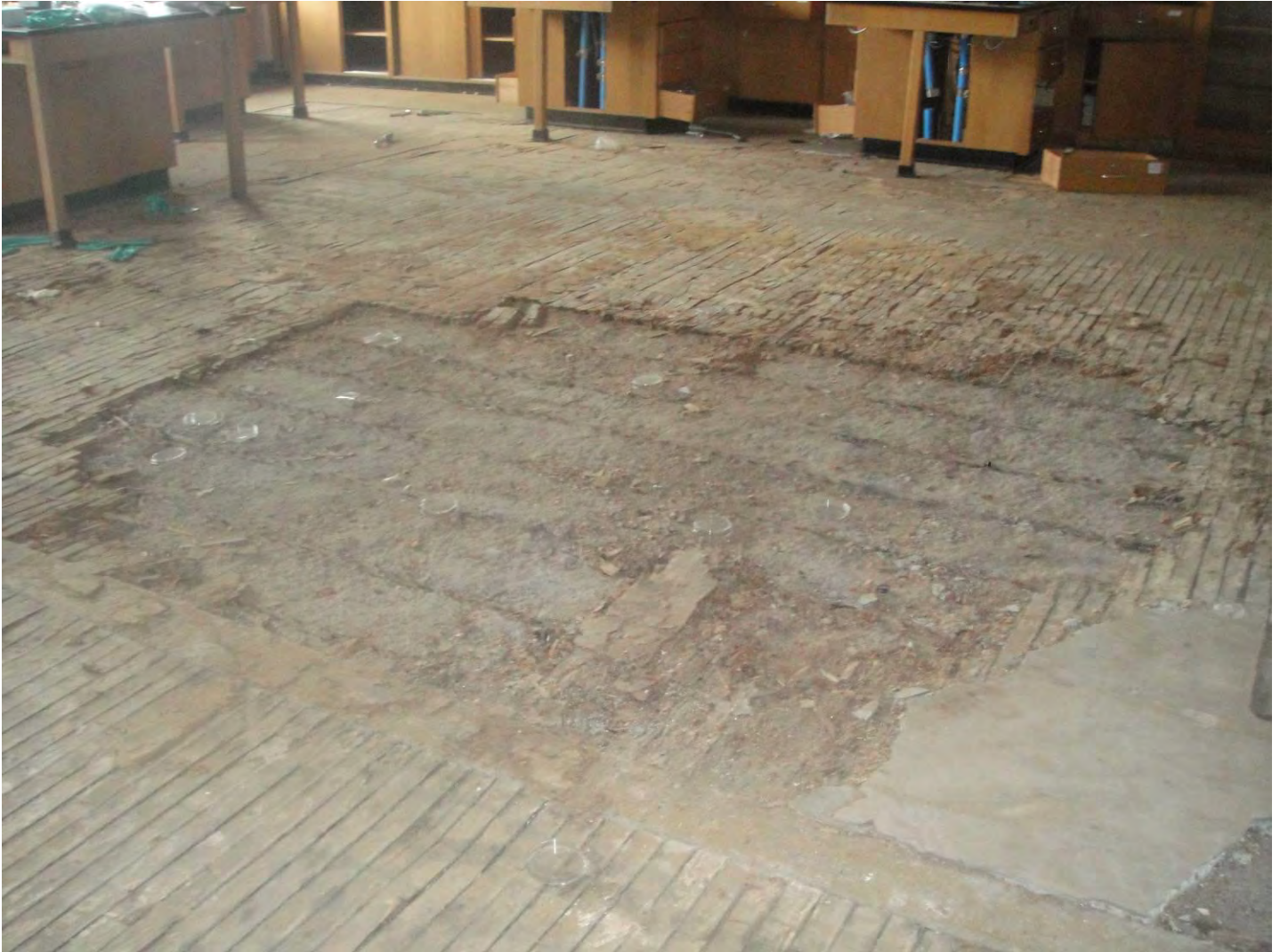
Photo 40 – Deteriorated Site Improvements.
