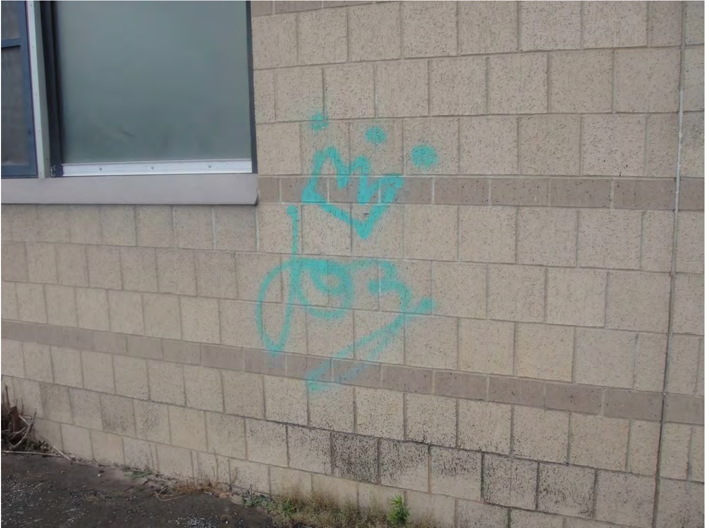
Photo 19 – Deteriorated Site Improvements.
