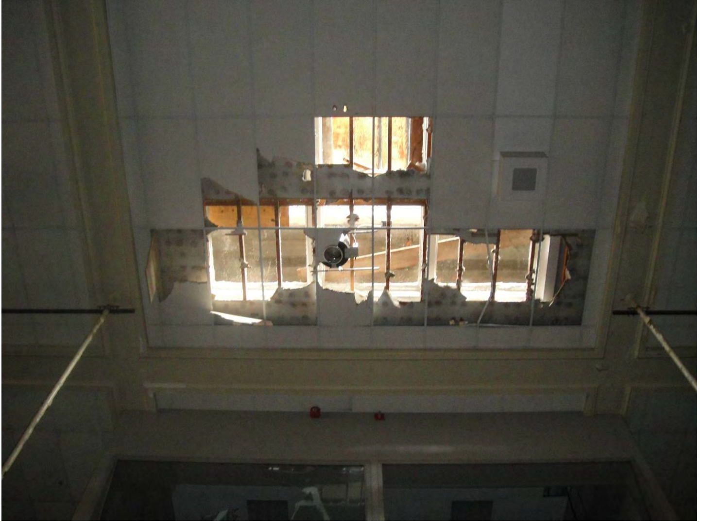
Photo 42 – Deteriorated Site Improvements.
