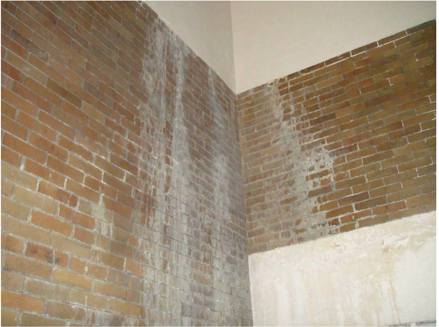
Photo 61 – Deteriorated Site Improvements.
