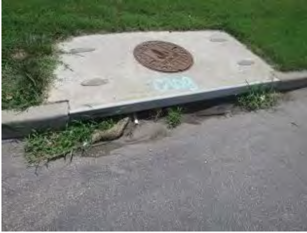
Clogged Sewer Inlet Along Swope Parkway
