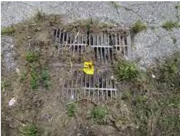
Clogged Sewer Inlet At 2801 Swope Parkway
