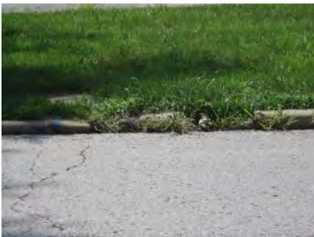
Deteriorated Curbs Along Agnes Avenue
