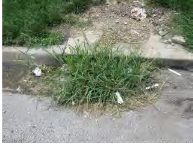
Clogged Sewer Inlet Along Chestnut Avenue
