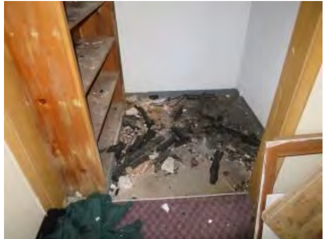
Interior Fire At 2801 Swope Parkway
