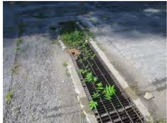
Clogged Drainage Grate At 2915 Swope Parkway
