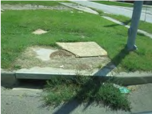
Clogged Sewer Inlet Along Swope Parkway
