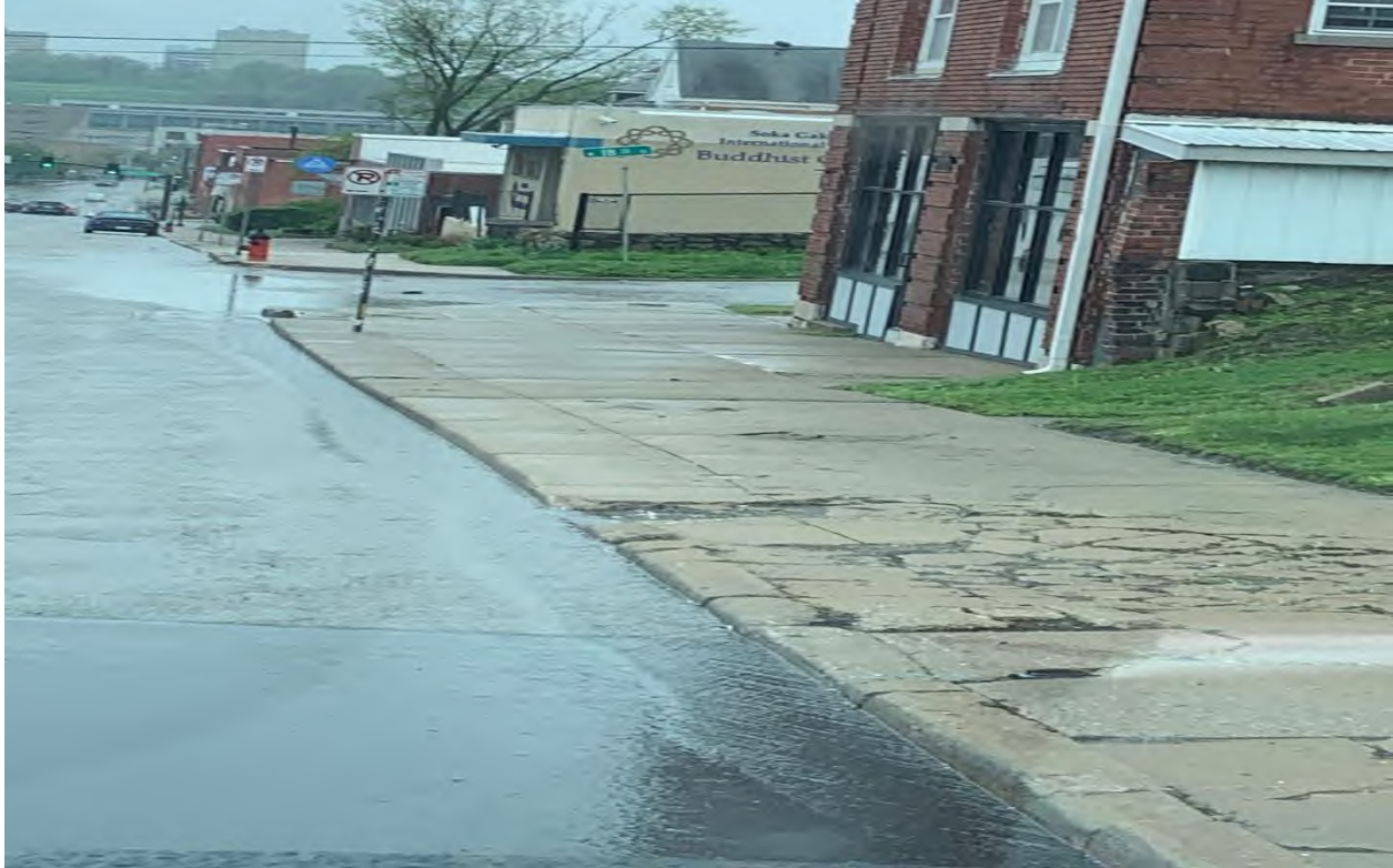
Figure 4. 18th Street and Broadway Blvd. Standing water, unable to drain.
