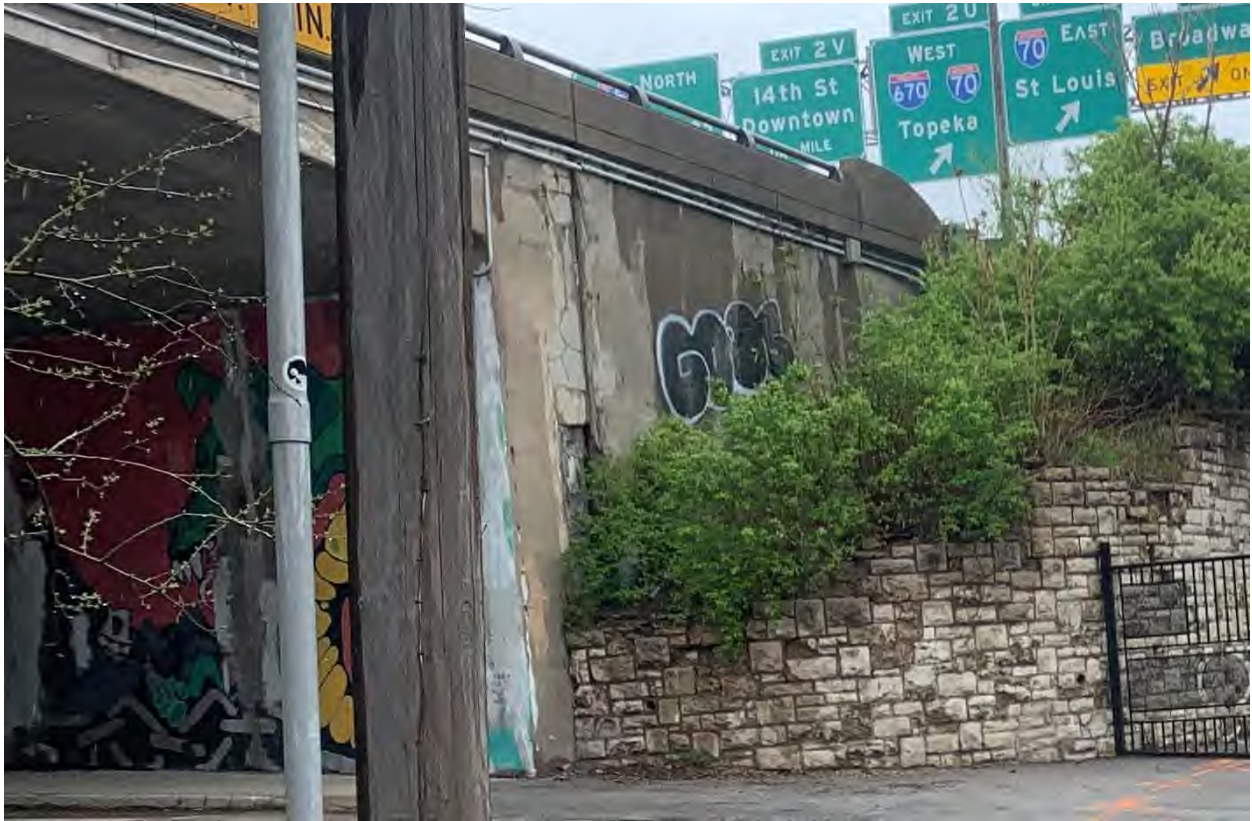
Figure 11. Freeway bridge on north side of 17th St. west of Washington. Graffiti.
