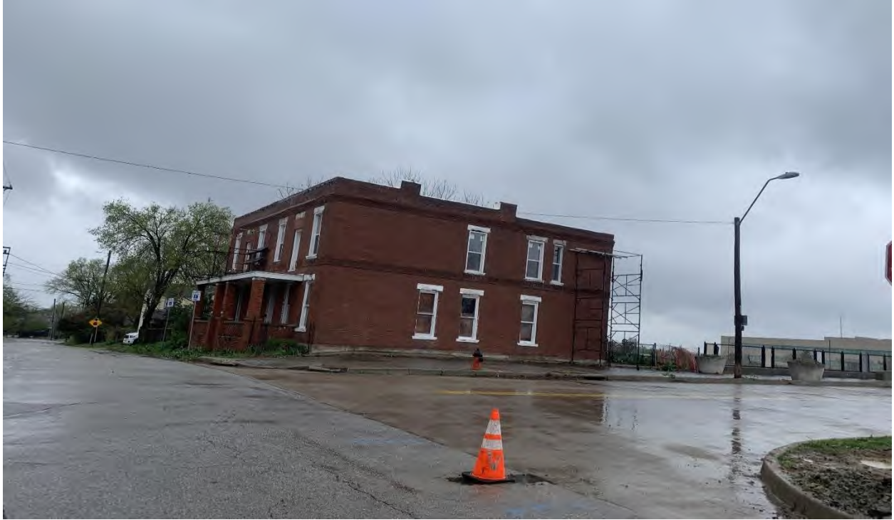
Figure 7. 802 W. 16th St. view from the east, unprotected scaffolding.
