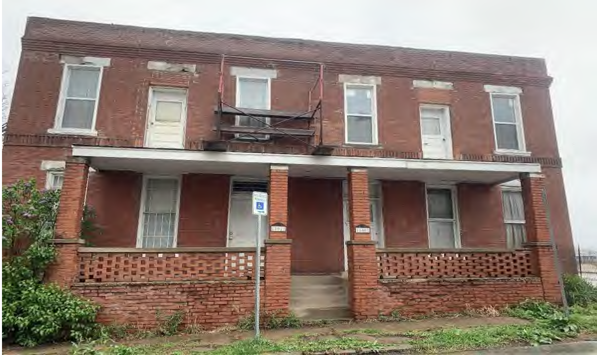
Figure 5. 802 W. 16th St. House in disrepair.
