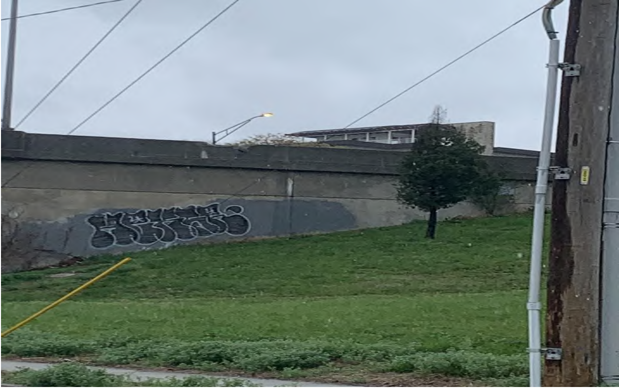
Figure 13. 20th and Washington. Graffiti on freeway wall
