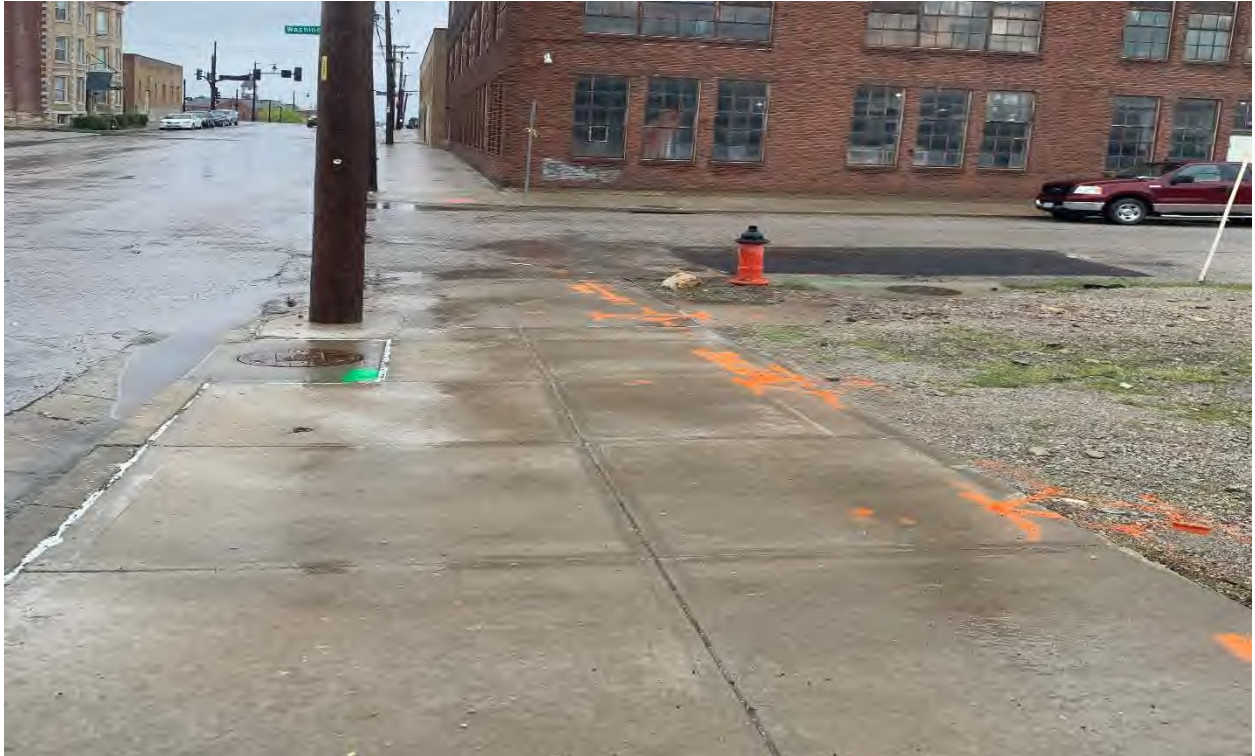
Figure 5. Southwest corner of Washington and 17th Street. Standing water at drain.
