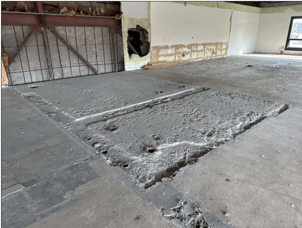
100 E. 20 th Street – interior – uneven floor
