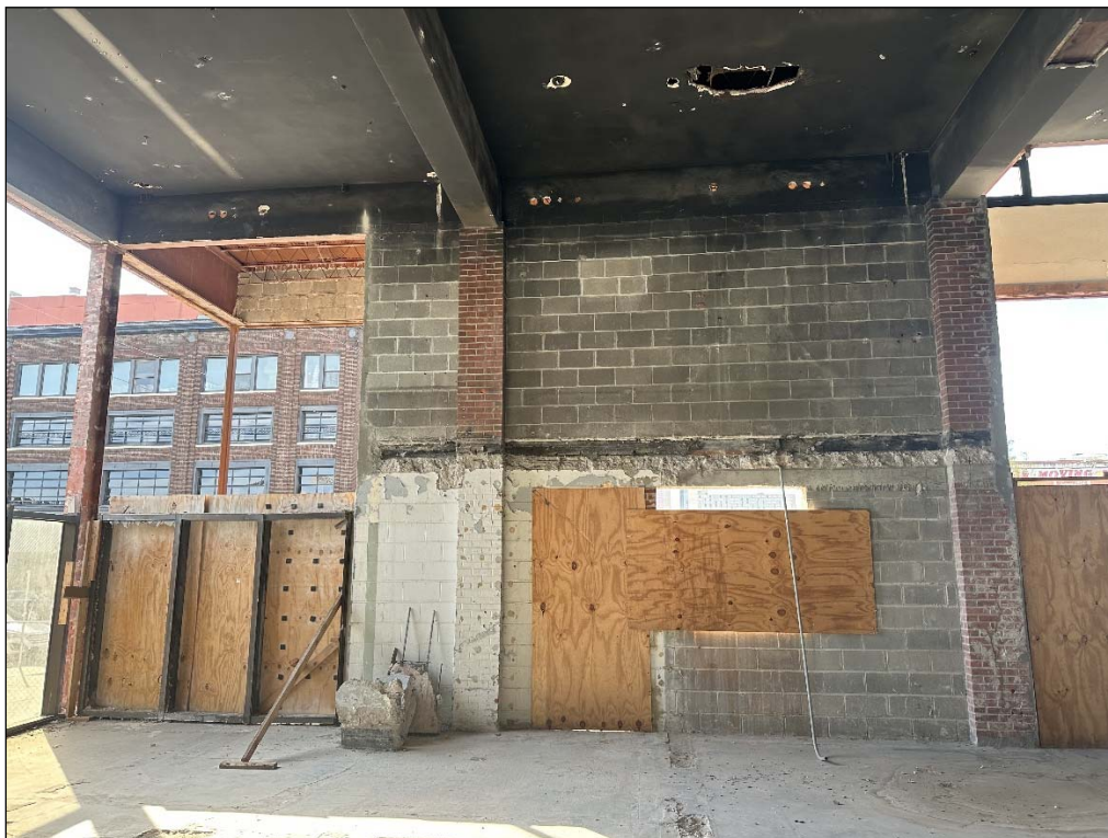
100 E. 20 th Street – interior – deterioration/damage of wall, interior finishes
