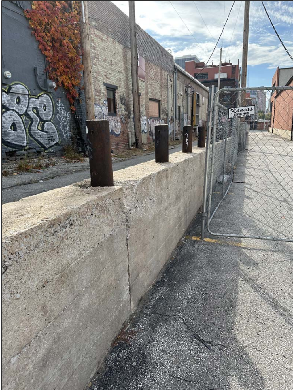
100 E. 20 th Street – looking south – deterioration of retaining wall
