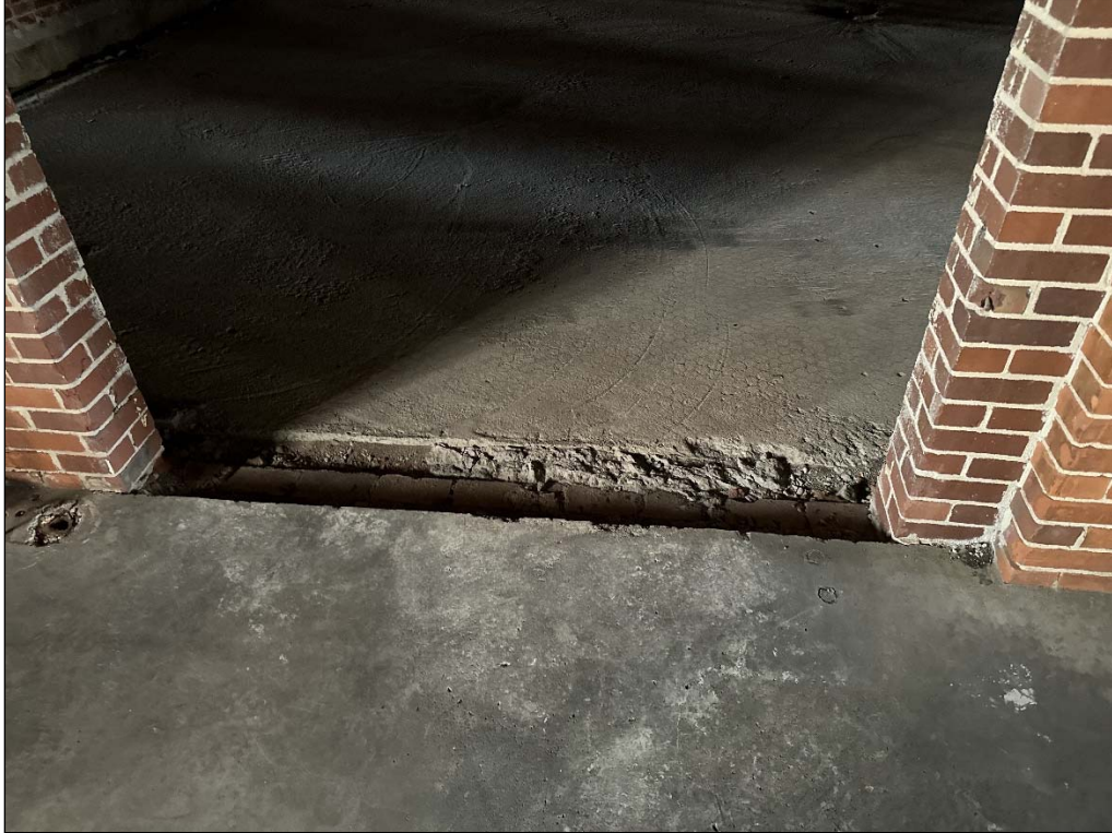
1905 Walnut Street – interior – uneven floor
