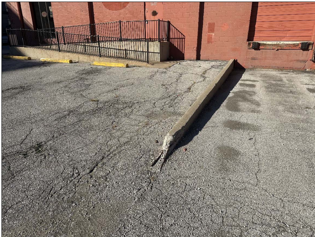
100 E. 20 th Street – looking north – deterioration of pavement
