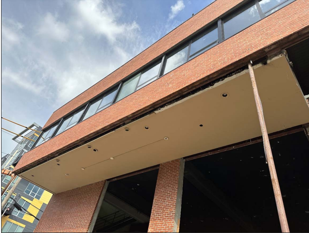
100 E. 20 th Street – looking north – deterioration/damage of interior finishes
