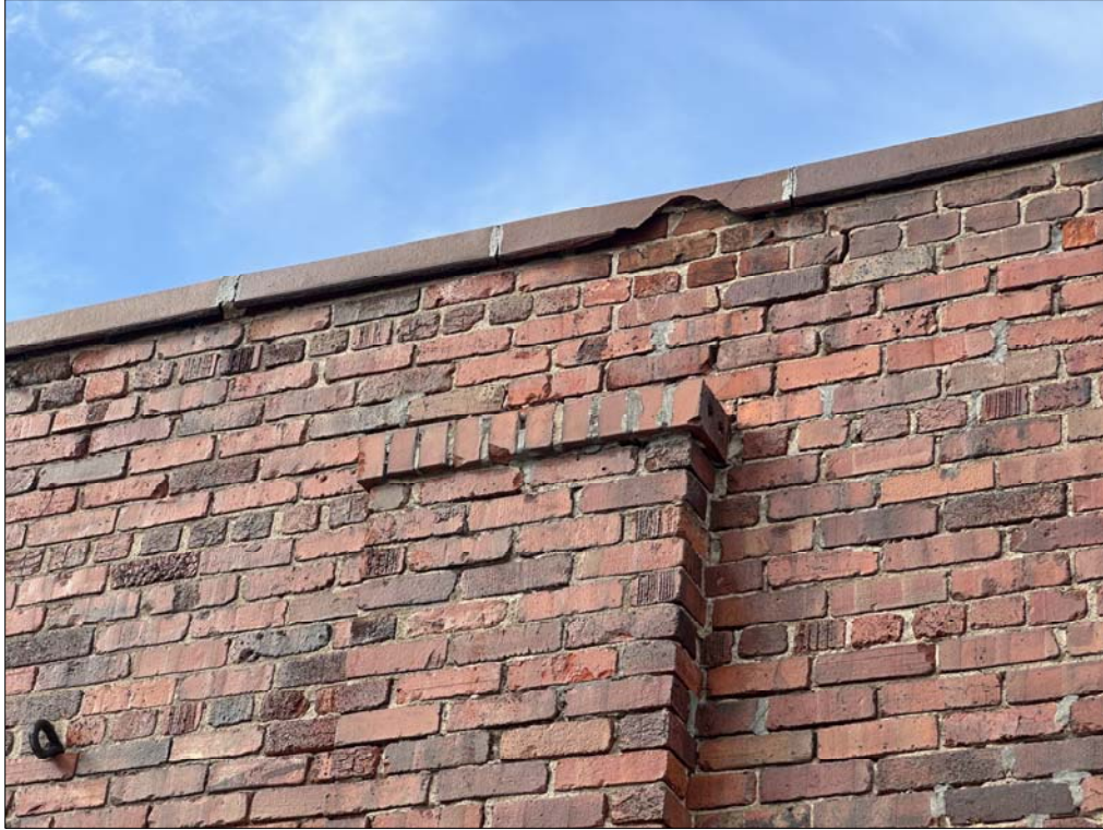
1905 Walnut Street – looking west – deterioration of masonry joints, roof coping
