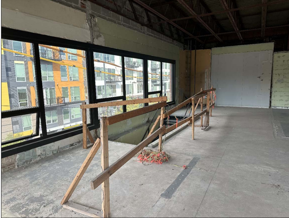
100 E. 20 th Street – interior – inadequate guardrails around floor opening
