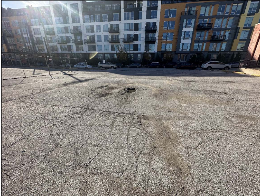
100 E. 20 th Street – looking west – deterioration of pavement
