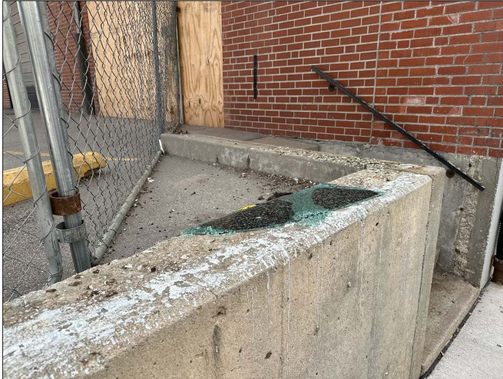
100 E. 20 th Street – looking southeast – broken glass (trash/debris) on retaining wall
