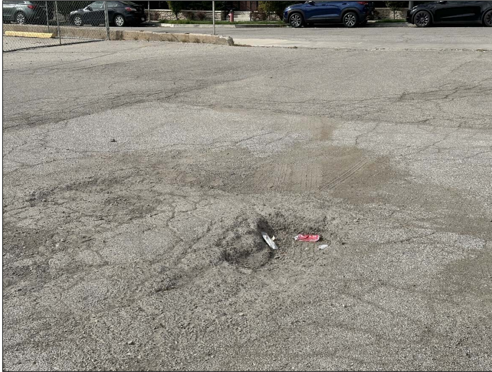
1905 Walnut Street – looking southwest – uneven pavement
