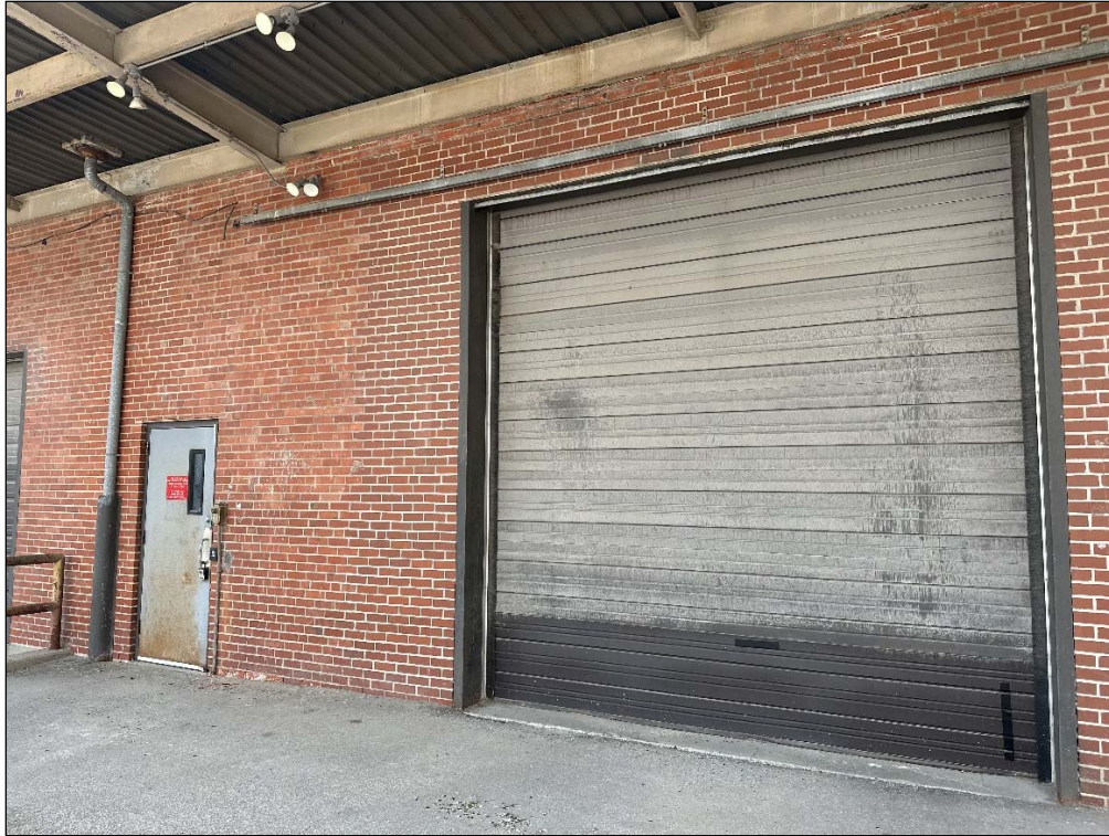
100 E. 20 th Street – looking south – deterioration of doors
