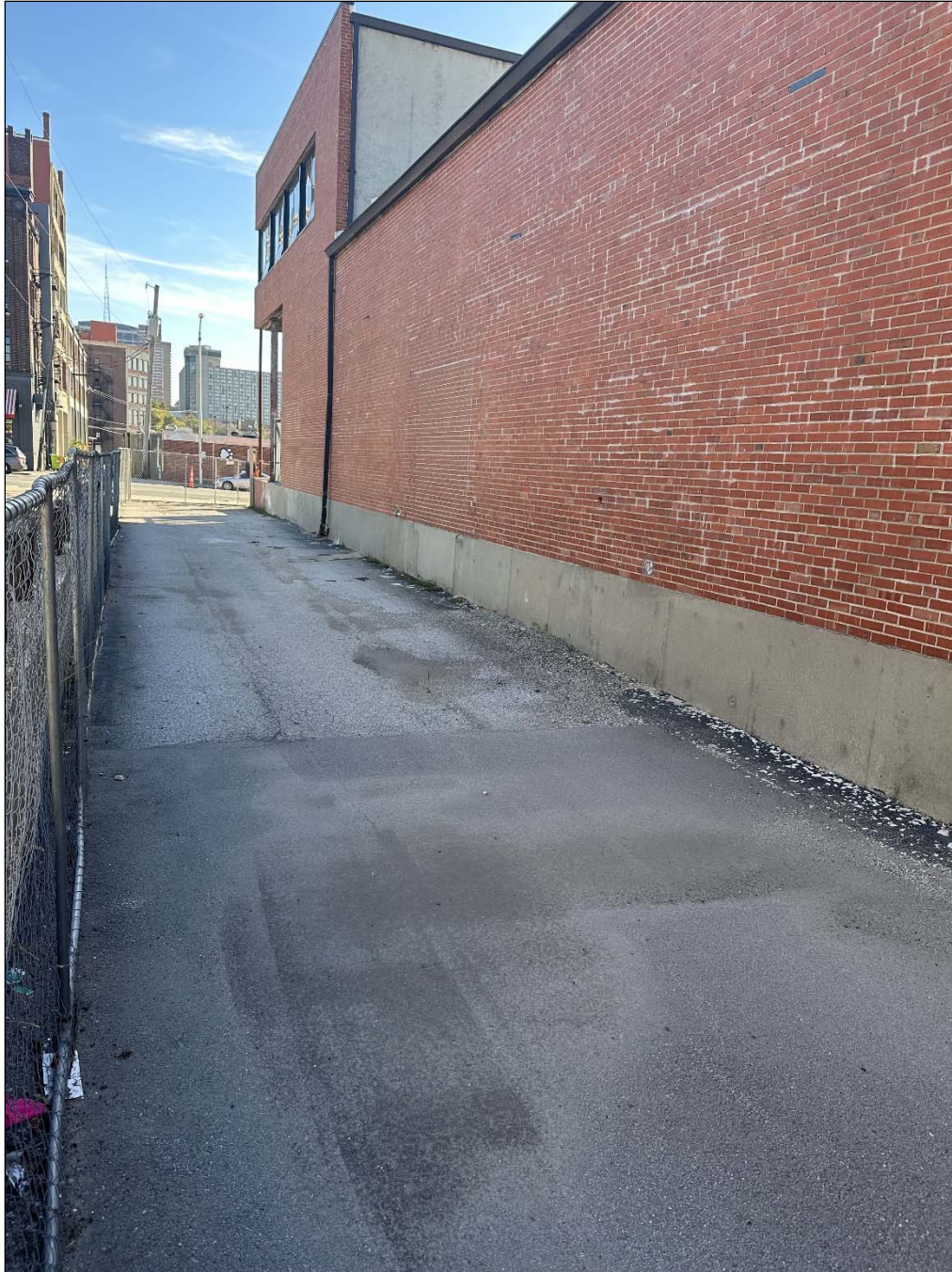
100 E. 20 th Street – looking south – deterioration of pavement
