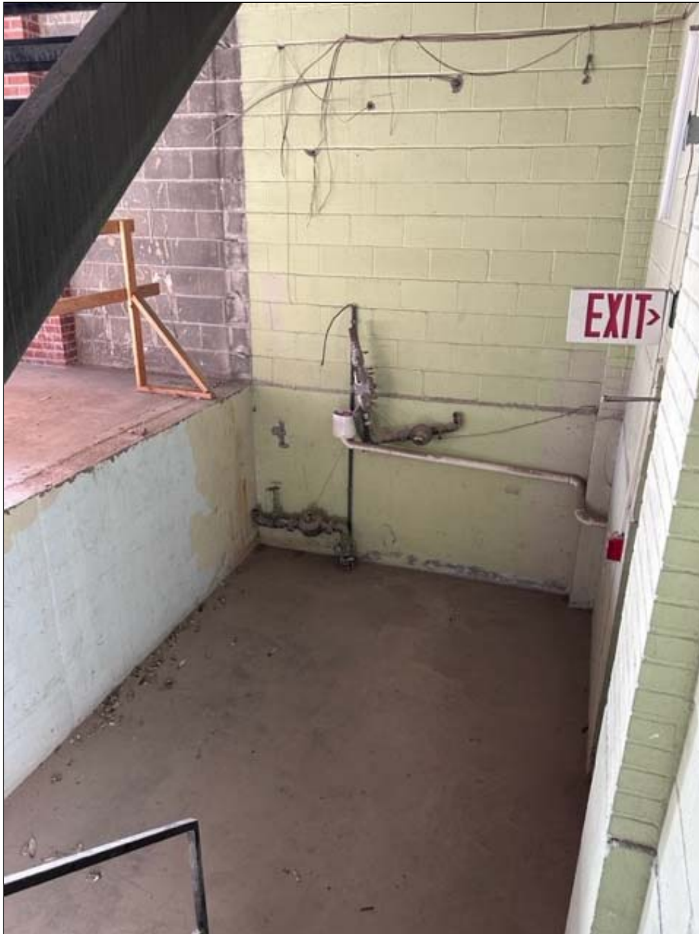
100 E. 20 th Street – interior – disconnected building systems
