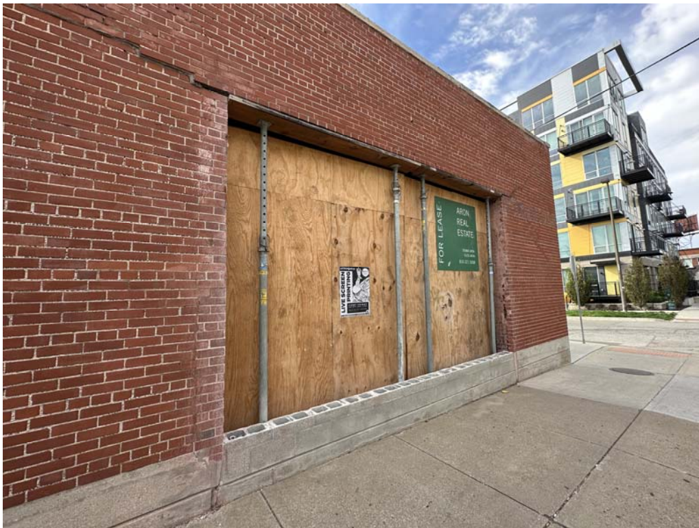
1905 Walnut Street – looking southwest – cracking, shifting of masonry
