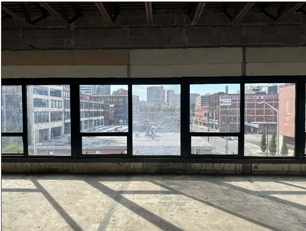
100 E. 20 th Street – interior – shattered window
