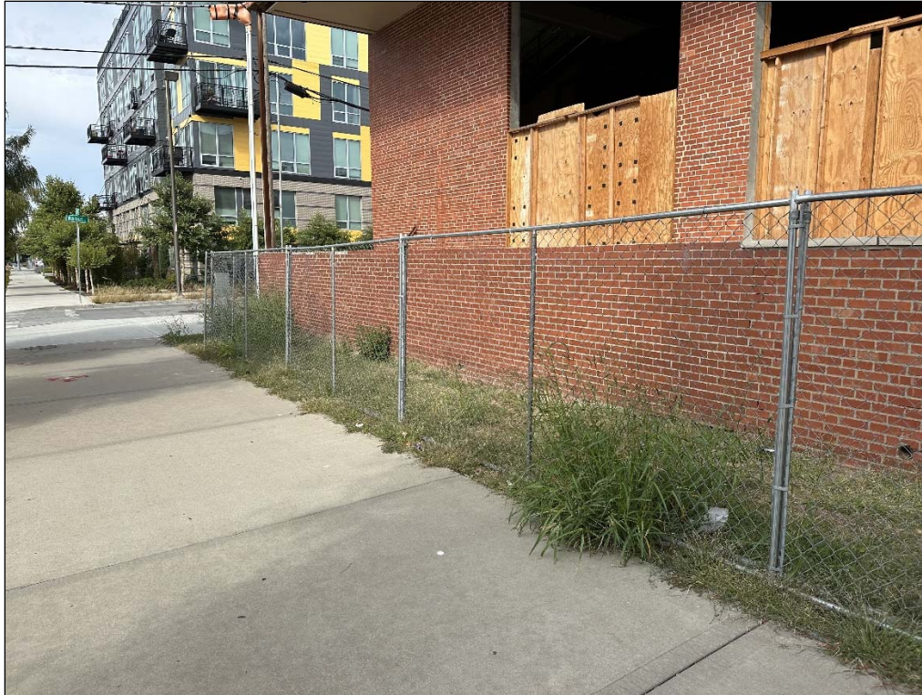
100 E. 20 th Street – looking west – overgrown vegetation along sidewalk
