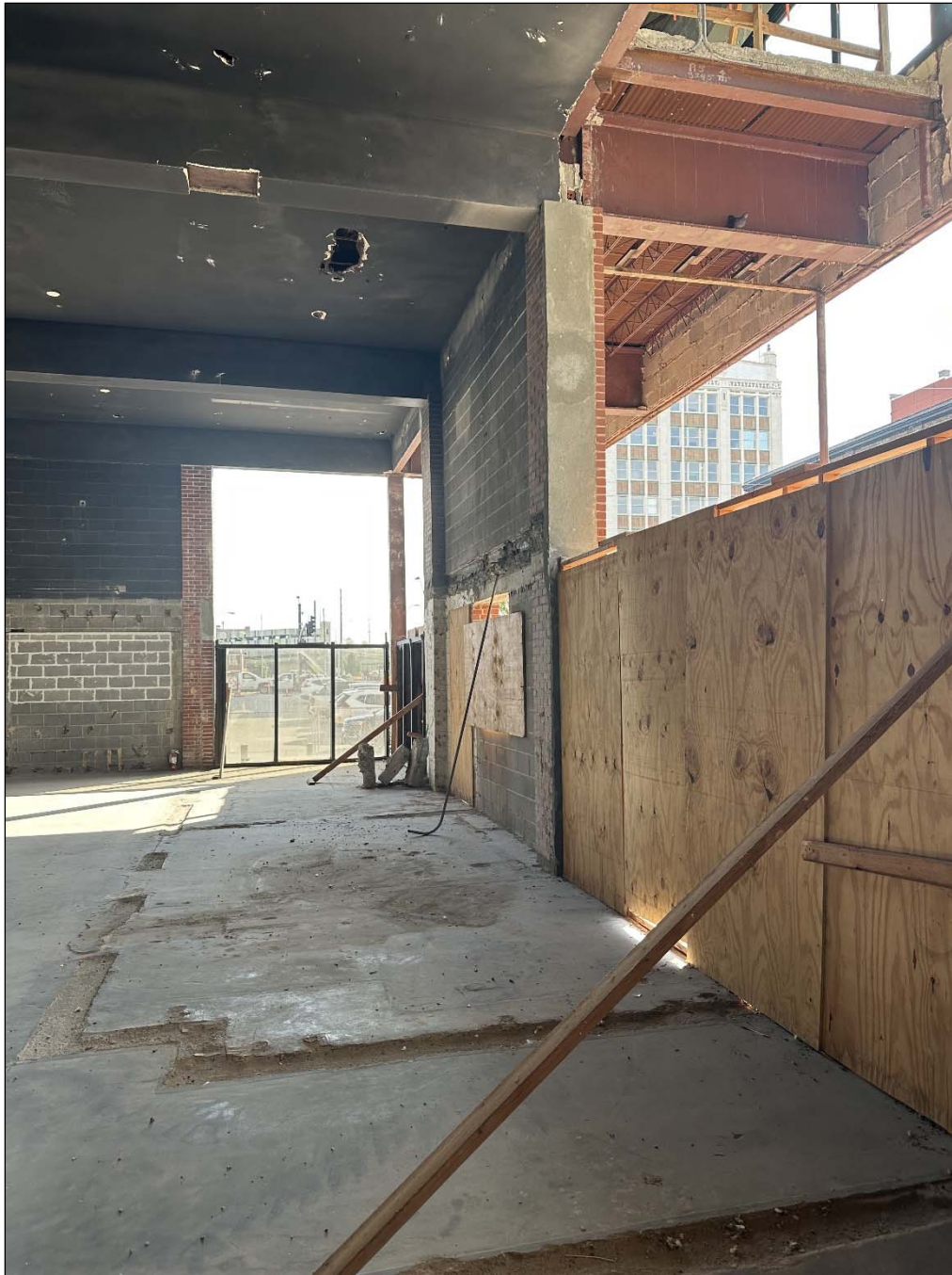
100 E. 20 th Street – interior – uneven floor; open building (lack of windows, doors)
