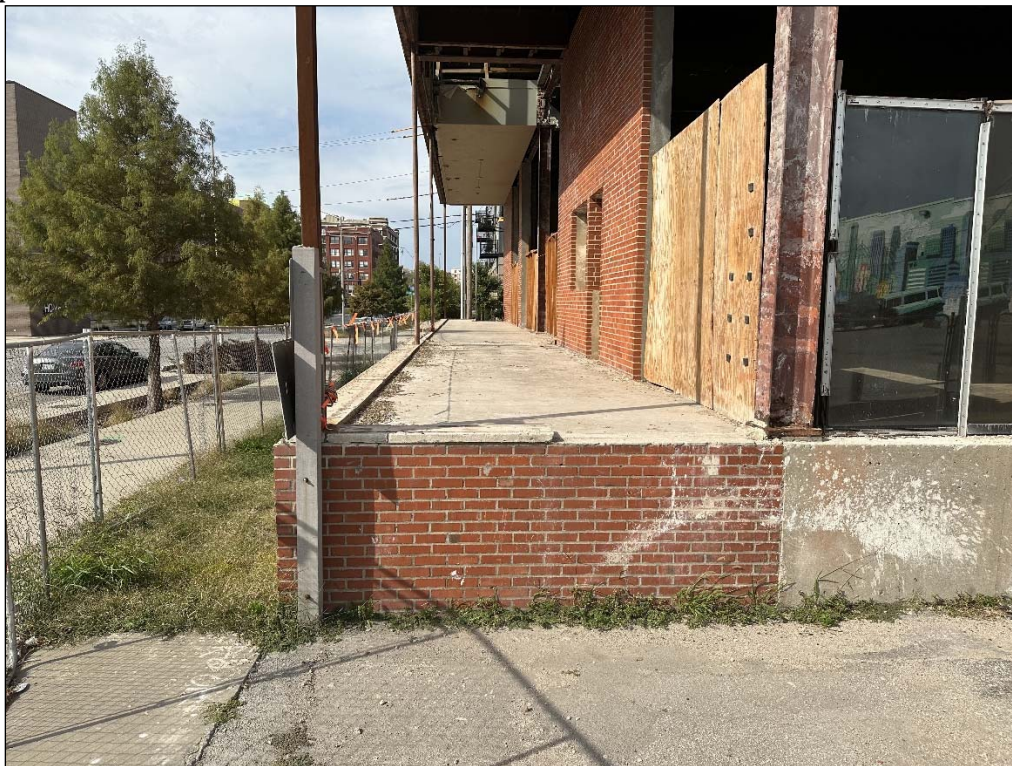
100 E. 20 th Street – looking west – no warning line/guardrail at perimeter of porch
