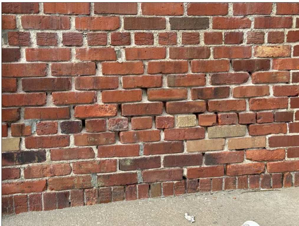
1905 Walnut Street – looking west – deterioration of masonry joints
