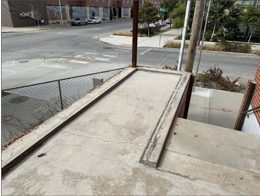
100 E. 20 th Street – looking west – accessible stair to property; no warning line/guardrail at perimeter of porch
