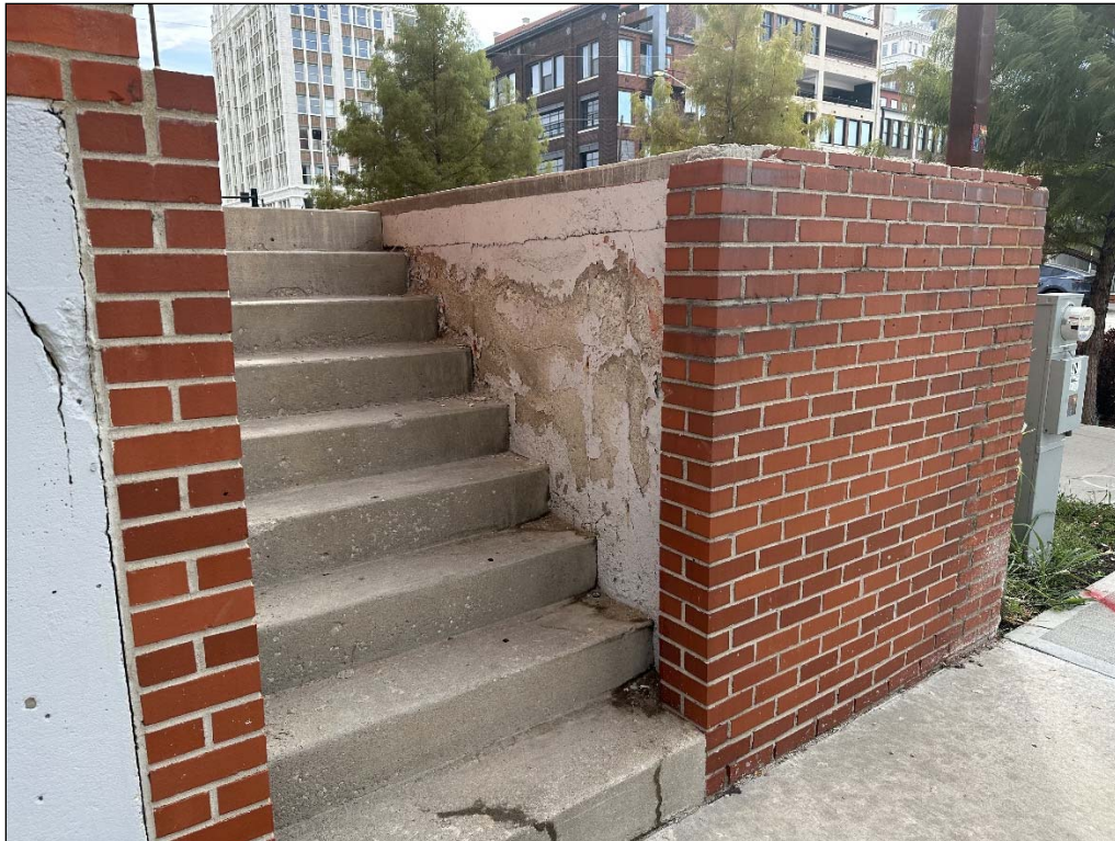
100 E. 20 th Street – looking southeast – deterioration of wall
