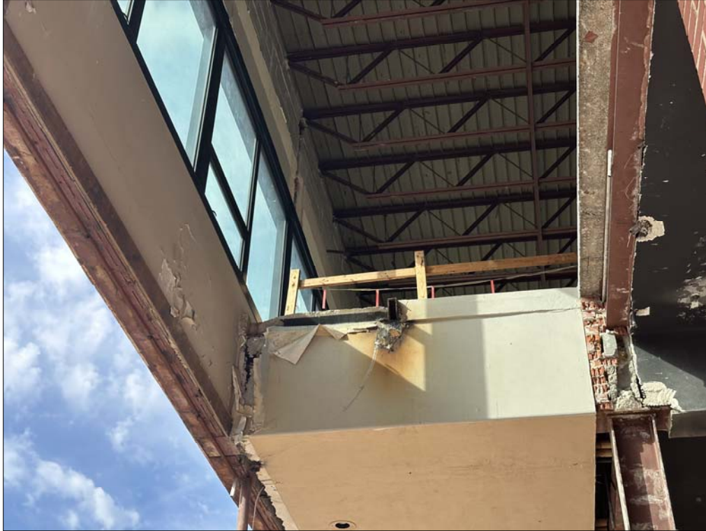
100 E. 20 th Street – interior – deterioration/damage of interior finishes
