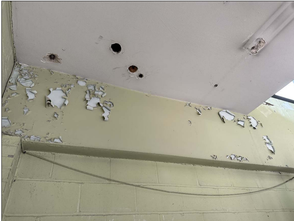
100 E. 20 th Street – interior – failure of finishes
