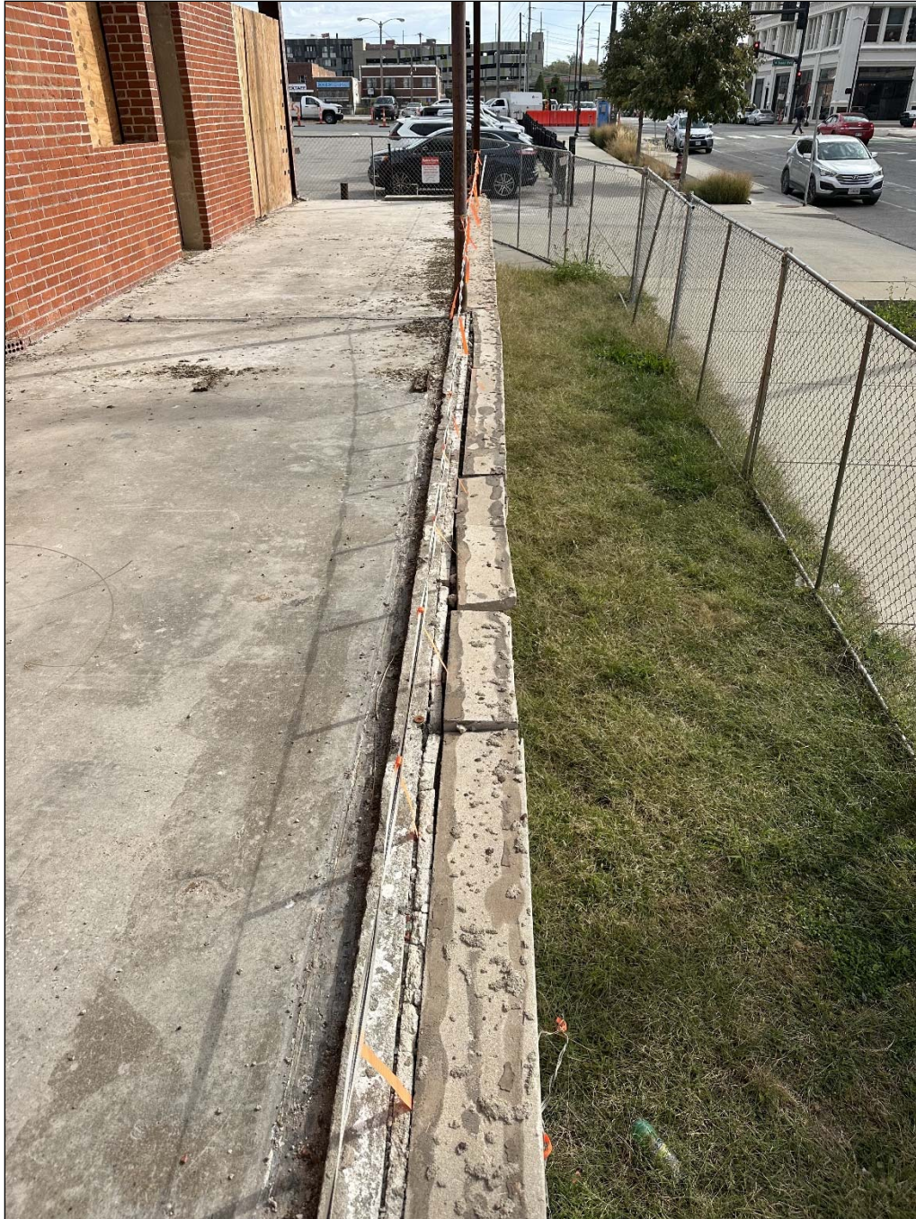
100 E. 20 th Street – looking east – deteriorationn of wall
