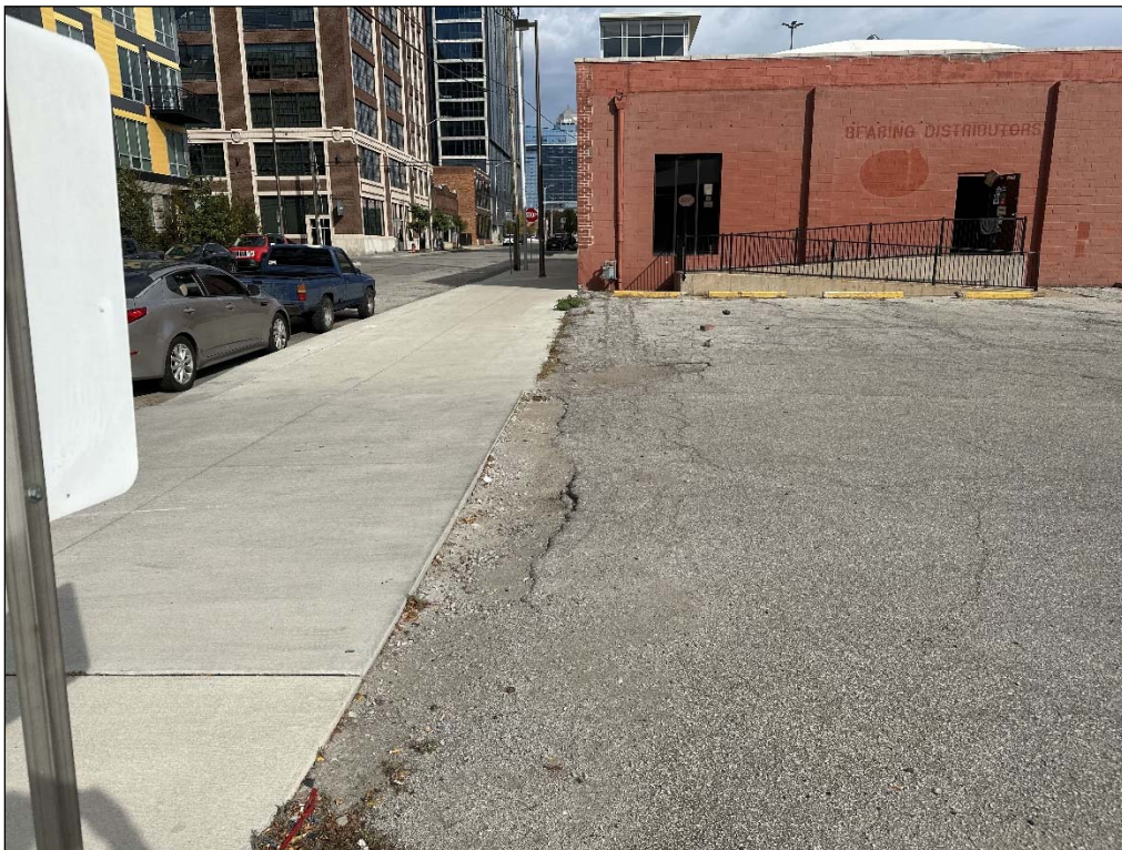
1905 Walnut Street – looking north – uneven pavement
