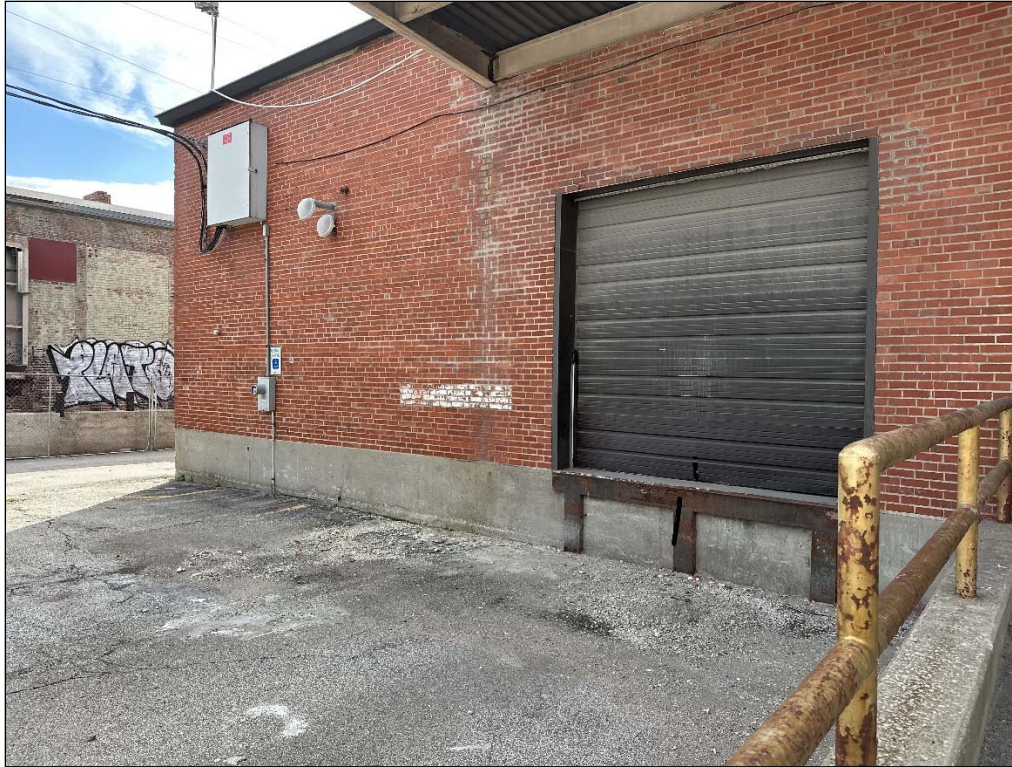
100 E. 20 th Street – looking southeast – deterioration of pavement, dock area
