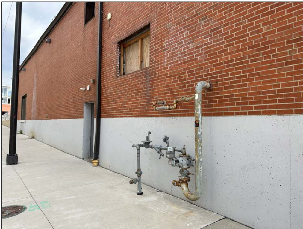
100 E. 20 th Street – looking east – failure of finishes on equipment
