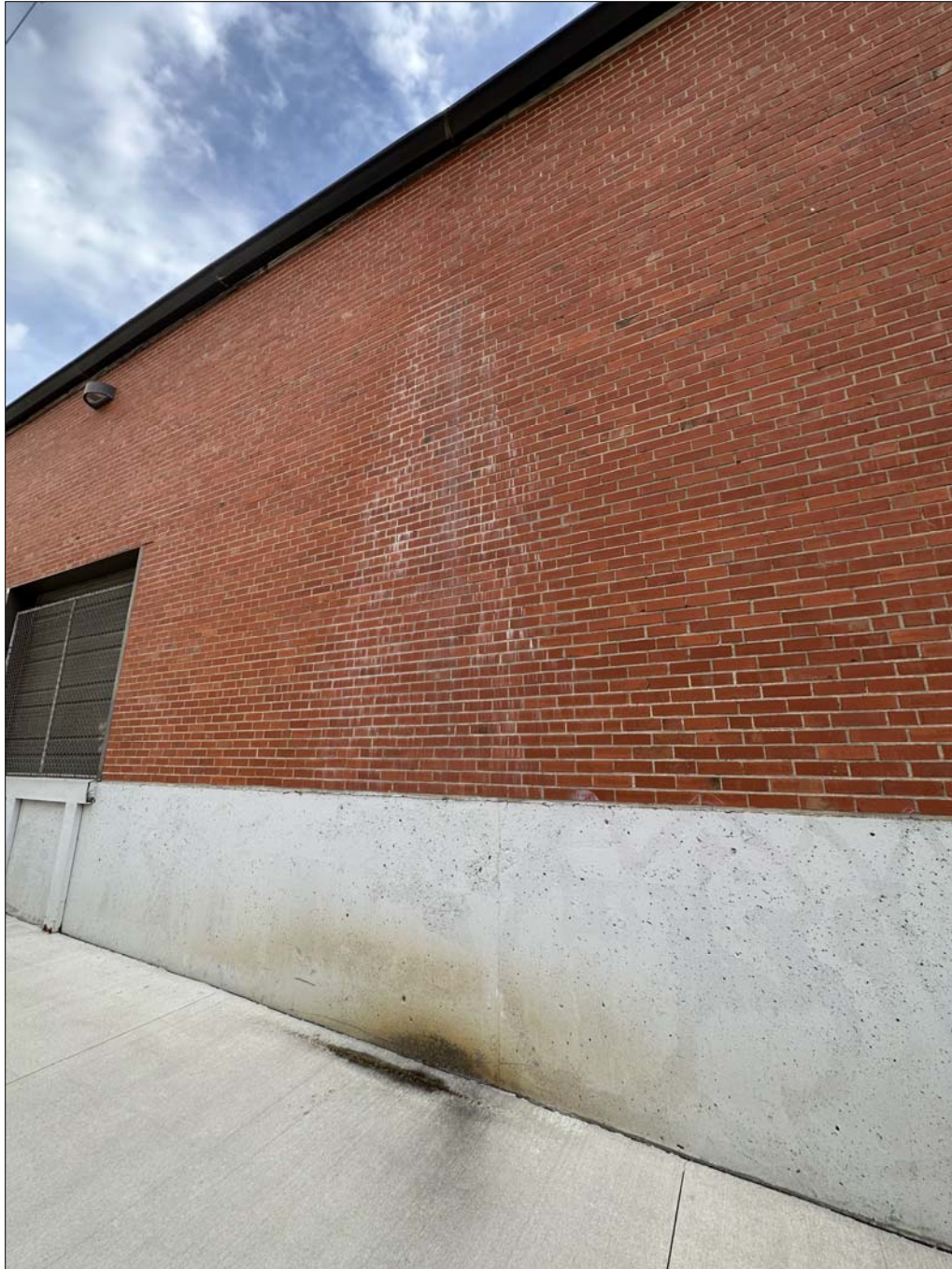
100 E. 20 th Street – looking east – deterioration of gutter, water damage
