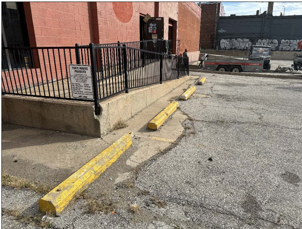
1905 Walnut Street – looking east – deterioration of pavement, wall
