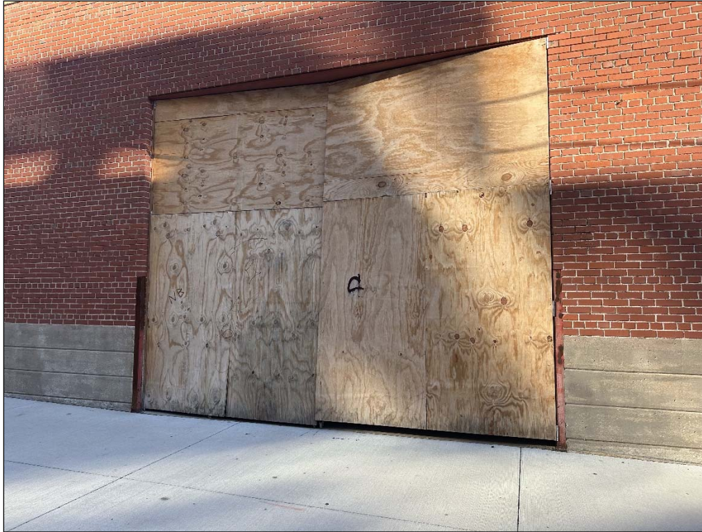
1905 Walnut Street – looking east – lack of building enclosure (windows/doors)
