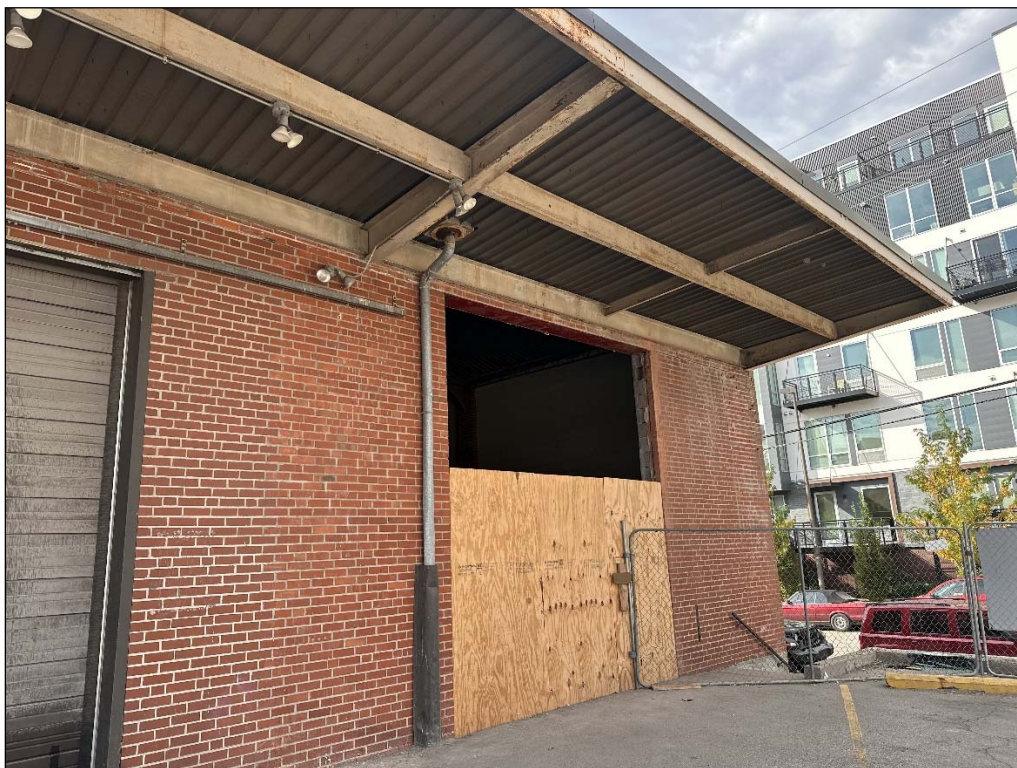
100 E. 20 th Street – looking southwest – failure of finishes on canopy structure
