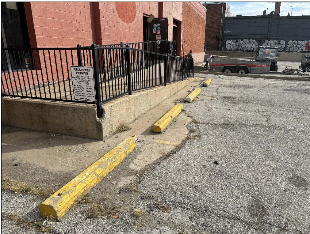
1905 Walnut Street – looking east – uneven pavement; lack of handrails for ramp; narrow ramp
