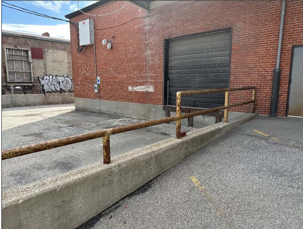
100 E. 20 th Street – looking southeast – failure of finishes on railing
