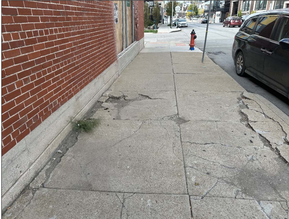
1905 Walnut Street – looking west – deteriorated sidewalk
