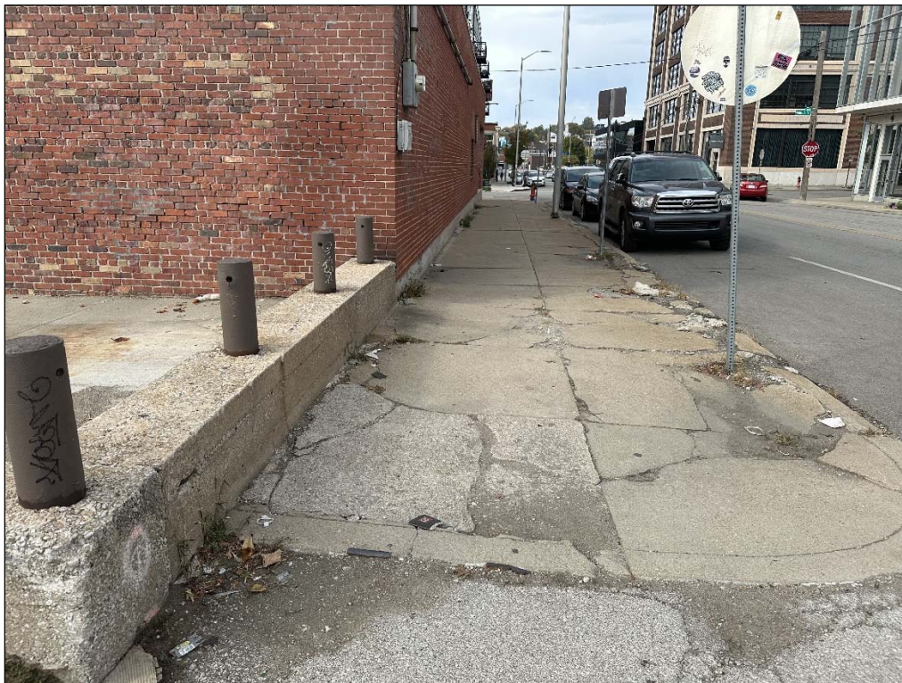
1905 Walnut Street – looking west – deteriorated sidewalk
