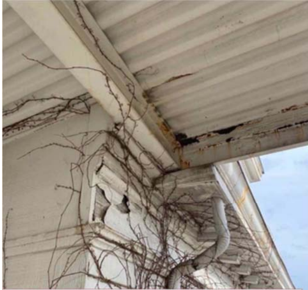
Building 1200 third-floor balcony has wood rot on exterior trim above doorway & multiple locations
