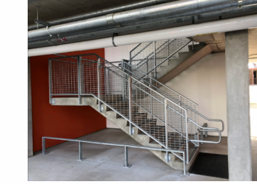
GALVANIZED STEEL GUARDRAIL WITH MESH INFILL
