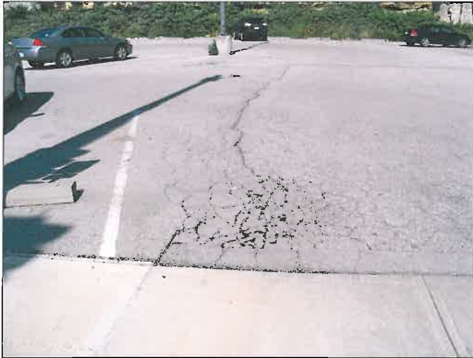
1514 Baltimore Avenue – looking west – deterioration of surface parking lot
