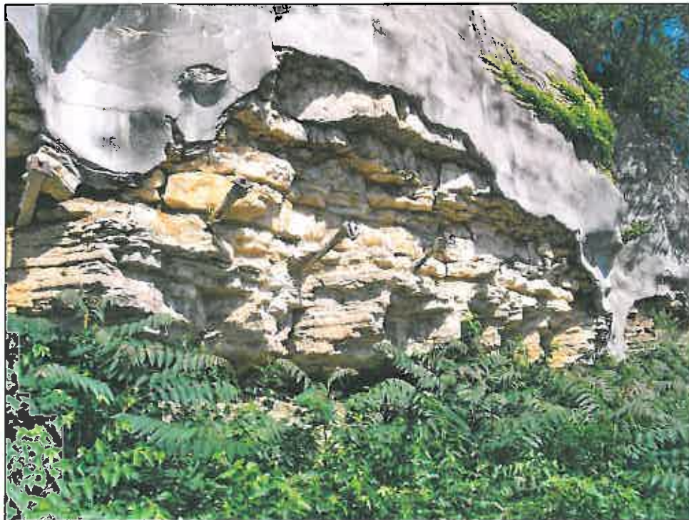
1514 Baltimore Avenue – looking west – deterioration of gunite and rock wall; deterioration of steel ties; overgrown vegetation
