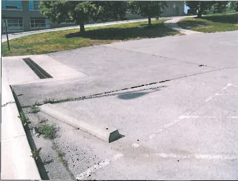
1514 Baltimore Avenue – unsafe parking stall due to slope of pavement for drainage
