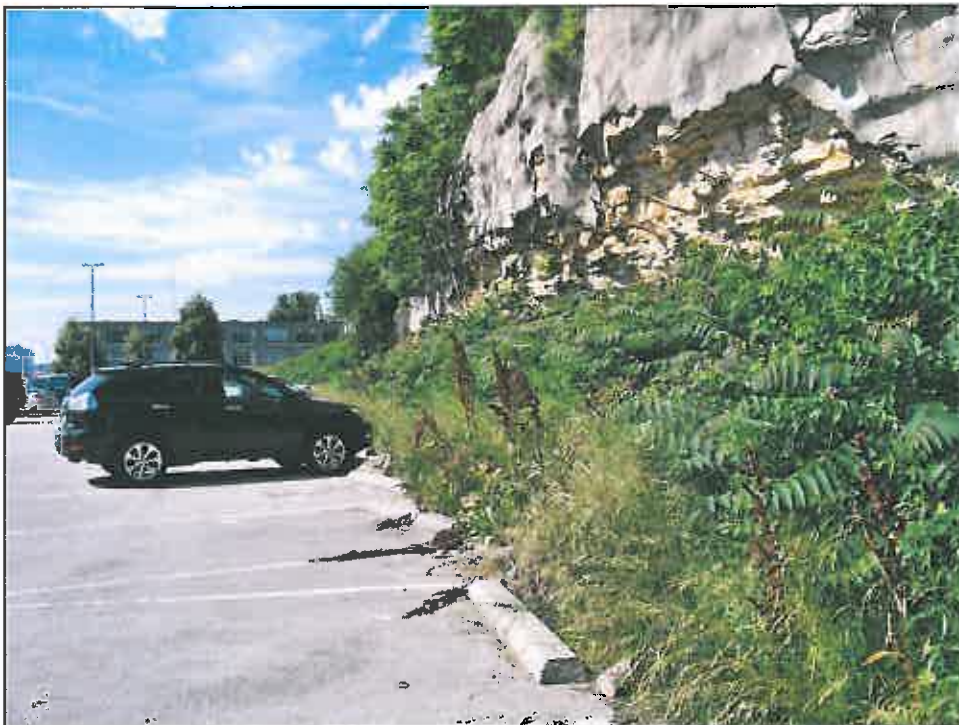
1514 Baltimore Avenue – looking south – overgrown vegetation; falling rock; trash/debris
