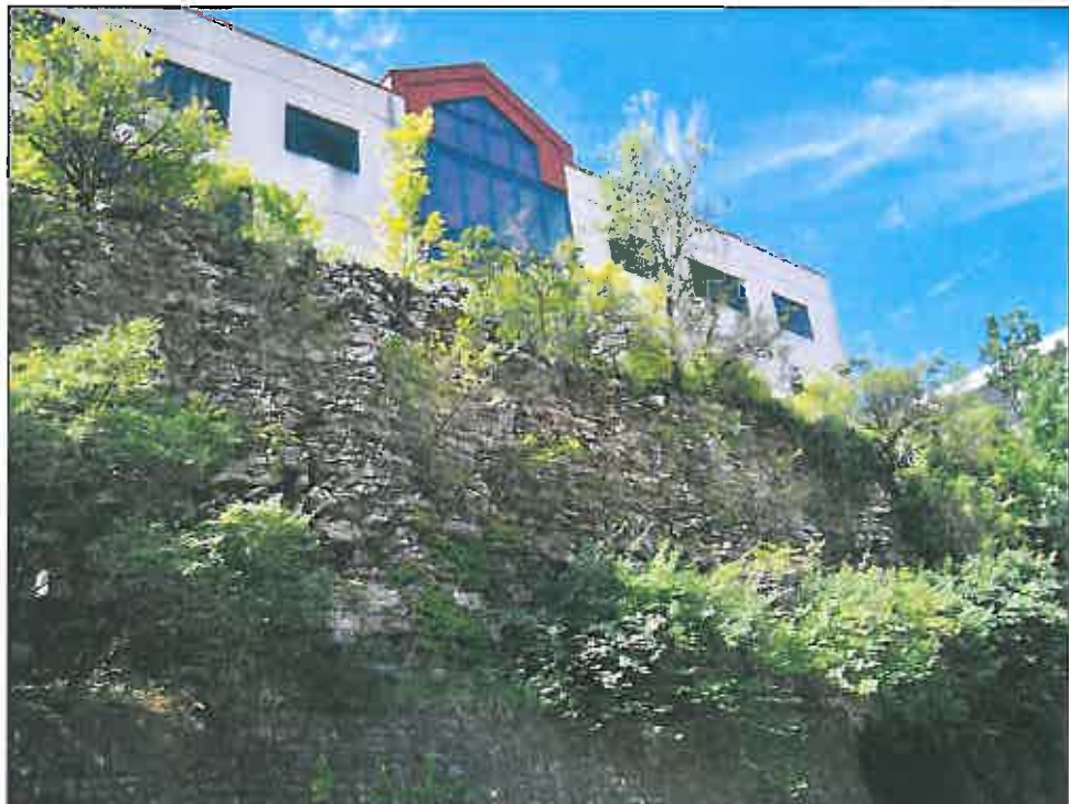
1501 Wyandotte Street – looking south – deterioration of rock/stone armor and wall; overgrown vegetation
