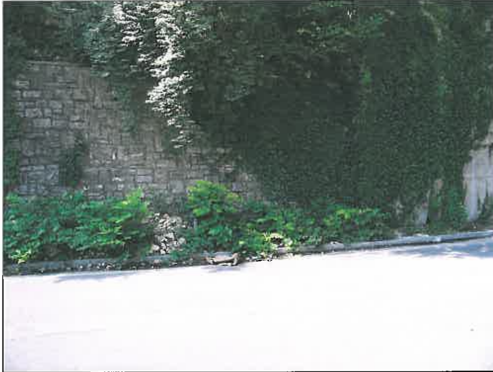
1501 Wyandotte Street – looking south – overgrown vegetation; falling rock
