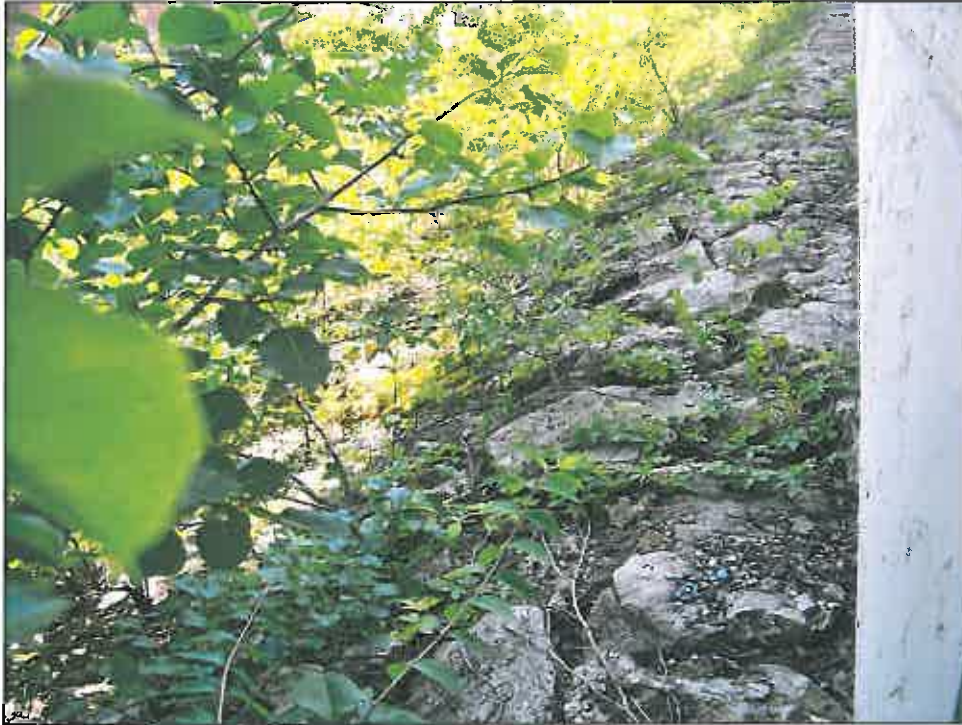
1501 Wyandotte Street – looking east – deterioration of rock/stone armour; overgrown vegetation
