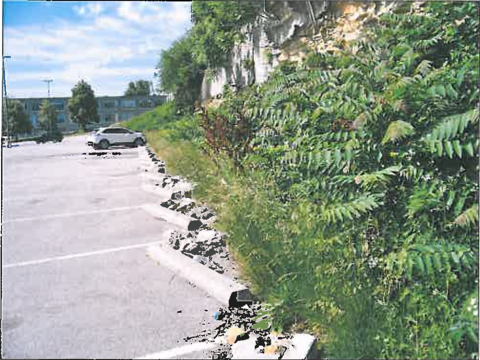
1514 Baltimore Avenue – looking south – overgrown vegetation; trash/debris; deterioration of surface parking lot; falling rock
