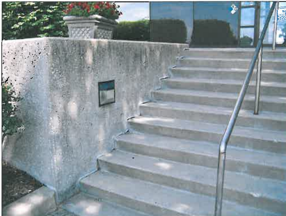
1501 Wyandotte Street – looking northwest – failure of joints/sealants
