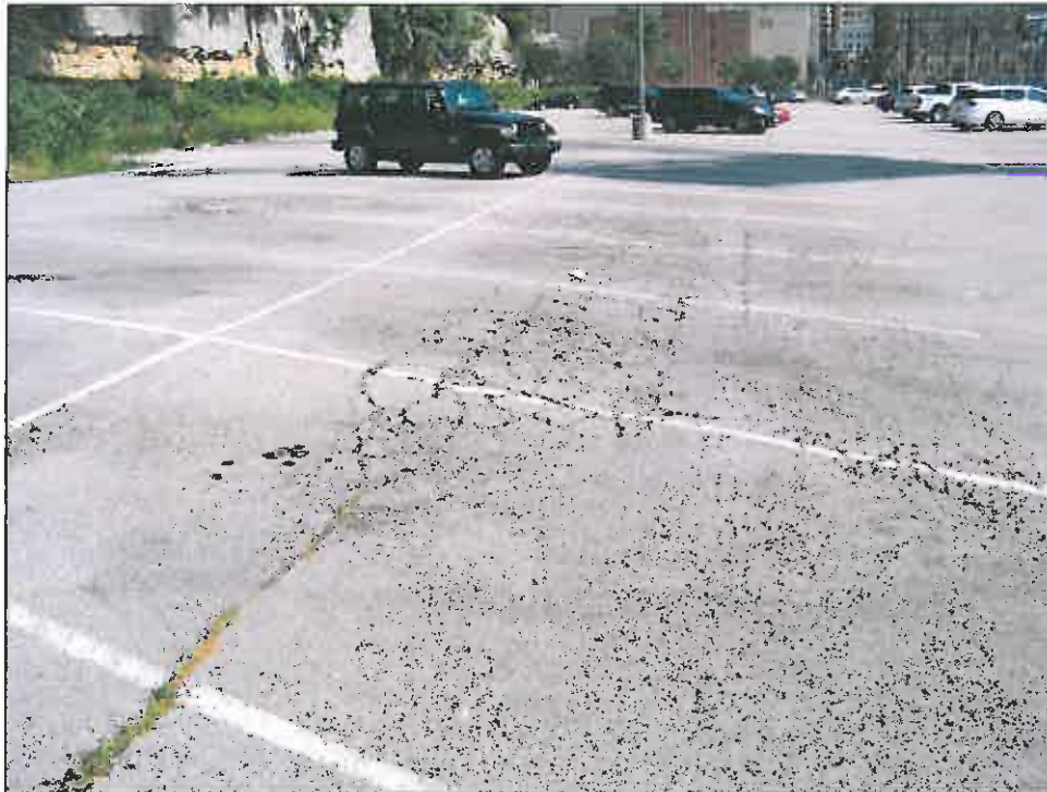
1514 Baltimore Avenue – looking north – deterioration of surface parking lot
