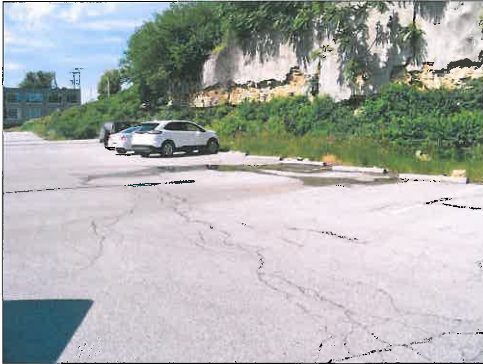
1514 Baltimore Avenue – looking southwest – deterioration of surface parking lot; overgrown vegetation; deterioration of gunite and rock wall
