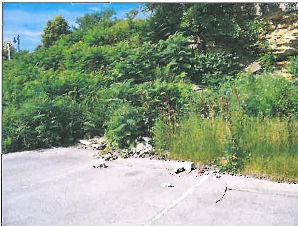
1514 Baltimore Avenue – looking southwest – falling rock; overgrown vegetation
