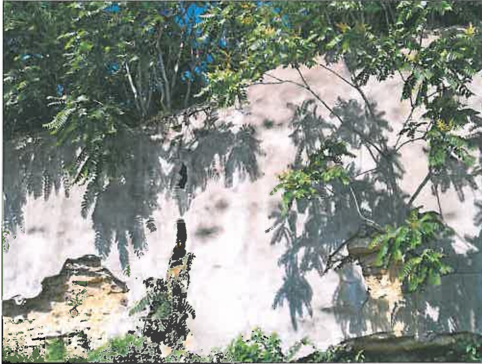
1514 Baltimore Avenue – looking west – deterioration of gunite, rock wall; overgrown vegetation
