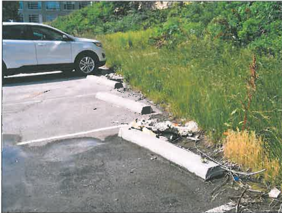
1514 Baltimore Avenue – looking southwest – falling rock; overgrown vegetation; deterioration of surface parking lot
