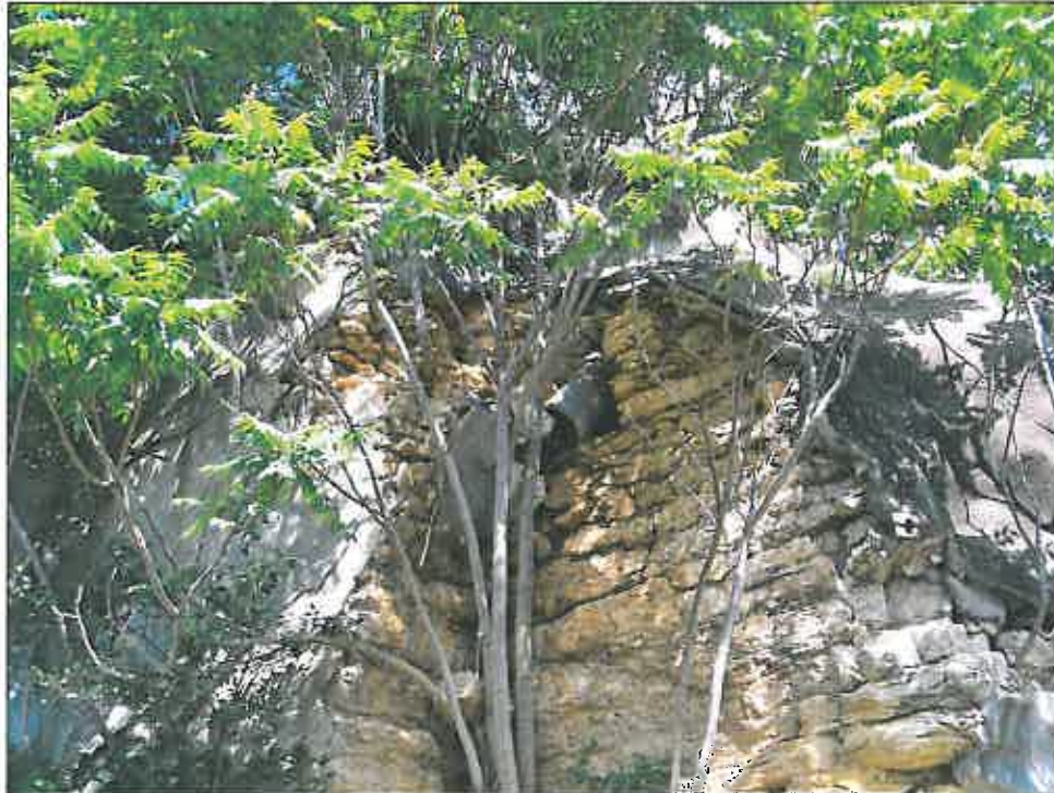
1514 Baltimore Avenue – looking west – deterioration of rock wall and gunite; overgrown vegetation; deterioration of steel ties
