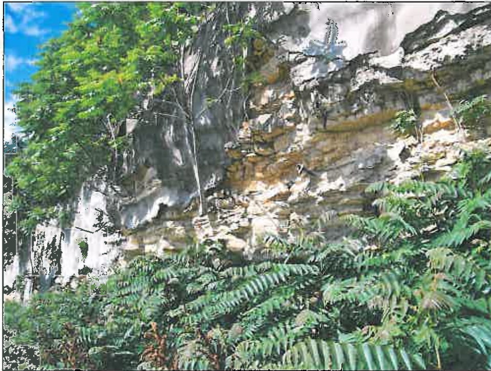
1514 Baltimore Avenue – looking west – deterioration of steel ties; deterioration of gunite and rock wall; overgrown vegetation
