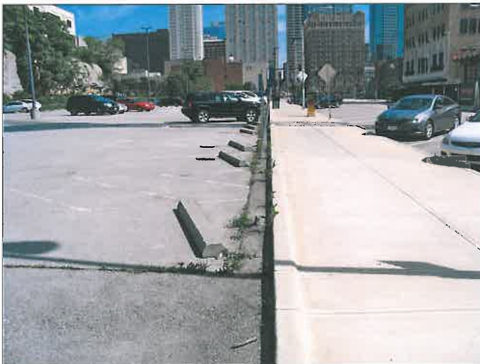
1514 Baltimore Avenue – lack of safe access from handicapped stalls to sidewalk
