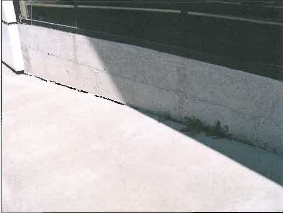
1501 Wyandotte Street – looking north – failure of joints/sealants
