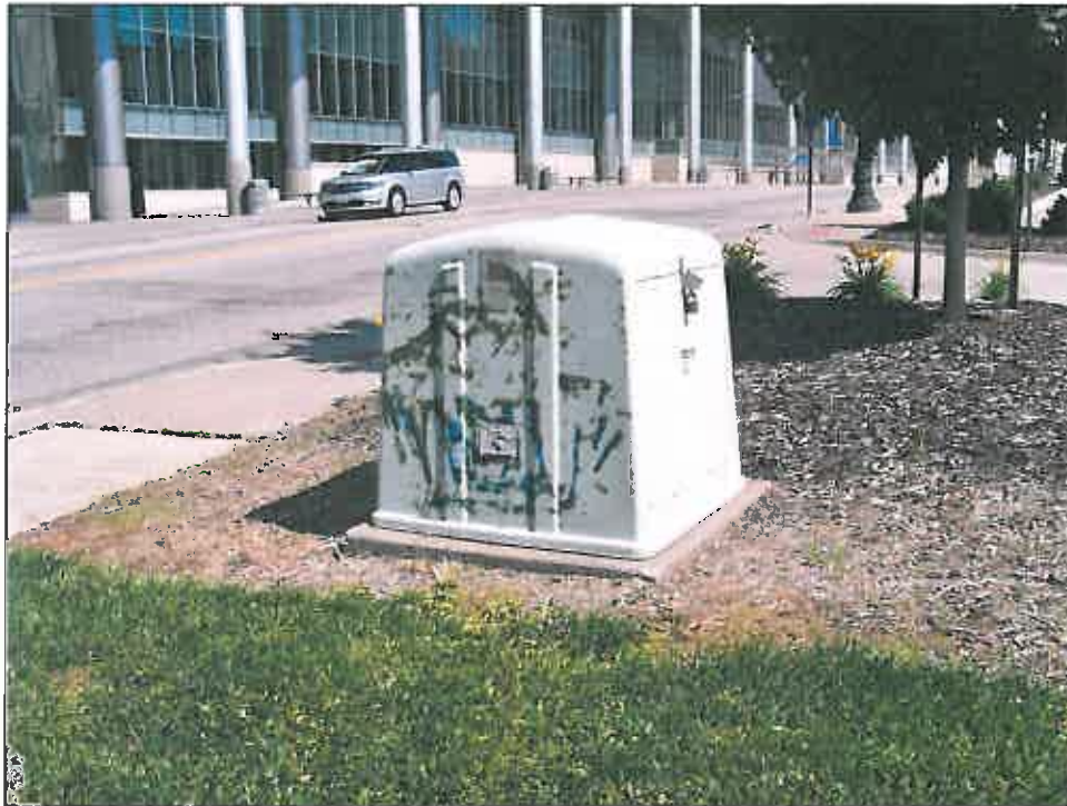
1521 Wyandotte Street – looking northwest – graffiti
