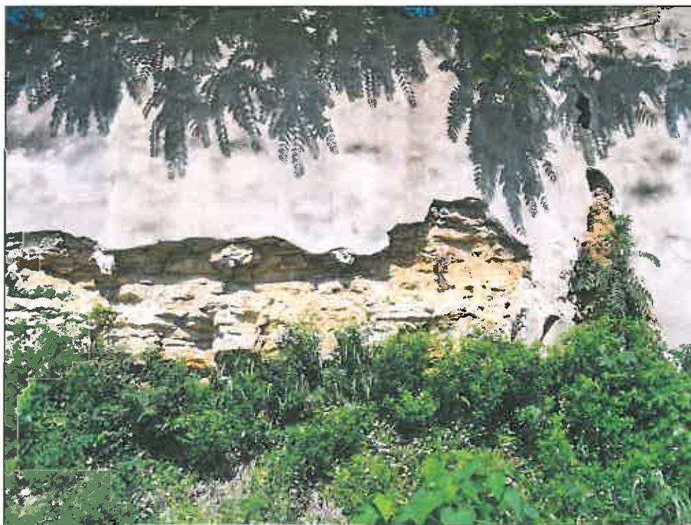
1514 Baltimore Avenue – looking west – deterioration of steel ties; deterioration of gunite and rock wall; overgrown vegetation
