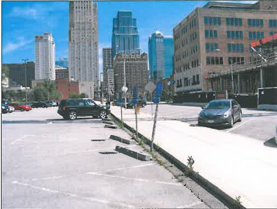
1514 Baltimore Avenue – looking north – lack of curb ramps to sidewalk
