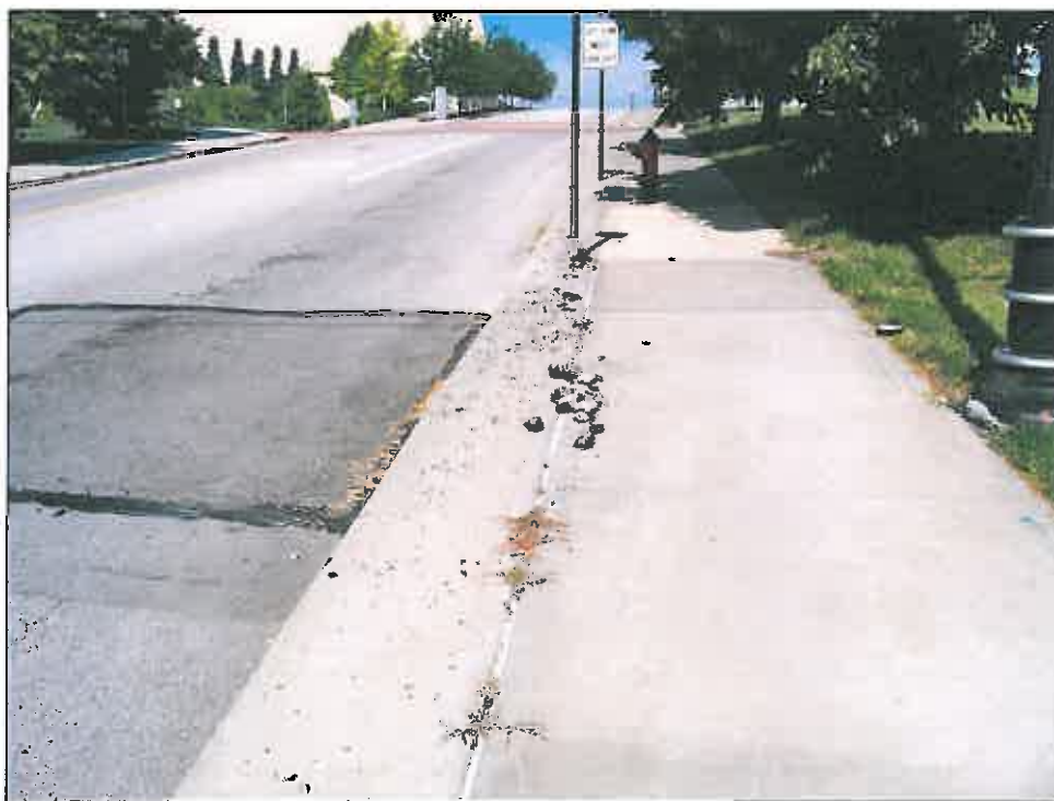
1514 Baltimore Avenue – looking west – trash/debris on sidewalk
