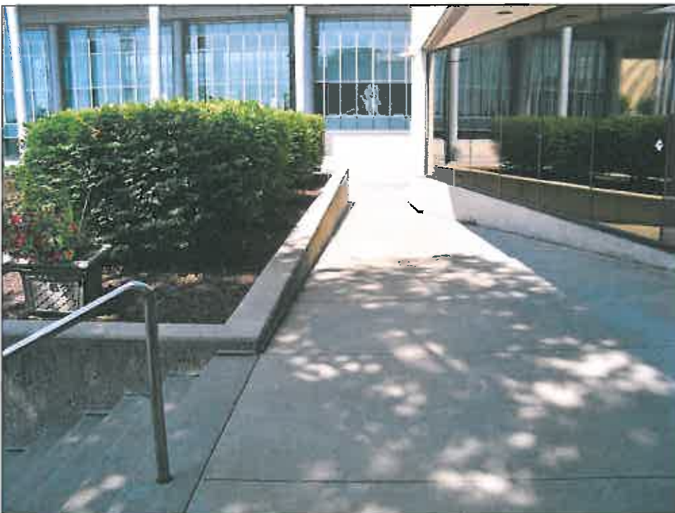
1501 Wyandotte Street – looking west – ramp noncompliant with ADA code
