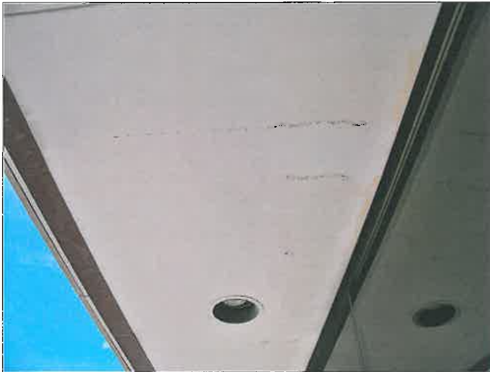
1501 Wyandotte Street – looking west -- failure of finishes on soffit at building entrance
