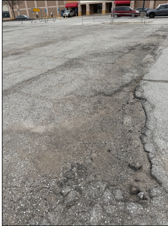
Figure 1: Dilapidated and Deteriorating Paved Parking Areas and Internal Drives
