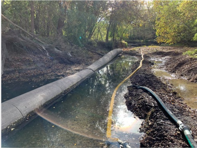
Site 42- Dyke Branch at Holmes Road / $1,500,000 estimated cost / temporary emergency repair already completed
