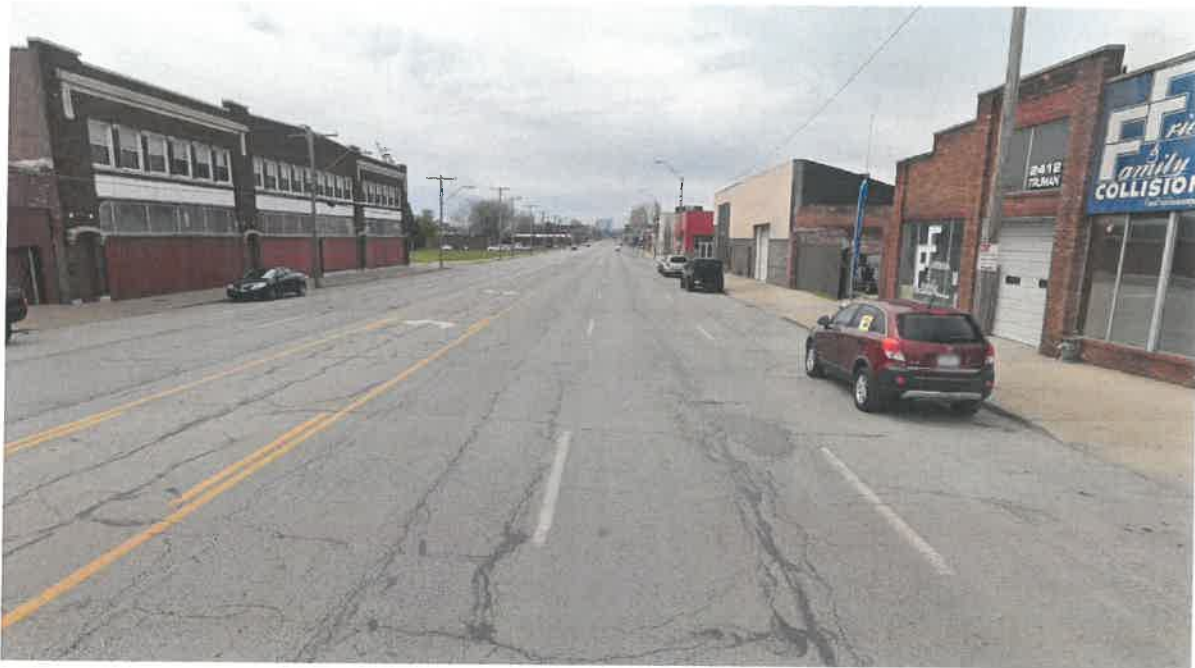
Figure 75: Needlessly Wide Roads like Truman Road Contribute to Elevated Risk of Fatal and Serious Injury Crashes (Image Source: Google)
