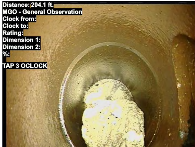
SHEET 25 S087-154 IS NOT A MANHOLE LISTED AS O/C POINT REPAIR BASE BID
