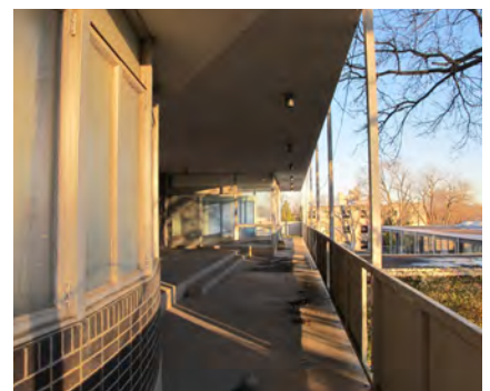
Top to bottom: 1) Cafeteria/Parish Hall, 2) Gymnasium 3) Typical classroom, 4) Balcony on second floor (Photographs of St. Francis Xavier School taken December 2012)
